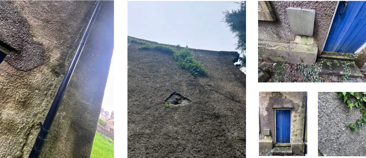
Fig: 3 Examples of deteriorating current cementitious render in extremely poor condition. Evidence of vegetation growing through the render in places along with substantial surface cracks.
