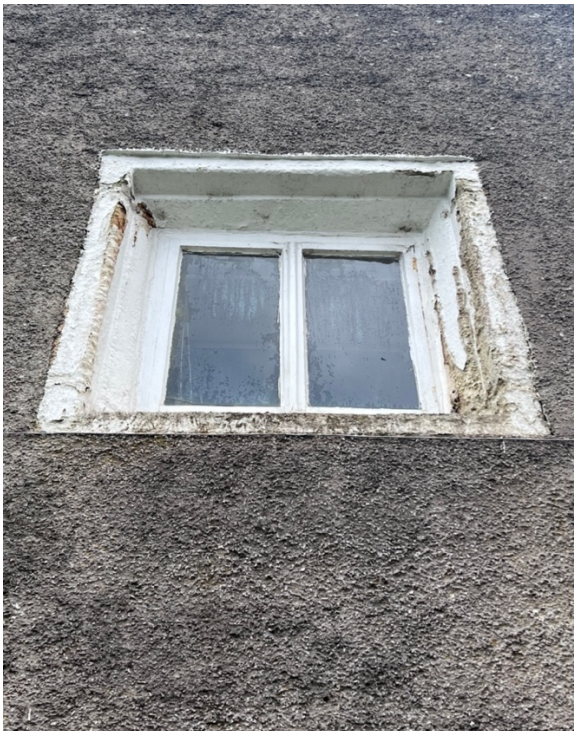
Fig: 5 Example of existing stone surround in extremely poor condition to be replaced with new natural stone to match profile/size
