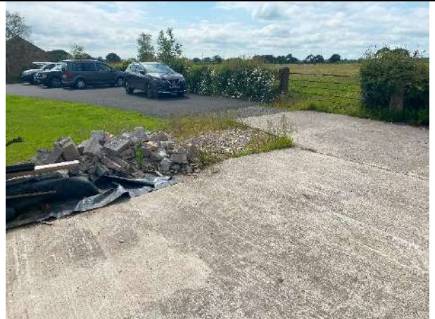
P2: View of where the access road meets the hardstanding of the barn area in the north of the site
