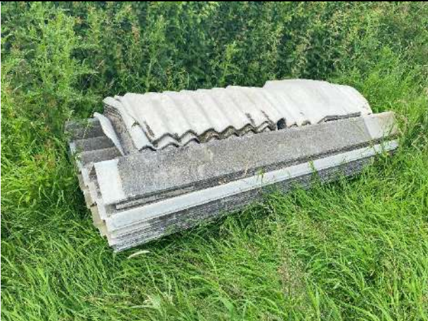
P11: Roof sheeting material used in the construction of the barn building proven to be devoid of asbestos through laboratory testing
