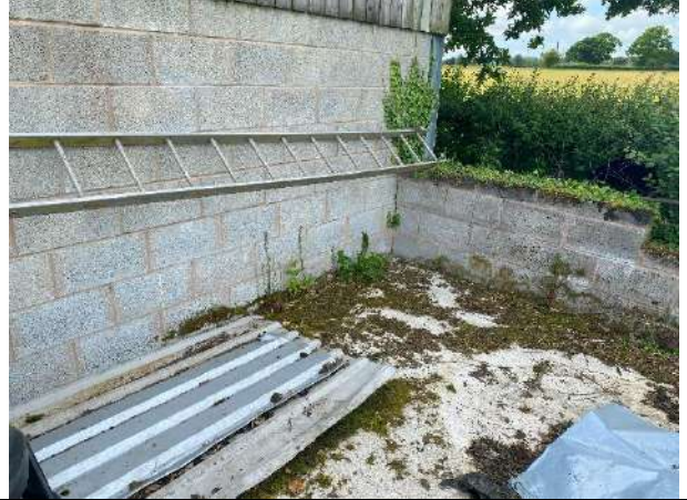
P10: Miscellaneous items to the rear/gable end of the barn building
