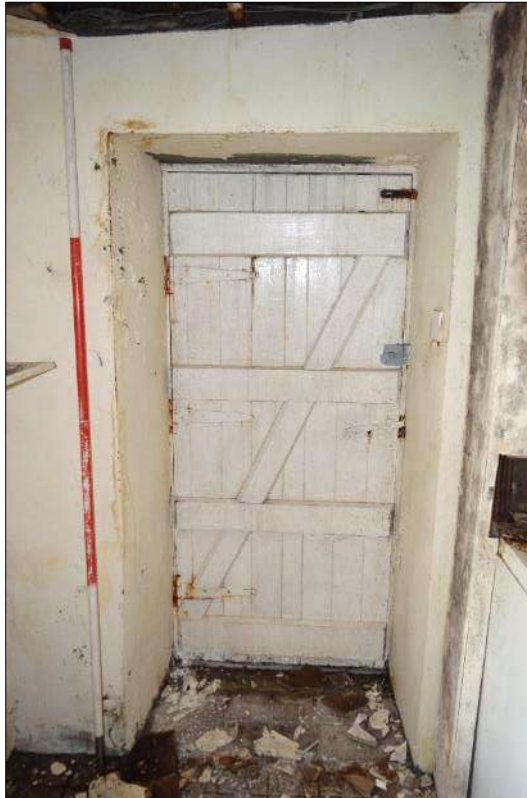
Plate 32 (shot 175): Plank and batten door with later brace, looking east-northeast, 2m scale
