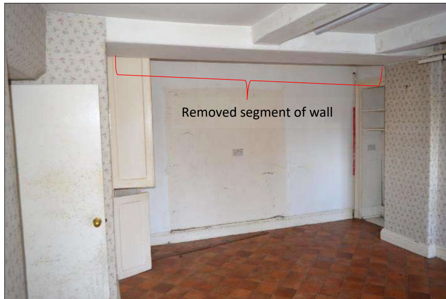
Plate 18 (shot 142): Segment of wall removed between pantry and extant kitchen (1.1), looking southwest, 2m scale
