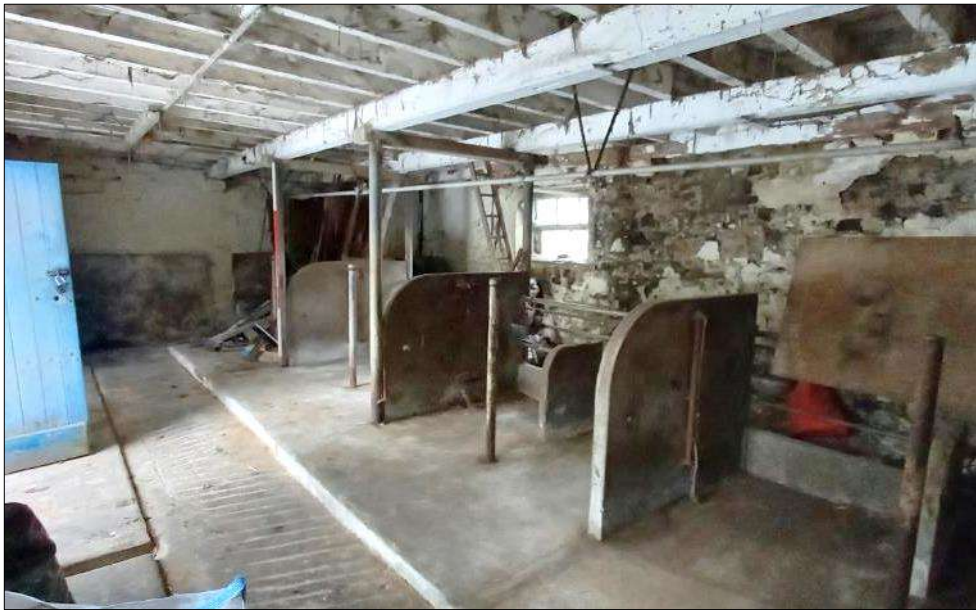
Plate 75 (shot 10): View of ground floor in the byre, looking south, 2m scale
