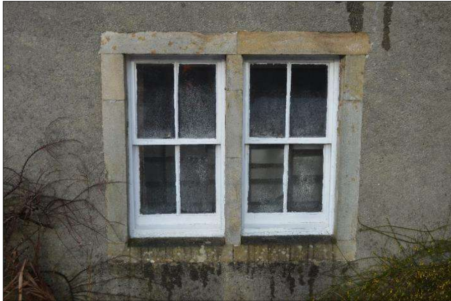
Plate 11 (shot 119): Close up of ground floor, recessed, sash window with glazing bars and no horn, looking north-northwest
