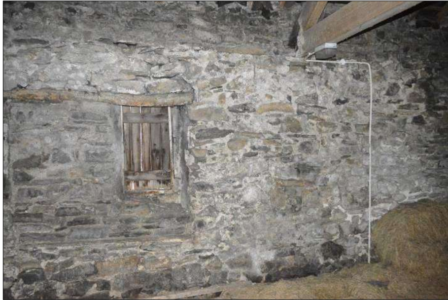
Plate 82 (shot 29): Modified and reduced window/pitching hole, notice the horizontal line in the stonework on truss level, looking southwest, 2m scale
