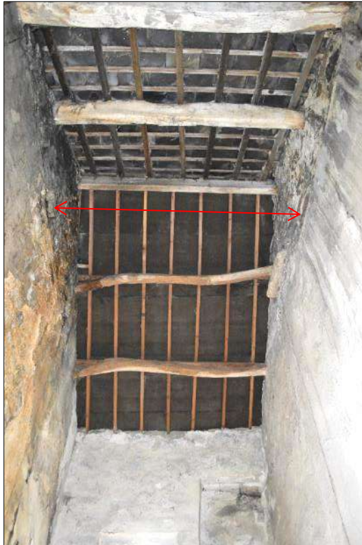
Plate 52 (shot 128): Purlin roof structure and niche or blocked opening on the southeast wall, first floor level, notice the lack of thick plaster on the gables, see arrow, looking southeast
