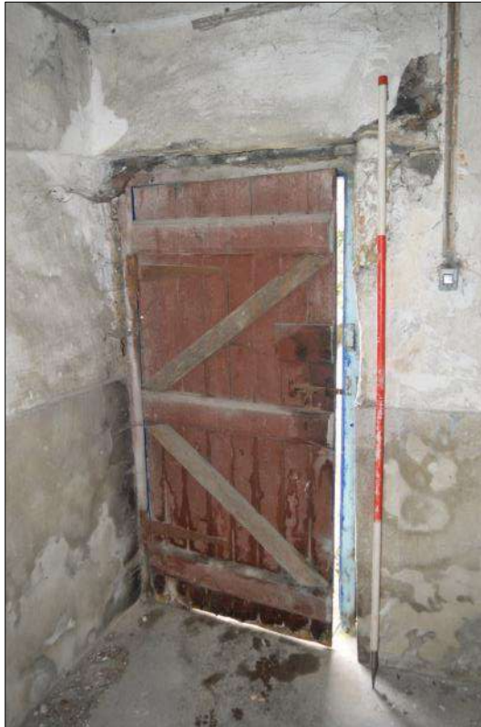
Plate 57 (shot 133): Close up of southwest plank and batten door, looking southwest, 2m scale
