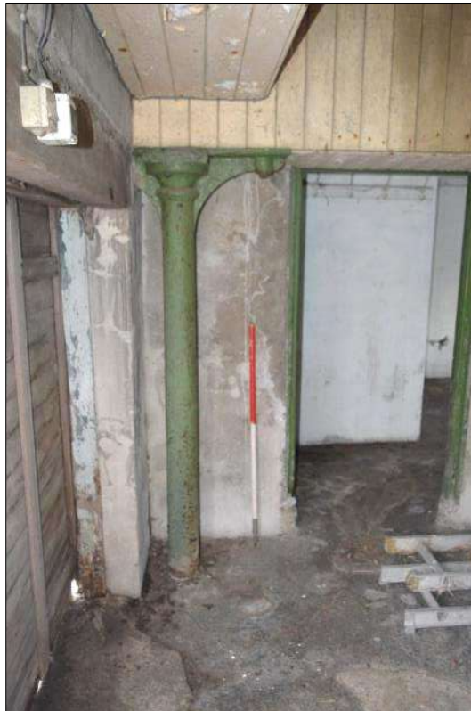
Plate 89 (shot 38): Close up of cast iron column along the northeast wall, looking southeast, 1m scale
