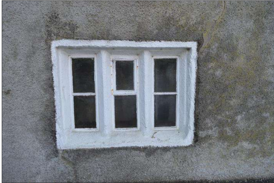
Plate 3 (shot 95): Small ground floor, mullioned window on the northwest elevation, looking south
