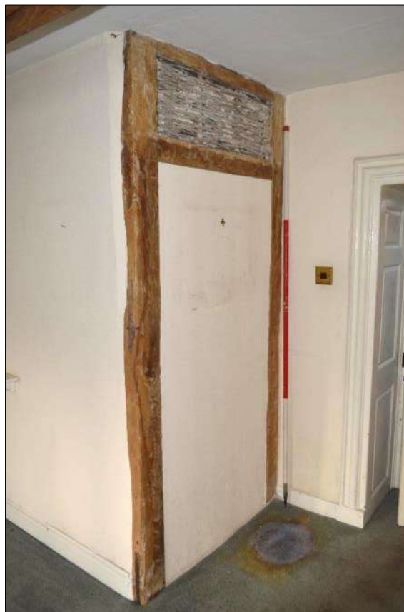
Plate 21 (shot 165): Blocked doorway to pantry with wattled panel above, looking west-northwest, 1m scale
