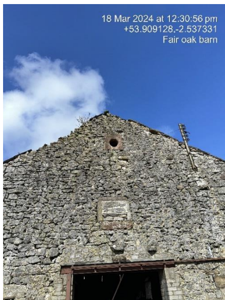
Photo 3: Gable end of barn, south side. Missing roof tiles, gaps in stonework throughout, unsealed entrance and unsealed circular window.
