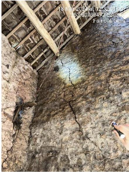
Photo 9: Crevices present on the internal wall.
