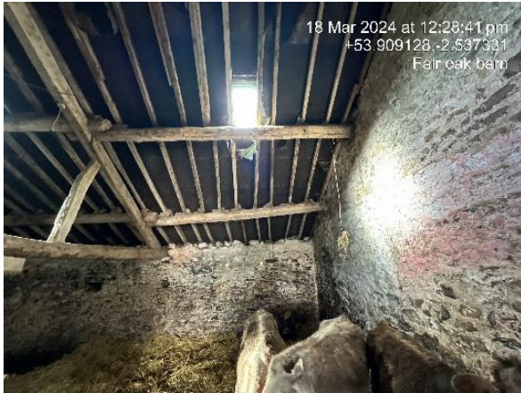
Photo 13: Unsealed roof membrane in side room.
