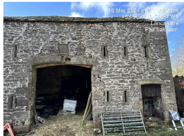
Photo 2: Eastern aspect of the barn. Gaps in missing/cracked mortar, most noticeably around entrance, providing bat roost opportunity. Entrance and windows lack closures.
