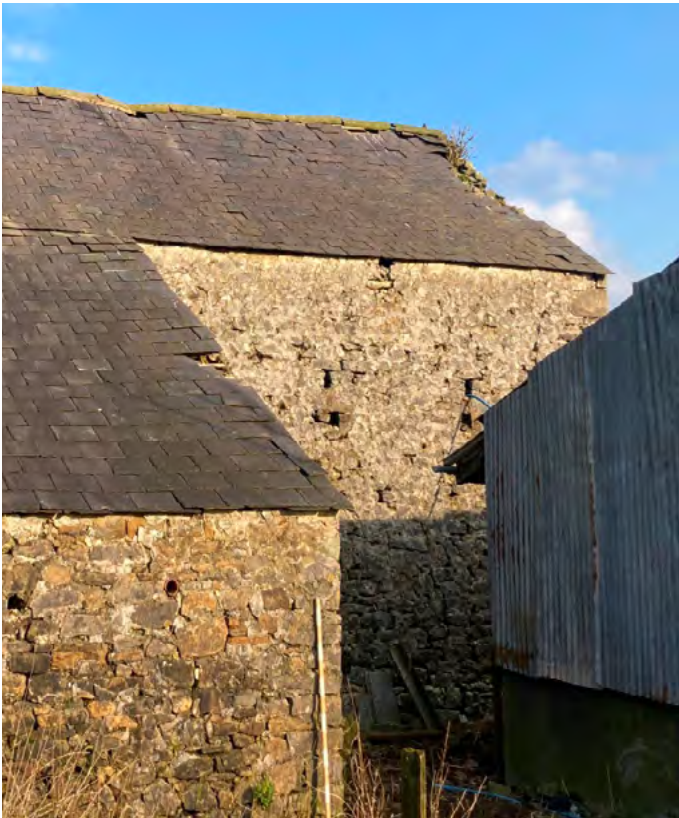
South end of oushut and main barn showing slipped and missing slates at verge and ridge including plant growing out of the wall top to main barn. Also note hairline cracking at high level to both walls.
