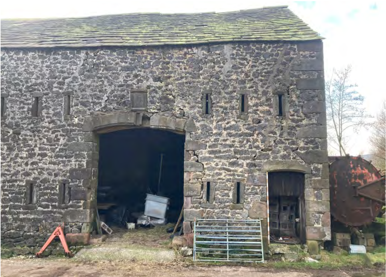
North end of east elevation showing vent slits to both floors and threshing doorway with lost voussoir to arched lintel and diagonal crack across the corner. Also note previously repointed cracking to high level.
