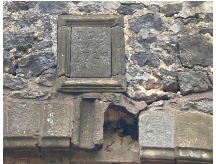
Missing stone voussoir to arched lintel and date stone above.
