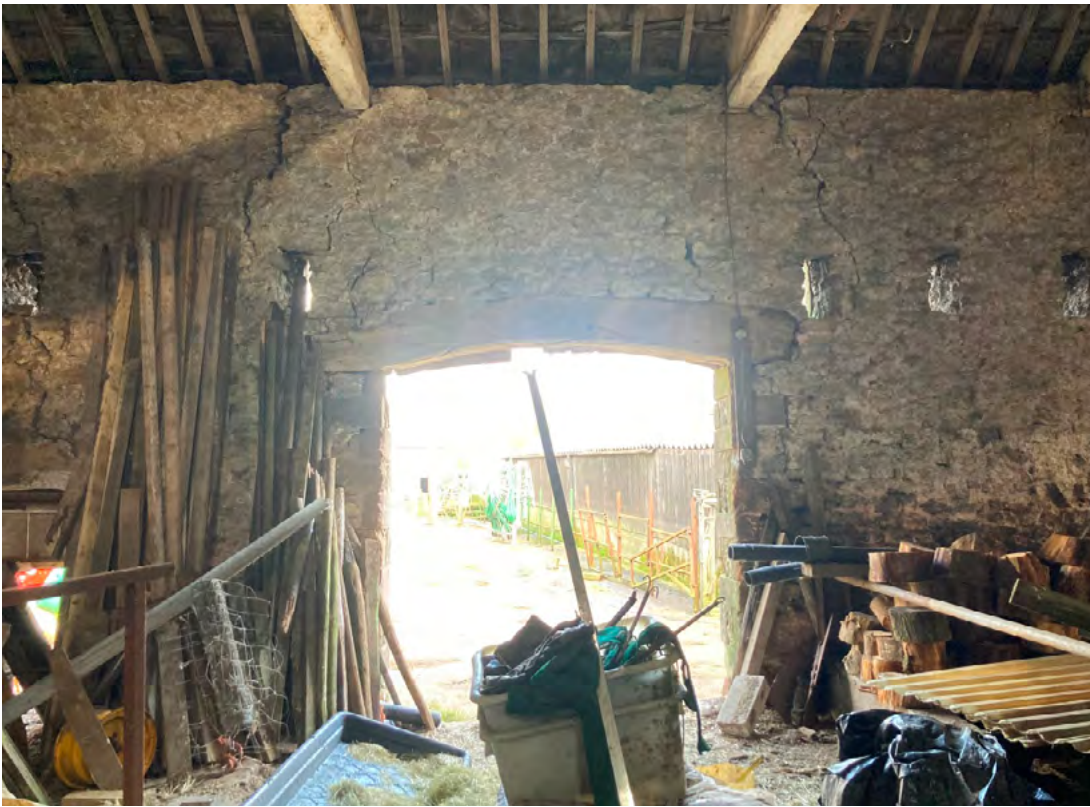
North end of east wall to main barn internally. Showing cracking from wall head to either side of the doorway.
