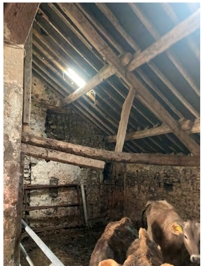
Outshut looking to southwest corner showing failed and partially supported half truss. Also note blocked openings to south wall beyond.
