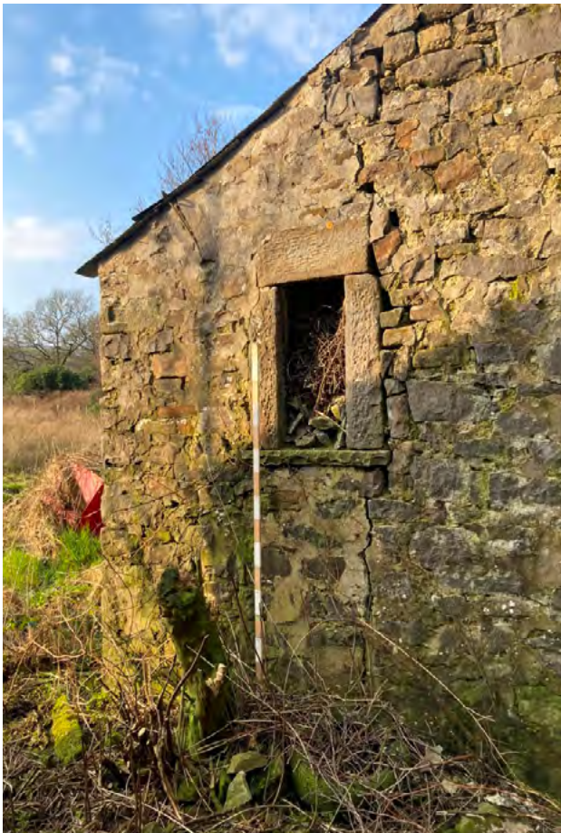
Southwest corner of outshut showing crack to the right of partially blocked window on south return wall.
