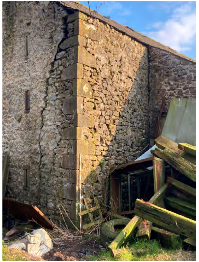
View of northwest corner of main barn and abutment with north return to oushut showing cracking to main barn and at unbonded abutment with oushut.
