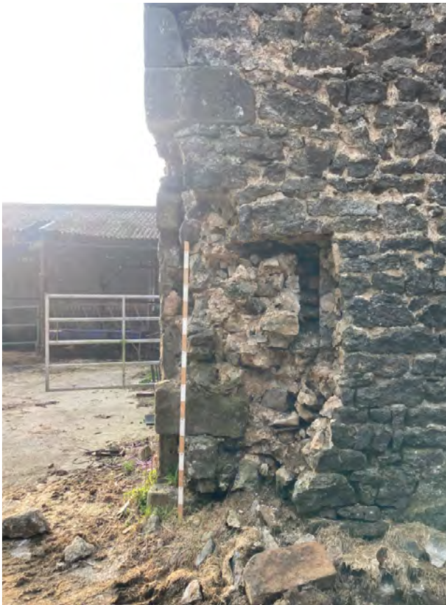
Lost masonry to southeast corner of the barn, viewed from the east side
