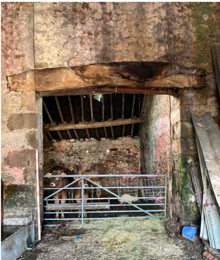
Arched timber lintel to doorway in west wall opposite threshing doorway through into outshut. Note hairline cracking the masonry above,
