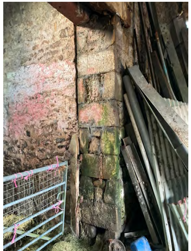
North side of doorway into outshut showing crack at abutment of main barn and outshut and fixing at head for lost doors.
