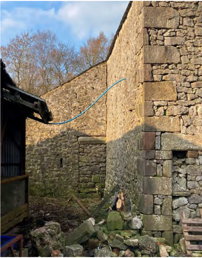
View of south west corner of main barn and south return of oushut. Note crack to unbonded masonry at abutment.
