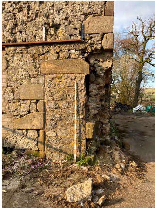
Lost masonry to southeast corner of the barn, viewed from the south side. Also not previously blocked doorway to shippon.
