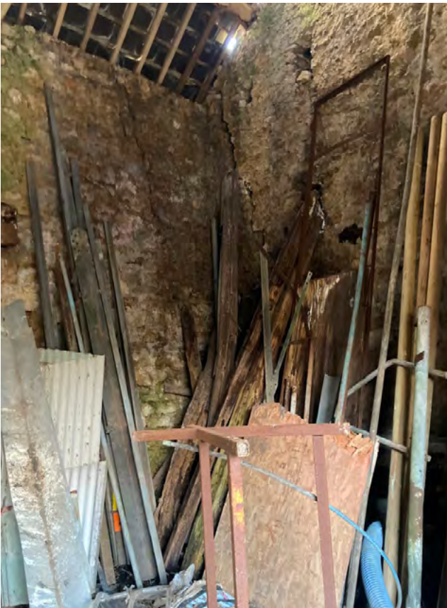
Cracking to northwest corner of main barn hidden behind stored items.
