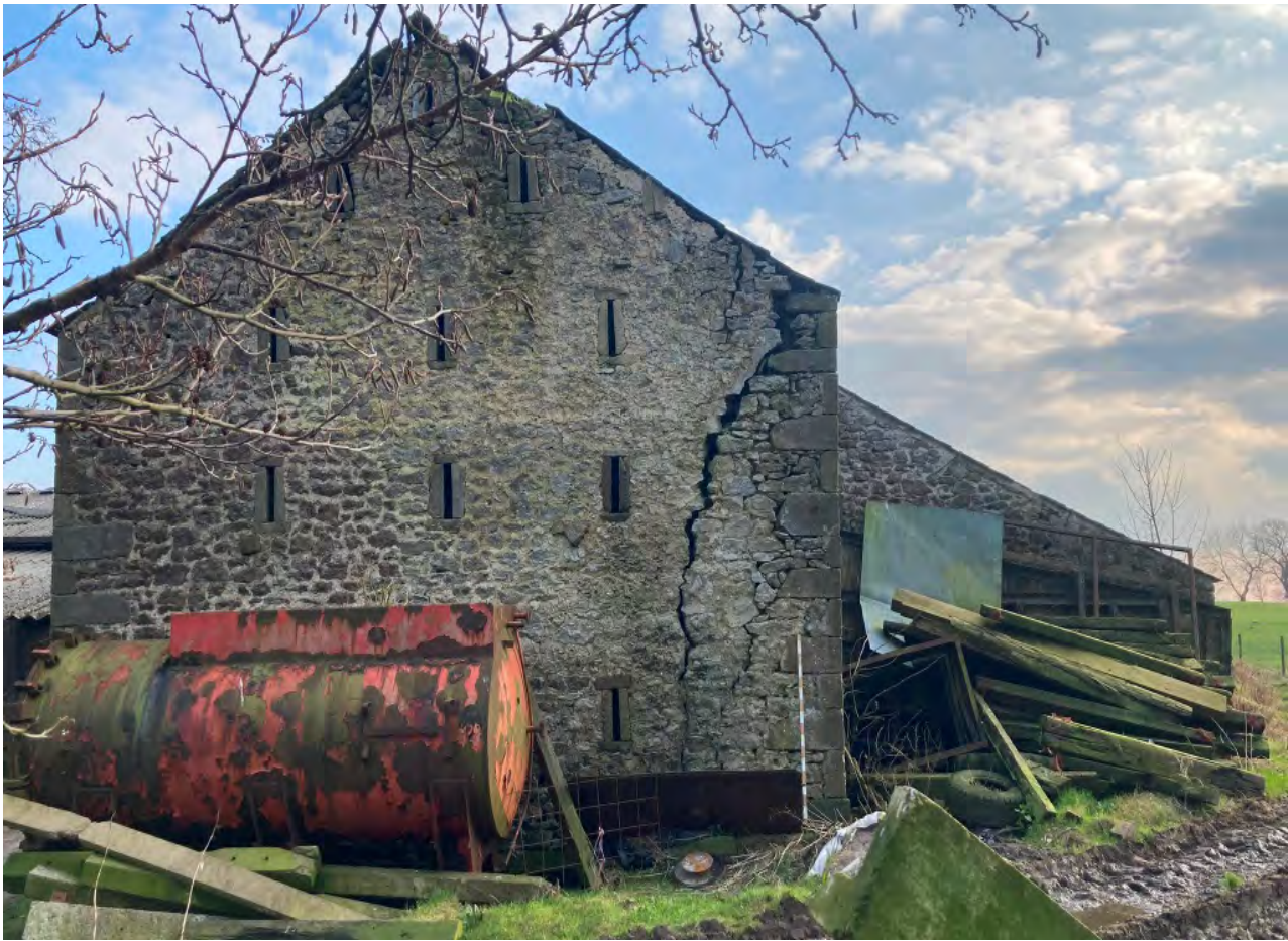
North gable of barn showing tear crack to east corner washed out walltops to main barn.
