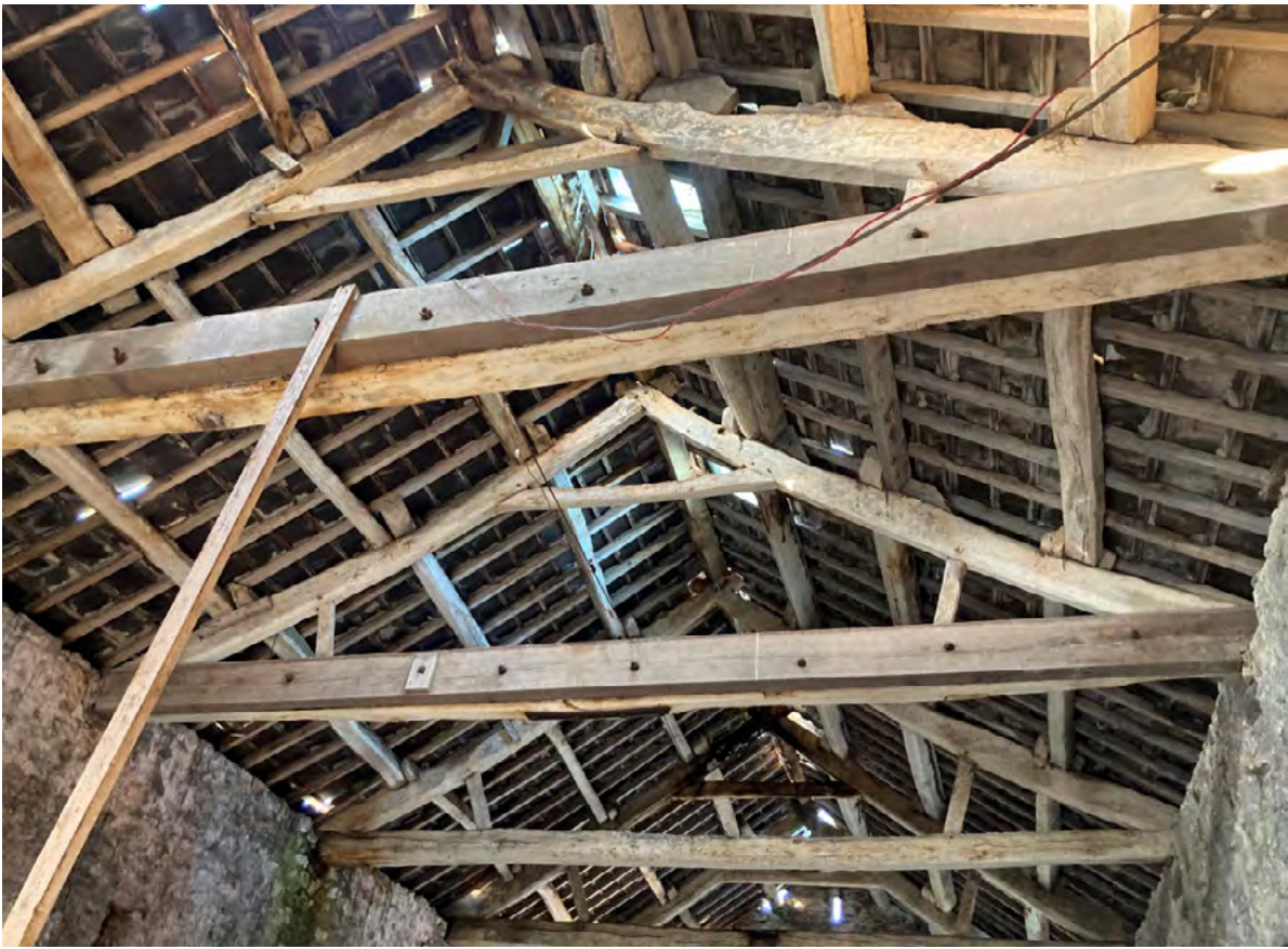
View of roof structure looking north, showing additional support to ties of end two trusses and decay from water ingress to head of truss beyond.
