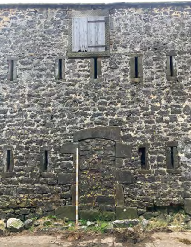
South end of east elevation showing blocked doorway and pitching window above. Also note missing masonry and washed out pointing at ground level.
