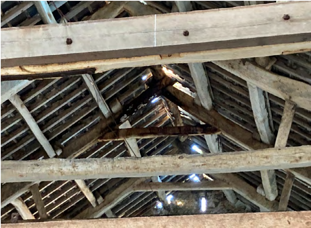
Viewed of decayed head to truss as a result of loss of ridge stones.
