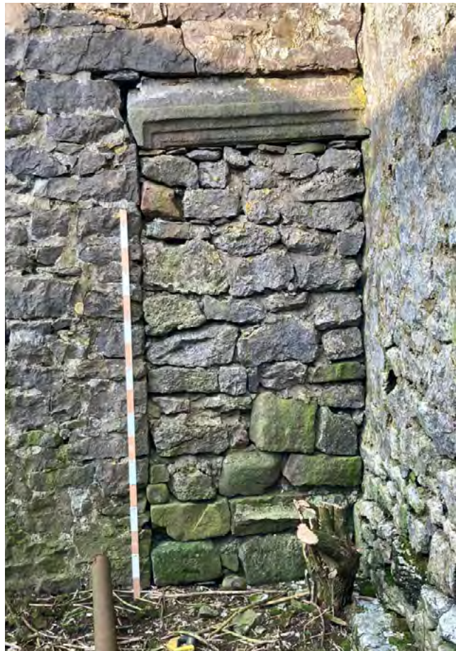
East return wall of oushut at abutment with the west wall of the main barn, showing crack at abutment and blocked doorway with reused lintel to head.
