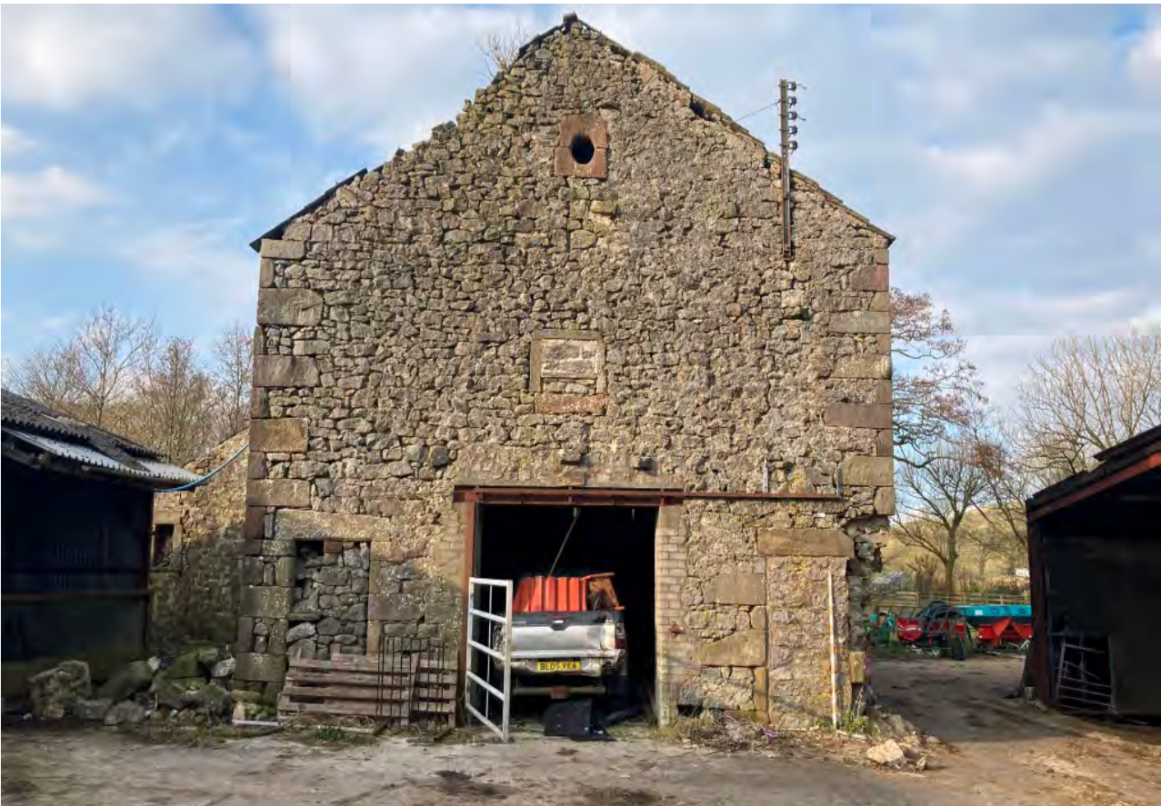
South gable of barn showing more recent central doorway, with blockwork jambs. Also note blocked pitching window above and blocked shippon doorways either side, lost southeast corner and washed out walltops.
