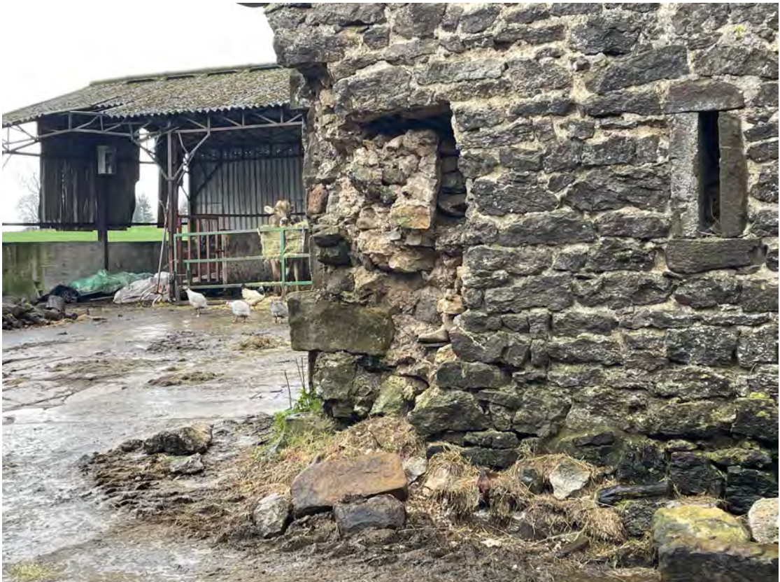
Photo 8: Collapsed South-East Corner
