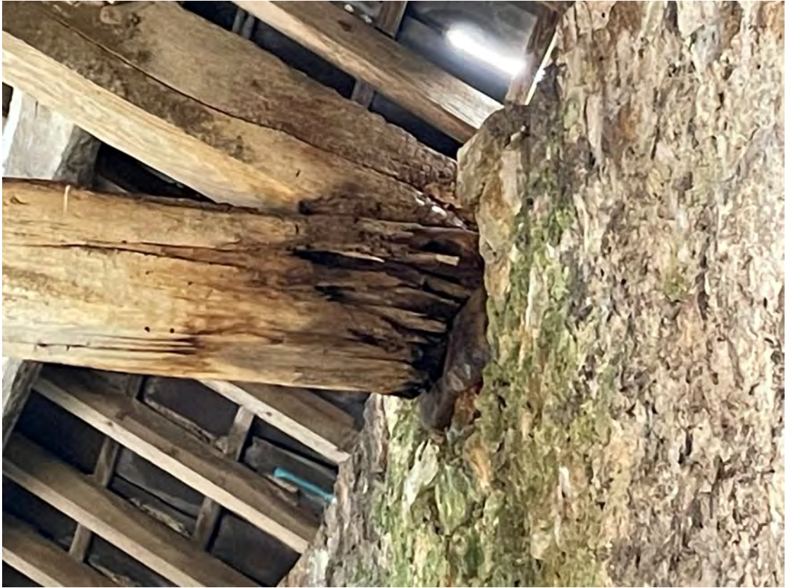
Photo 5: Central Truss End Failure
