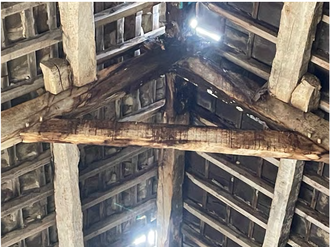
Photo 6: Truss No. 4 - Apex Timber Rot
