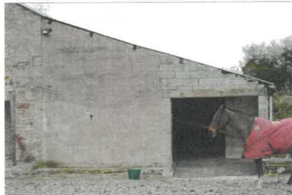
Blockwork rear extension to be removed – enhancing and exposing the original character of the barn
