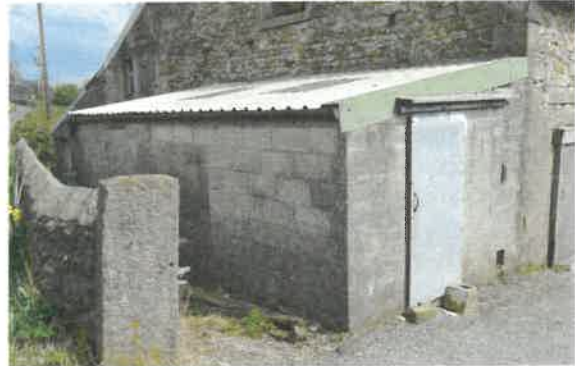
Blockwork extensions to be removed – enhancing and exposing the original character of the barn
