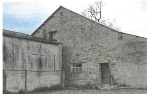
Adjacent dilapidated portal frame and fibre cement / asbestos agricultural building to be removed exposing the original barn and character.
