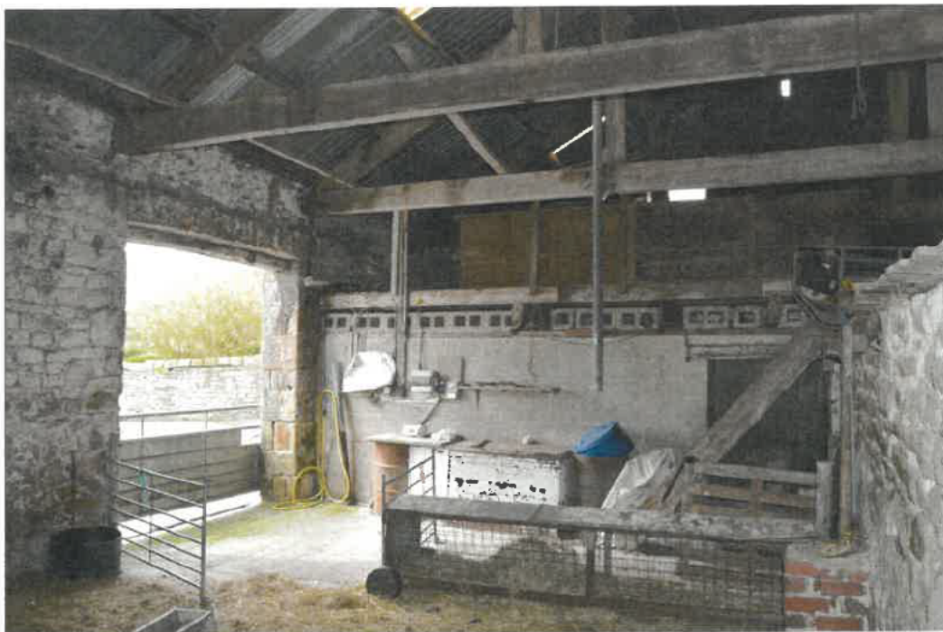
PL10: Photo showing internal roof structure with queen post trusses either side of large barn door opening. Underside of profiled metal sheeting visible over treated rafters.
