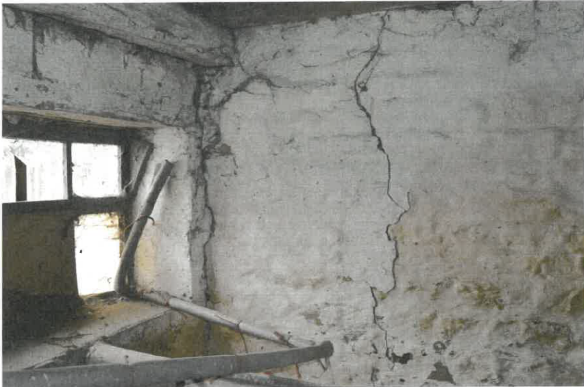
Cracks to be reviewed by Structural Engineer and crack stitch repairs proposed to be carried out.
