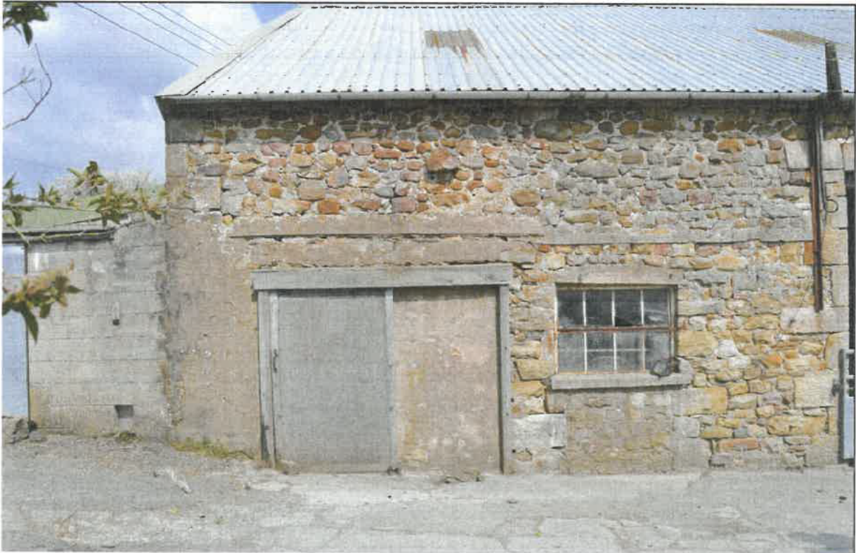
PL08: Photo showing metal roof sheeting to barn on front elevation and grey half round pvcu gutters
