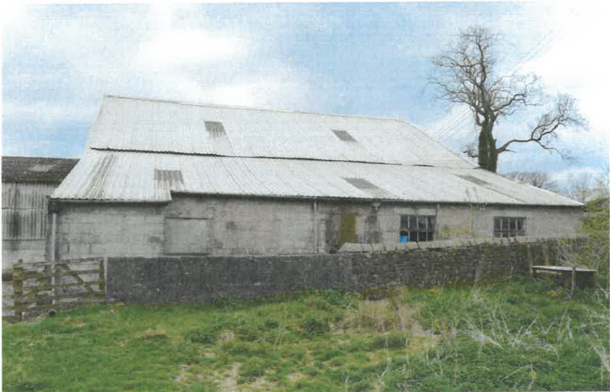
PLO7: Photo showing metal roof sheeting to barn in average to poor condition. The rear blackwork and rendered add on extension is proposed to be removed.
