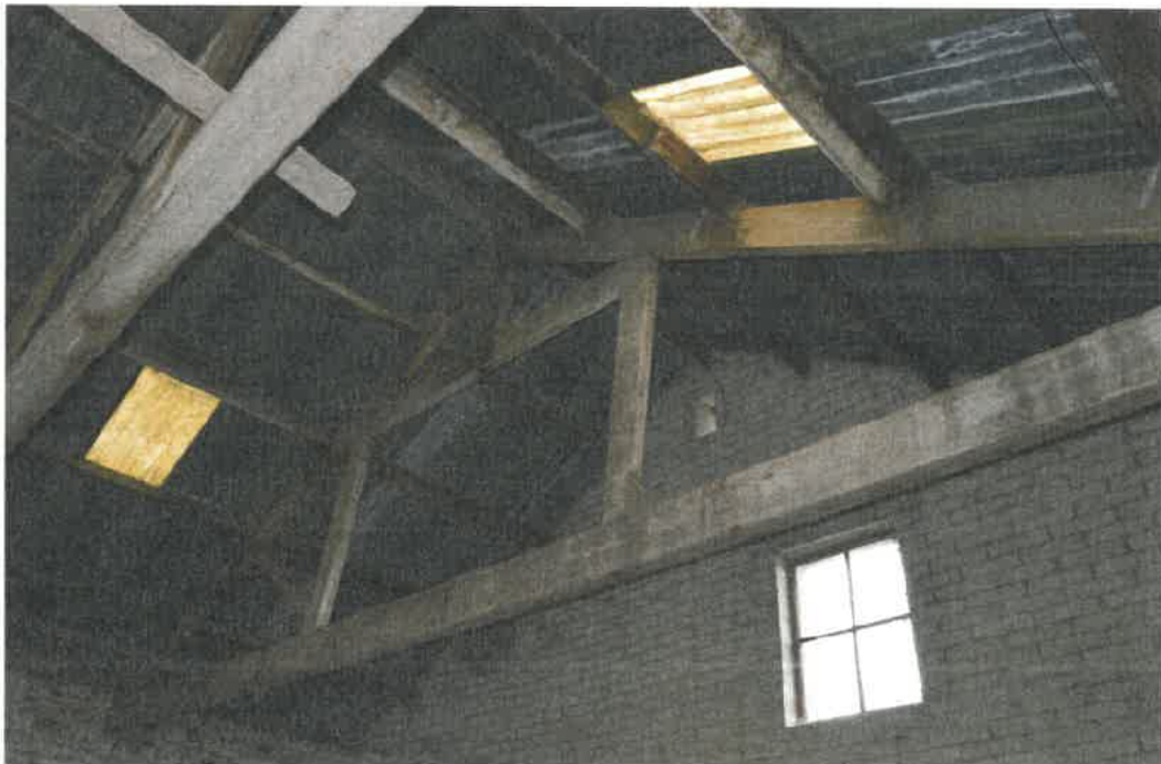
PL09: Photo showing roof structure, comprising of queen post sawn trusses, sawn purlins and rafters.
