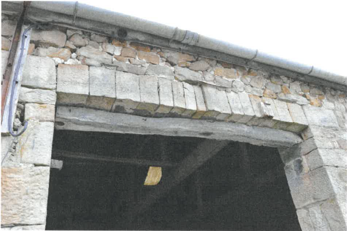
PL06: Internal photo of Vicarage Farm Barn – Large Entry doorway with reclaimed lintel over
