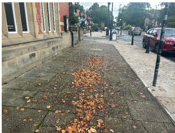
Photo 3: Front of the building. The demarcation between the two different pavement surfaces is where it is proposed to reinstate the wall in front of the building.
