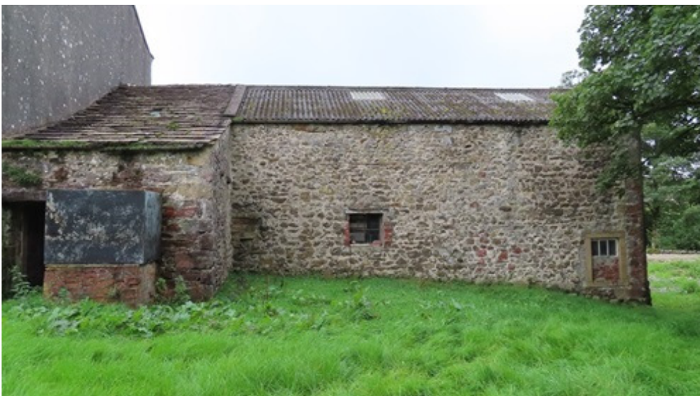
9. The rubblestone construction of the barn; note that the original roof finish is lost and has been replaced with corrugated mineral cement sheets, the original flag roof of the trap house remains
