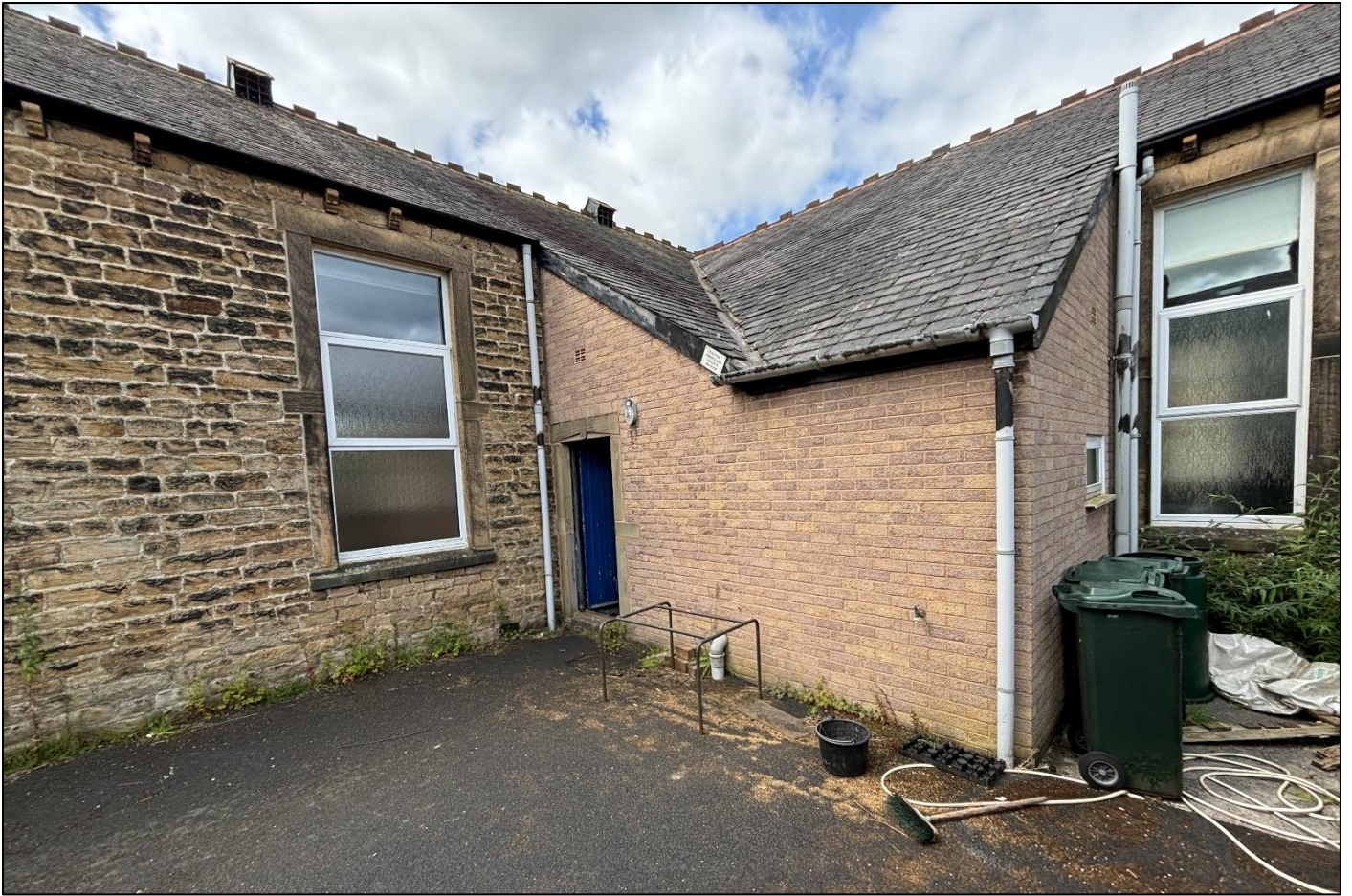
Fig 02: View of the existing toilet block to the rear of the building.
