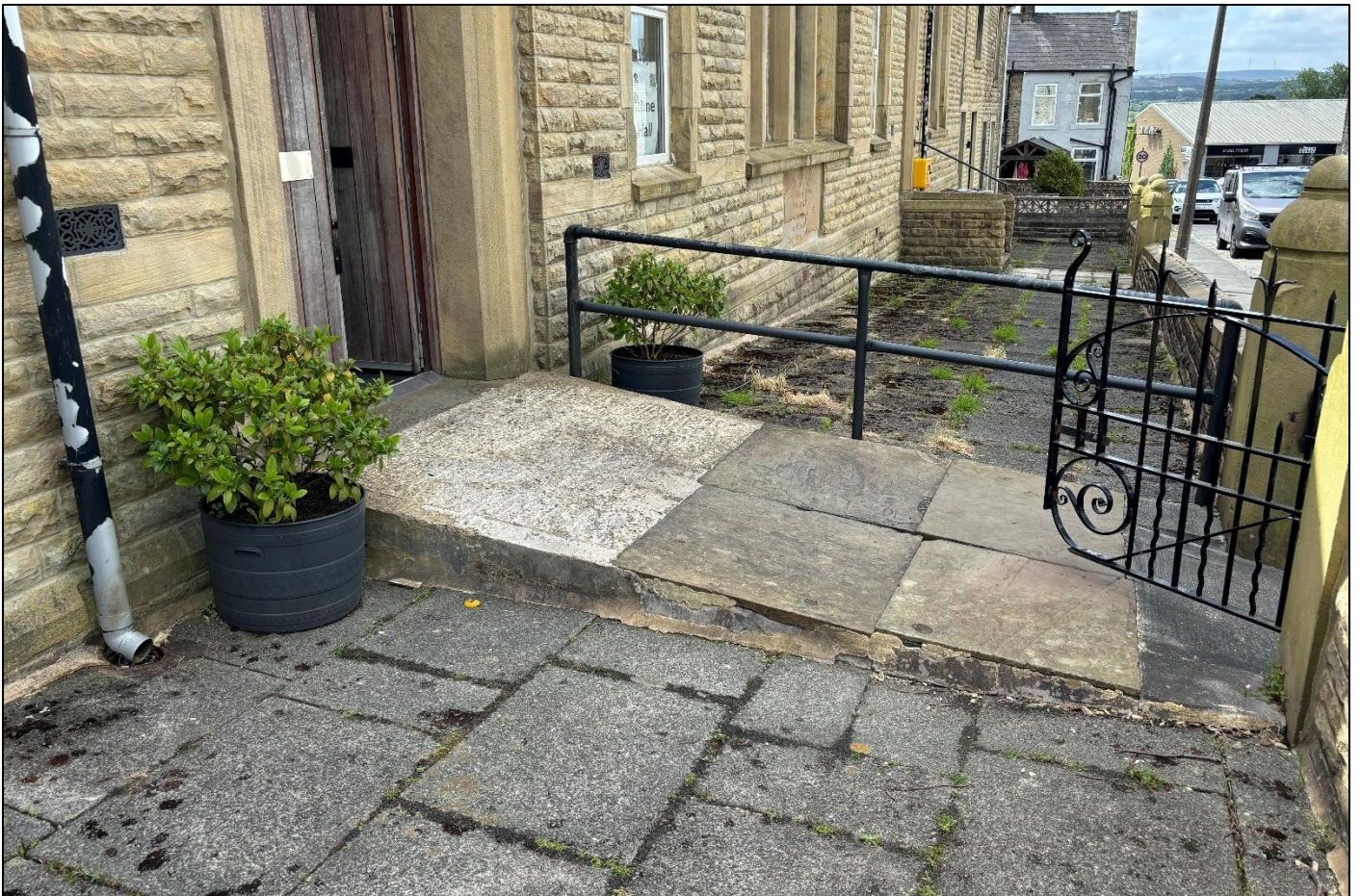
Fig 05: View of the existing ramp access to the north entrance to the building.
