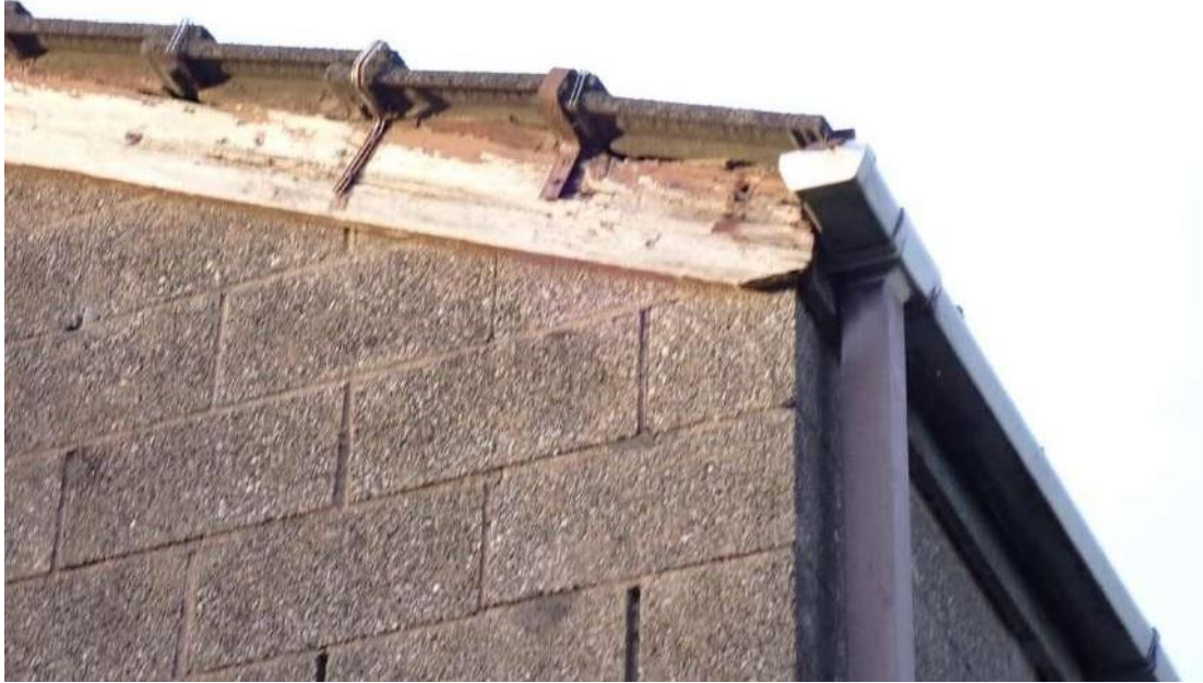
Photograph 5 – View of a damaged section of bargeboard on the western aspect of Building 1.
