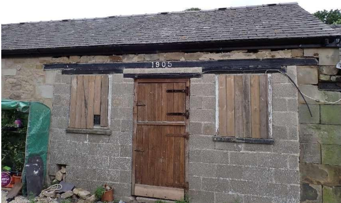
Photograph 18 - View of boarded over windows in on the southern aspect of the eastern section of Building 2.
