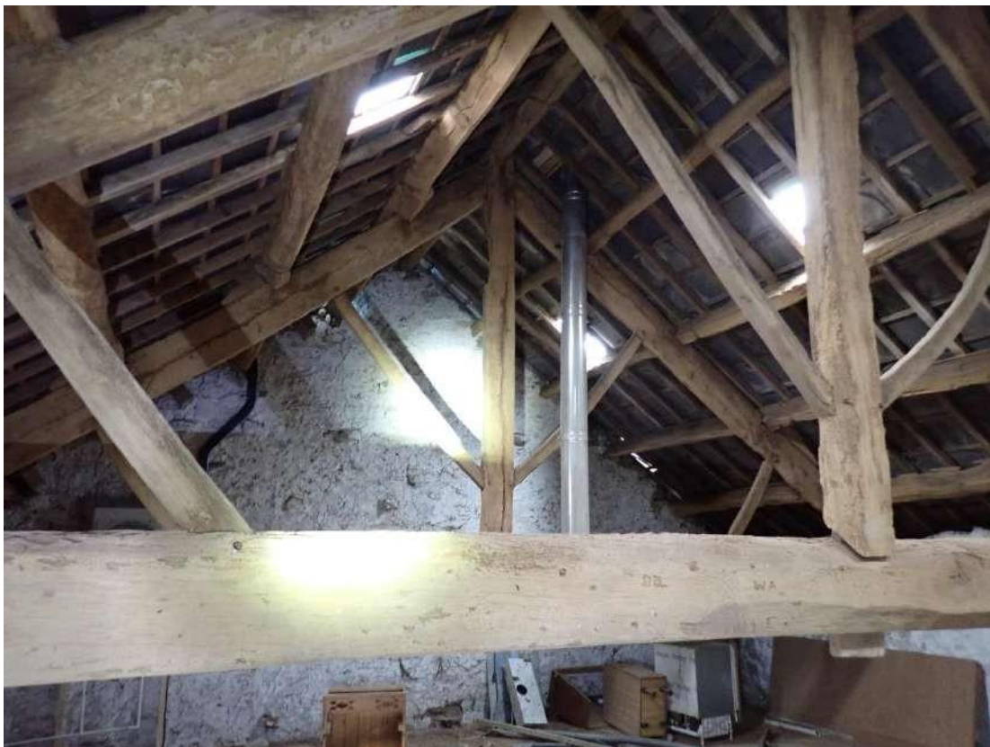
Photograph 62 – View of additional cracks and cavities of the gable end of the barn section of Building 3.
