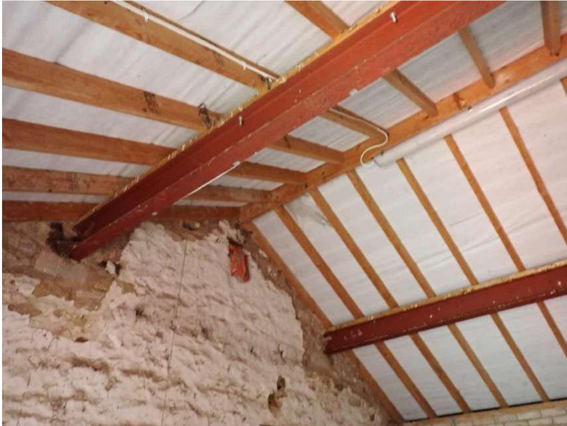
Photograph 39 – View of the underside of the roof in the western room of the pig styes in Building 2, showing the steel rafters and the breathable membrane lining.
