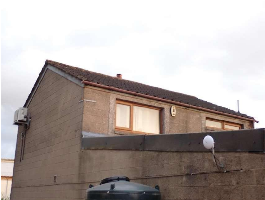
Building 9 – View of the lead flashing where the garage attaches to Building 1.
