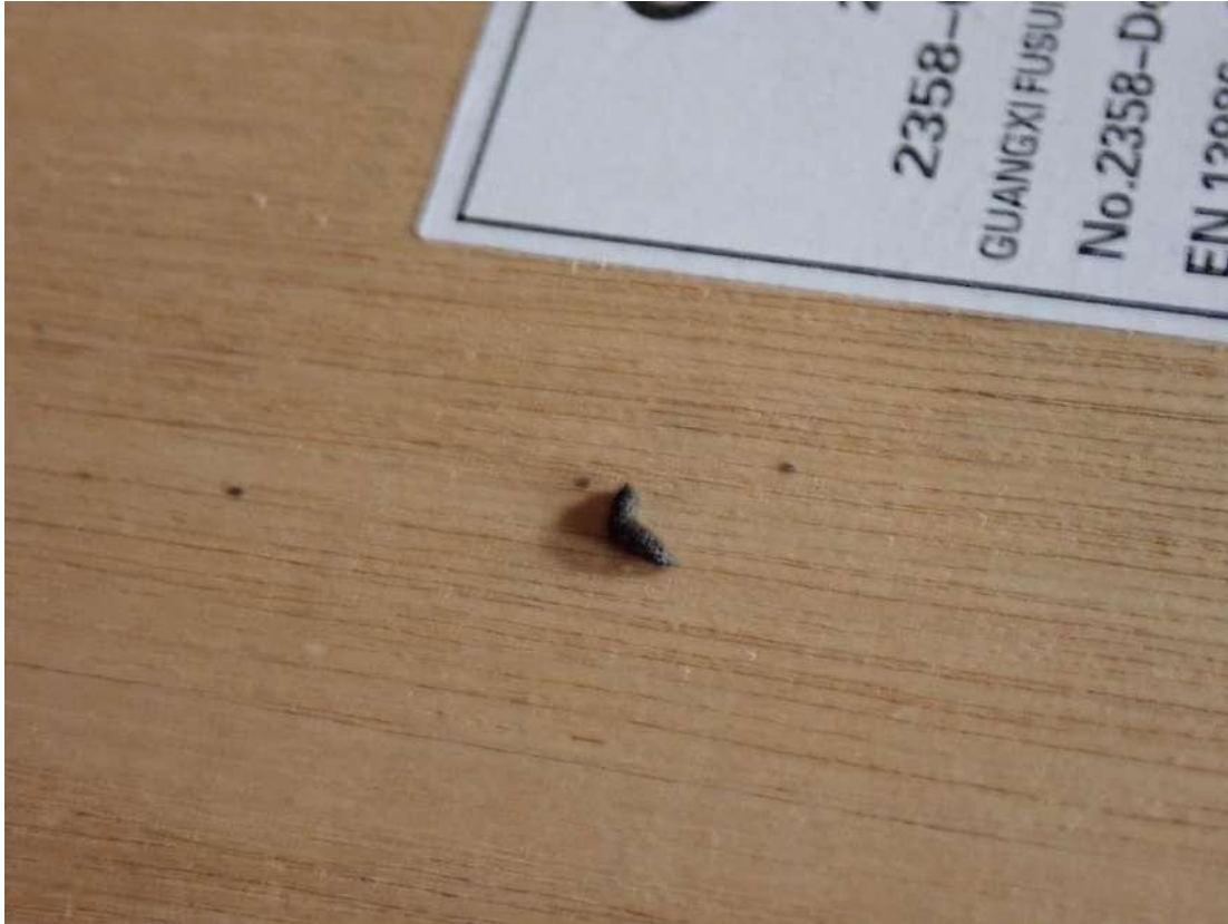
Photograph 65 - View of a bat dropping located in the ground floor of the barn section of Building 3.
