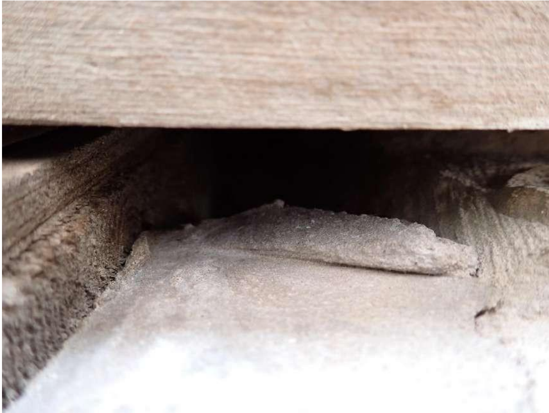
Photograph 25 – View of the cavity extending up to the wall plate, located behind the fascia board on the southern aspect of Building 3.
