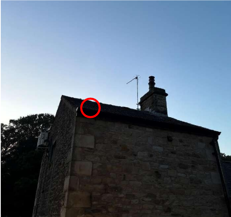
Photograph 69 – View of the entrance to Roost 3 circled in red, located on the western aspect of Building 2.
