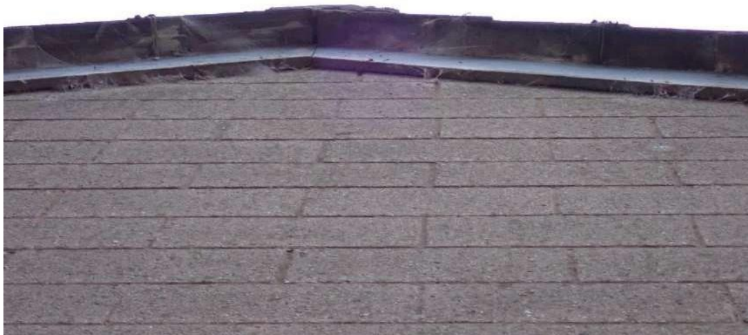
Photograph 4 – View of the gaps under the bargeboards on the eastern aspect of Building 1.
