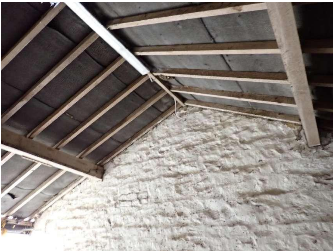
Photograph 42 – View of the bitumen lining the central room of the pig styes of Building 2.
