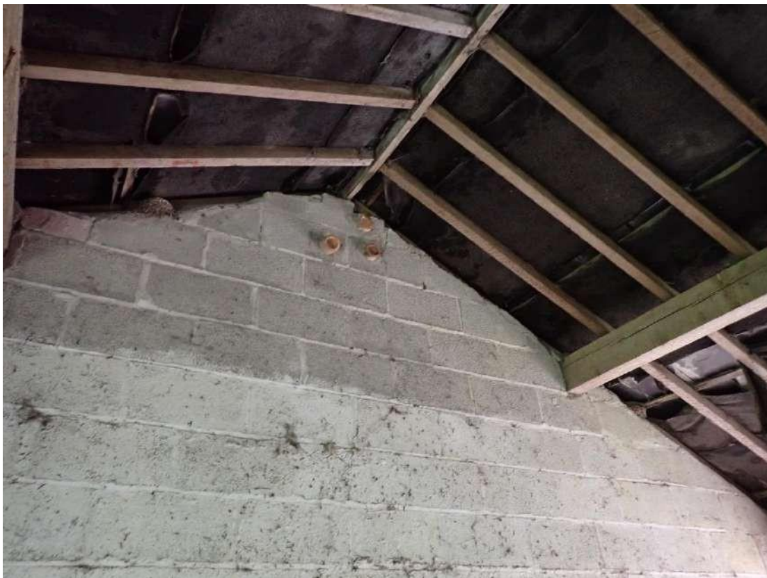
Photograph 46 - View of the damaged sections of the brickwork in the internal walls of the pig sty section of Building 2 leading to the wall cavity.
