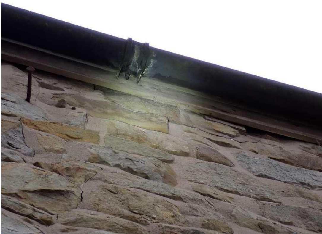
Photograph 24 – Close in view of the gaps between the fascia boards on the southern aspect of Building 3.
