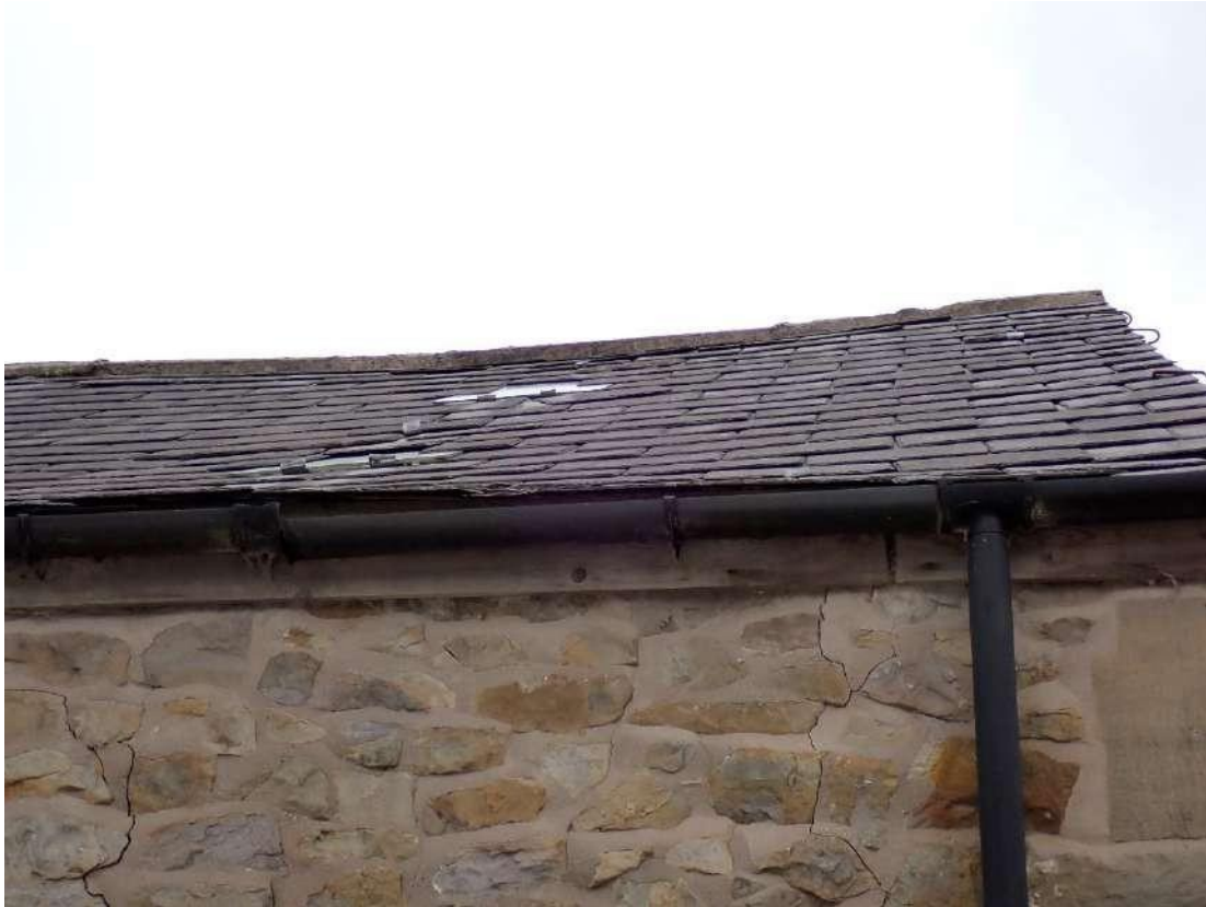
Photograph 21 - View of the raised tiles on the southern aspect of Building 3, forming PRFs.
