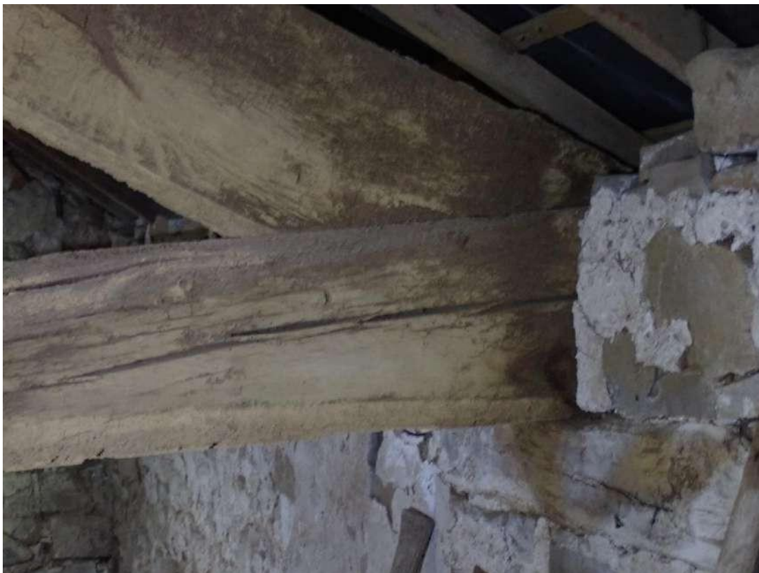
Photograph 60 – View of a PRF formed from cracks in the timber beams in the barn section of Building 3.
