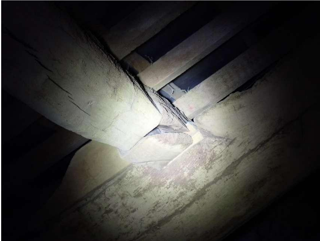
Photograph 59 – View of a PRF formed by ill-fitting joints in the timber structure of the barn section of Building 3.
