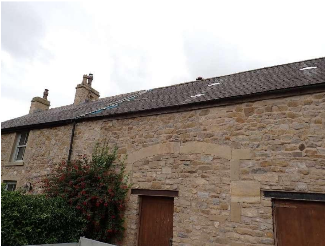
Photograph 22 – View of the southern aspect of Building 3 and the flashing around the chimneys and the skylights which is in good condition.
