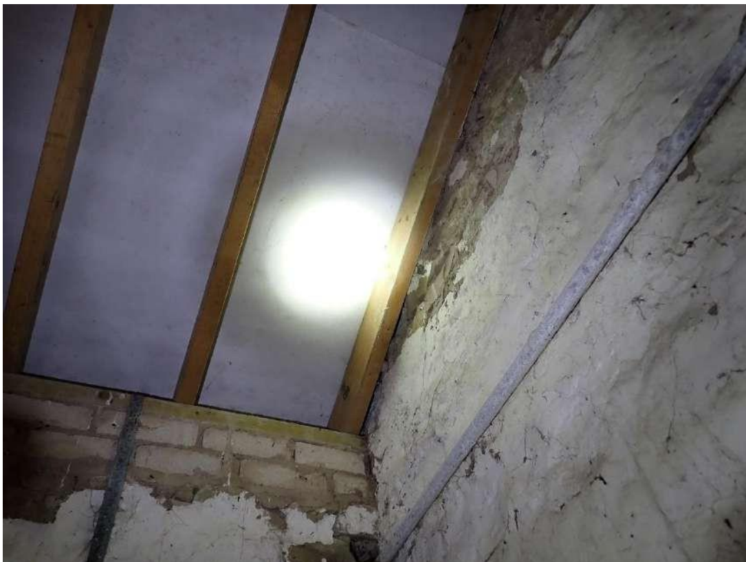
Photograph 40 – View of the PRFs in the gable ends where the timber of the roof ends.
