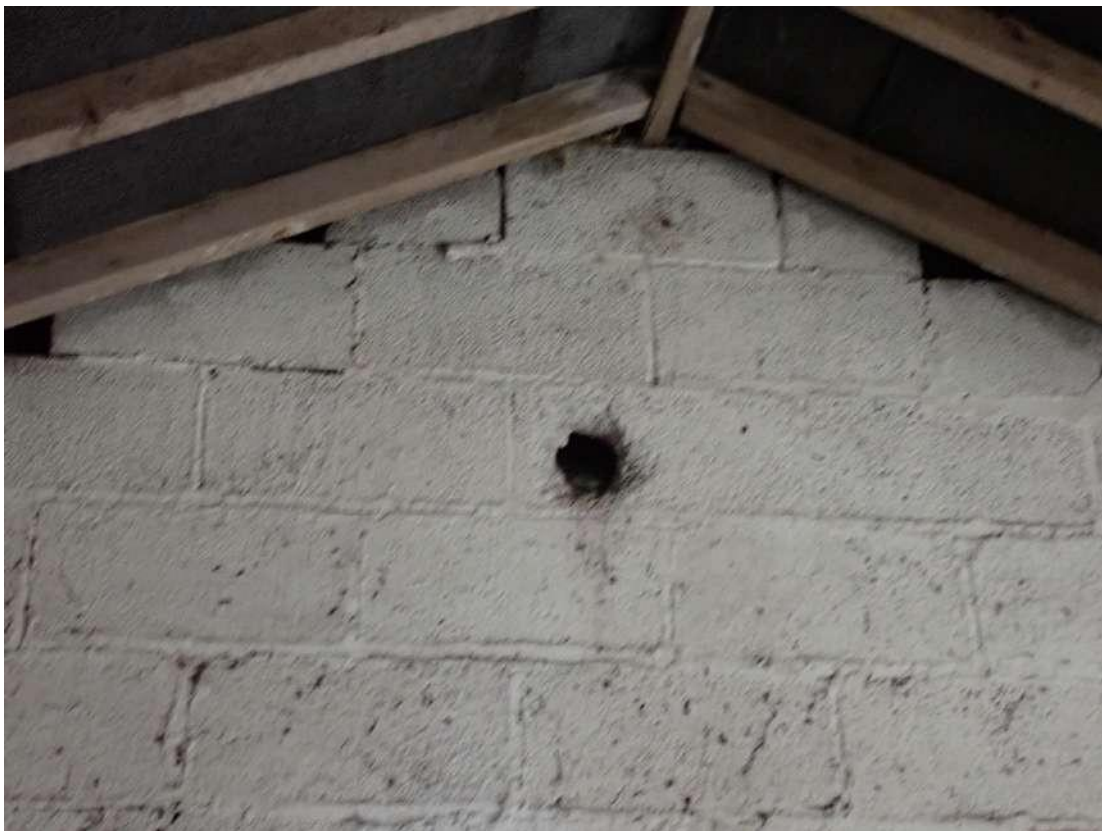
Photograph 48 – View of a hole in the breezeblocks at the gable end leading to the wall cavity in the eastern room of the pig sty section of Building 2.
