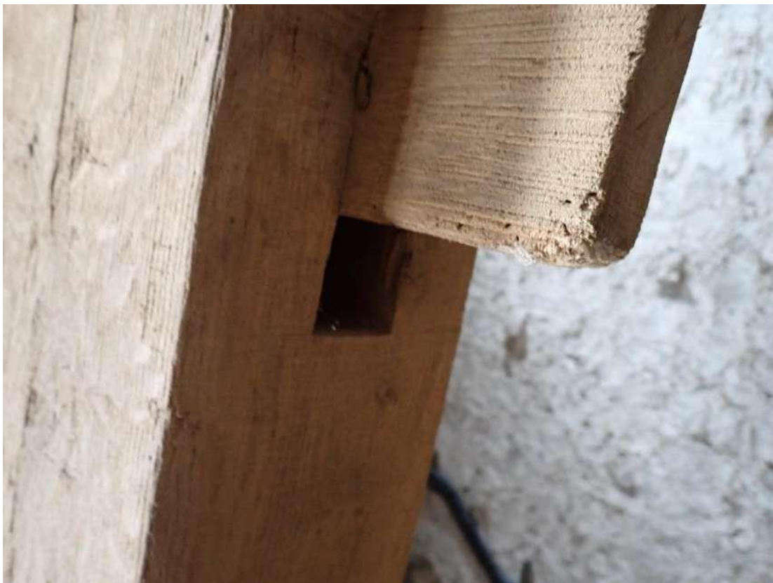
Photograph 58 – View of a PRF in the form of a gap around mortice joints in the wooden beams in the barn section of Building 3.
