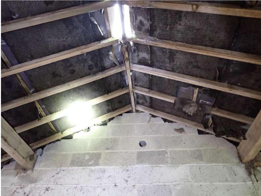
Photograph 43 - View of the damaged section of the bitumen lining of the middle room of the pig styes in Building 2.
