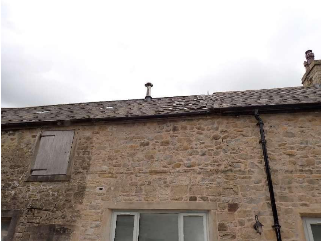
Photograph 27 – View of the PRF formed by cracks in the brickwork on the northern aspect of Building 3, where the newer extension meets the older barn.
