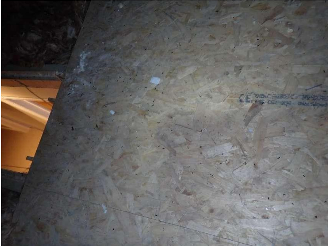
Photograph 55 – View of the numerous fresh bat droppings scattered over the chipboard lining the floor of the loft in the farmhouse of Building 3.
