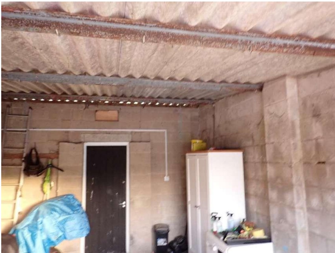
Photograph 8 – Internal view of the gaps behind the fascia boards in the garage attached to Building 1.
