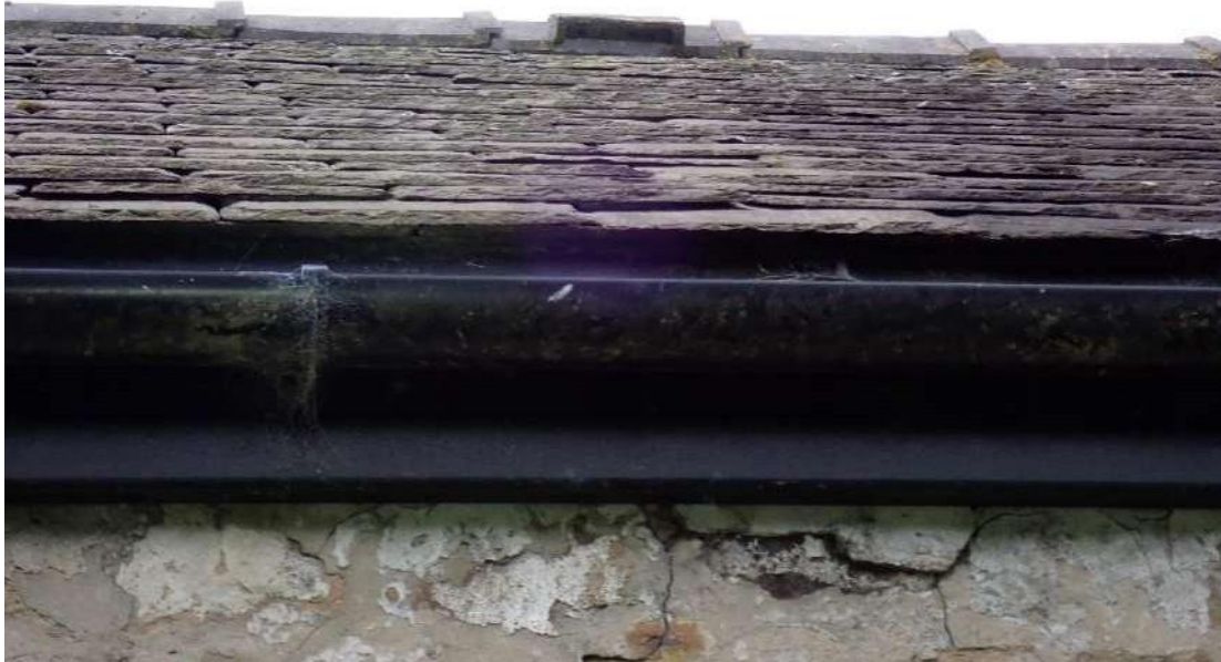
Photograph 11 – View of PRFs formed from raised roof tiles on the eastern section of Building 2.
