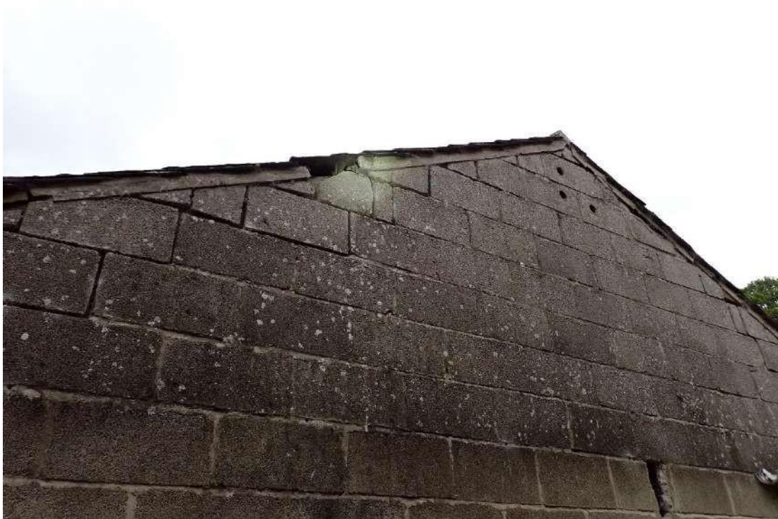
Photograph 15 – View of access points into the wall cavities of Building 2 via areas of damaged brickwork at the eastern gable end.
