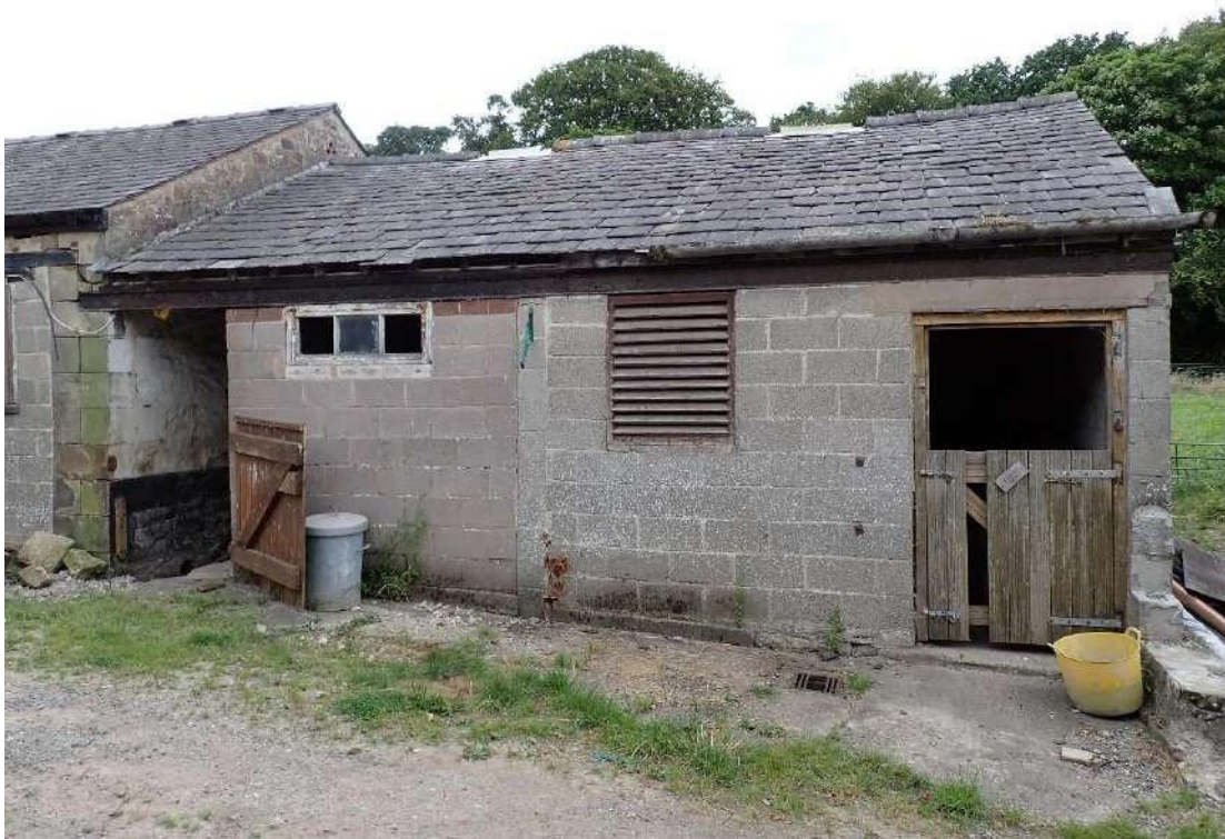
Photograph 19 - View of the open windows allowing access to the interior of the eastern section of Building 2.
