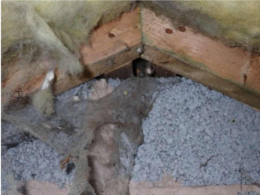
Photograph 35 - View of the gaps in the interior walls which allow access to the wall cavities.
