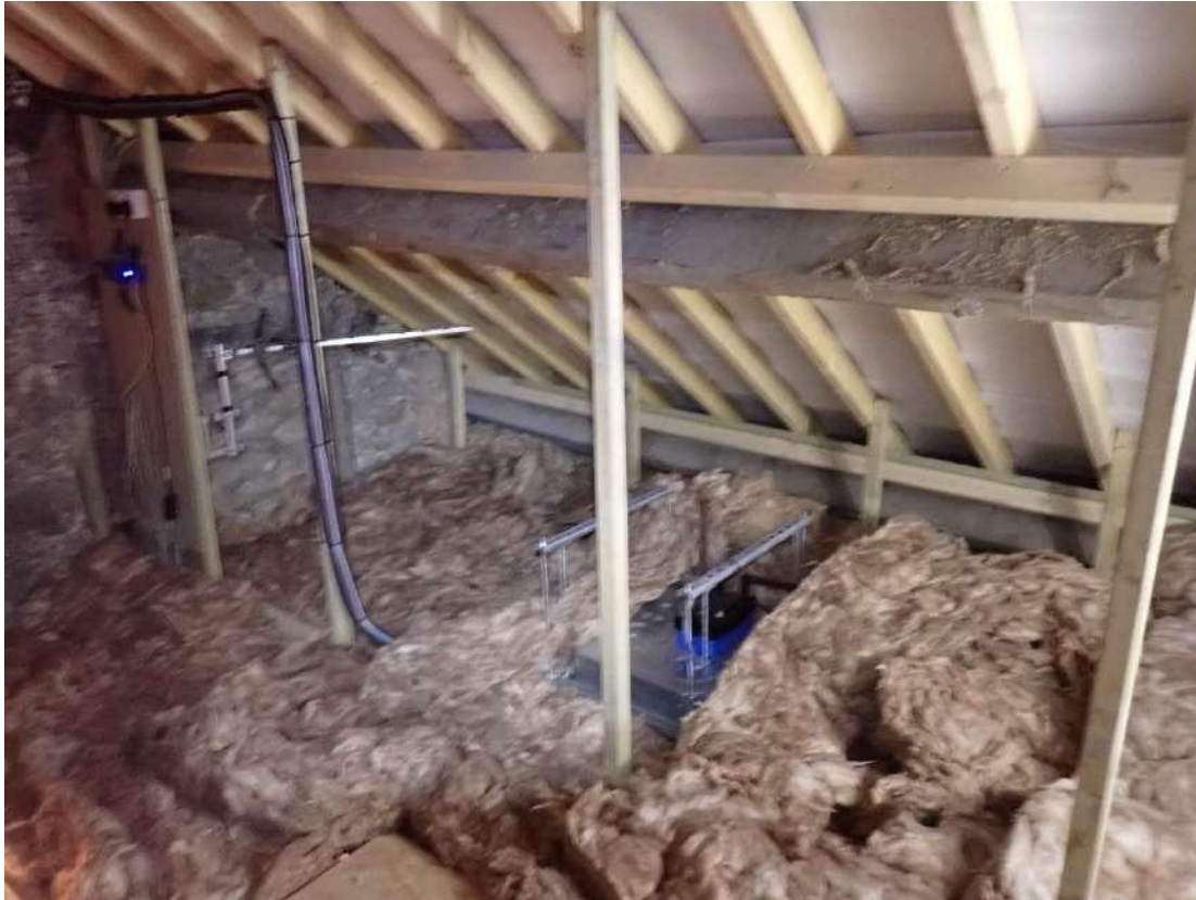
Photograph 51 - View of the internal loft space located within the farmhouse section of Building 3.
