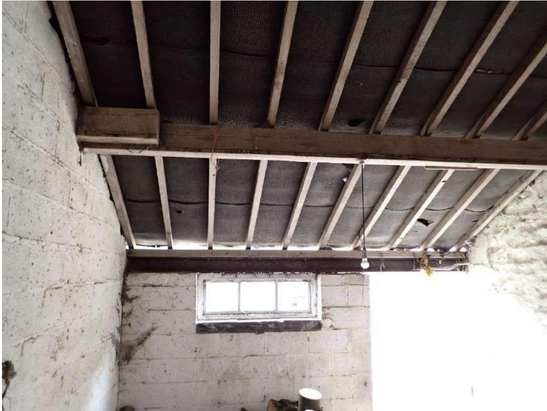
Photograph 47 – View of the gap in the wall above the final brick and the beam allowing access into the wall cavity of the eastern room of the pig sty section of Building 2.
