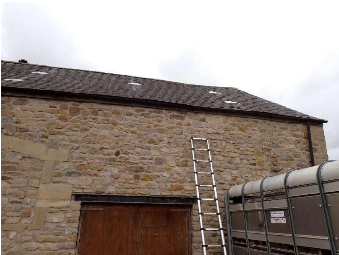
Photograph 26 – View of the location where droppings were observed on the southern aspect of Building 3.
