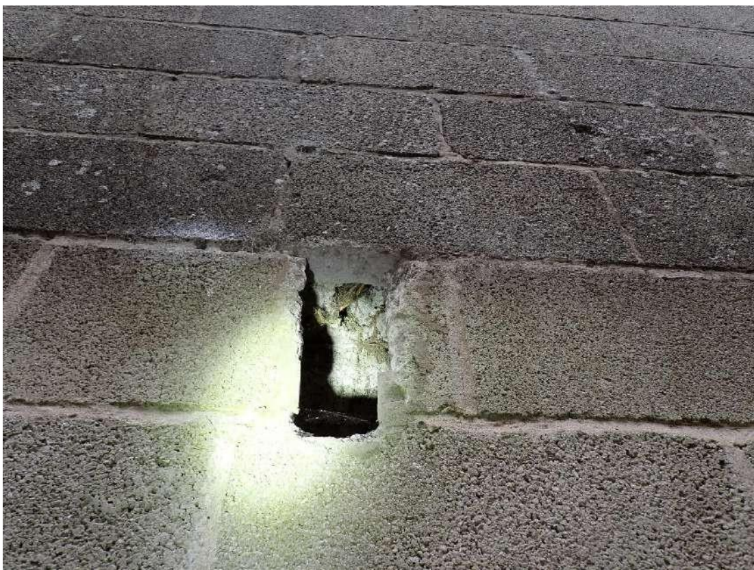
Photograph 16 – View of an access point into the wall cavity in the eastern section of Building 2, located on the eastern gable end.
