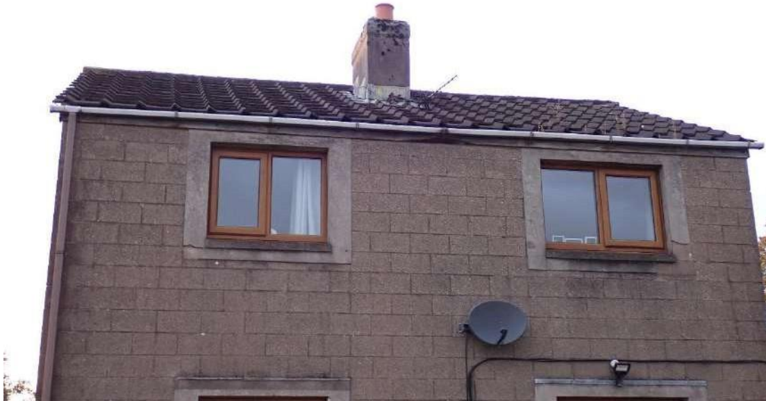
Photograph 3 – View of the PRFs formed from damaged fascia boards on the southern aspect of Building 1.
