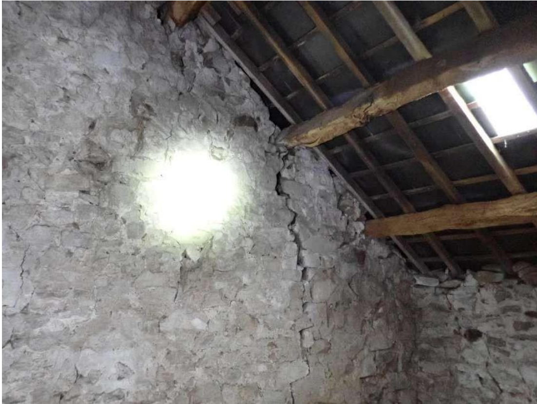
Photograph 61 - View of the cracks in the gable end and missing mortar at the wall plates in the barn section of Building 3.
