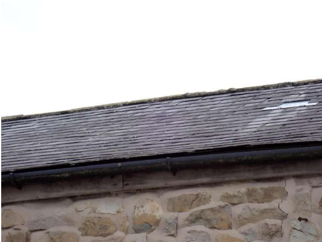
Photograph 23 – View of the gaps behind the fascia board on the southern aspect of Building 3.
