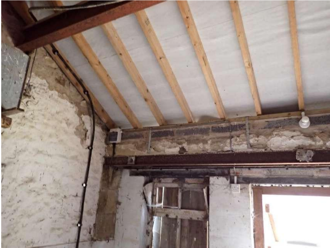
Photograph 41 - View of the gaps above the wall plate in the western room of the pig styes of Building 2.
