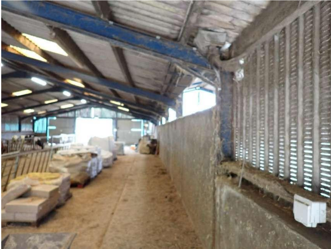
Photograph 67 – View of the interior of Building 4 showing the well lit and exposed conditions inside the building.
