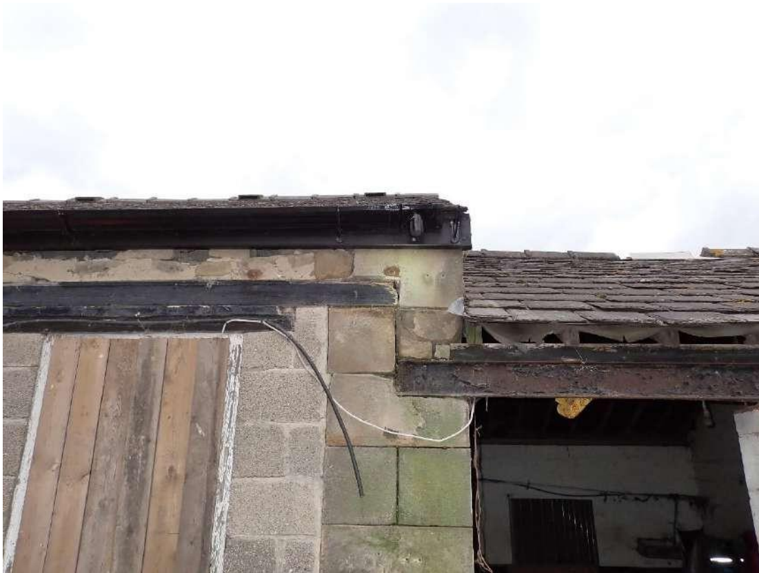
Photograph 17 – View of gaps in the brickwork on the southern aspect of Building 2.
