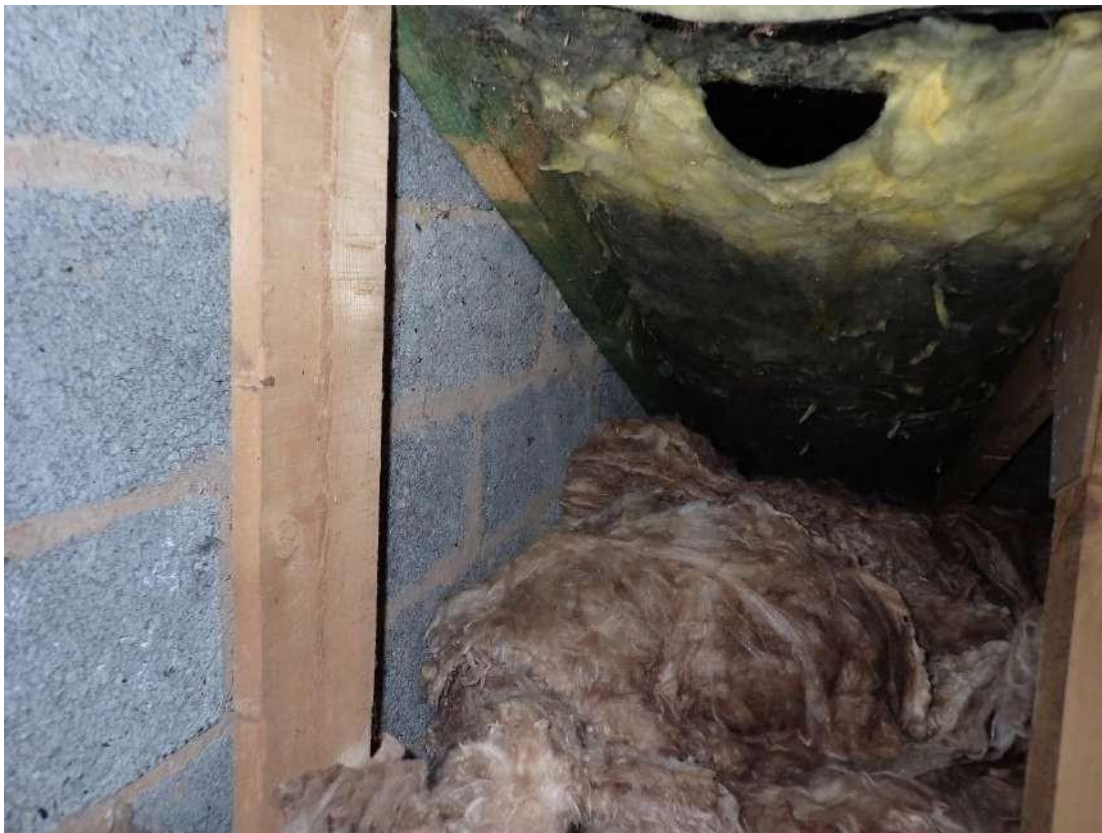
Photograph 36 - View of a hole in the mineral wool roof insulation leading to the underside of the tiles.
