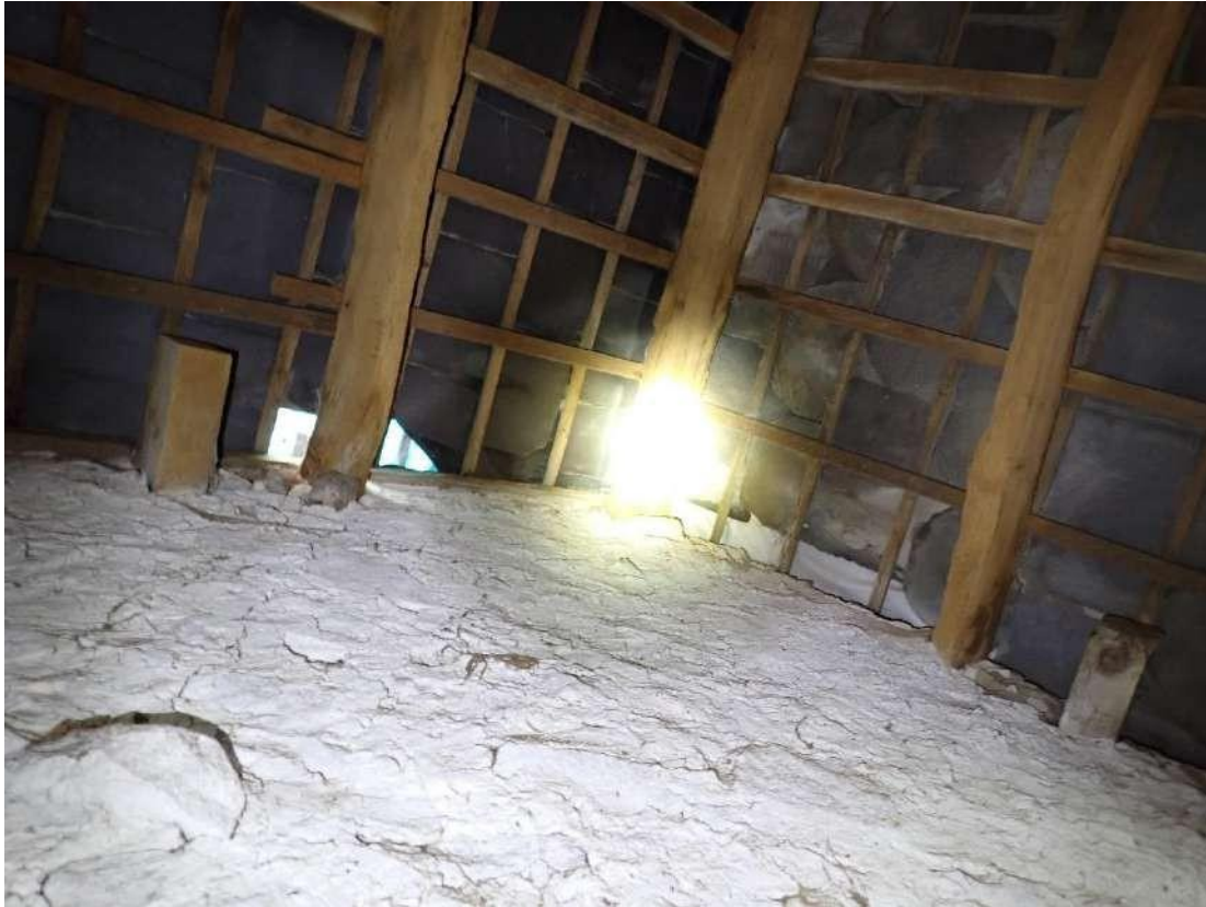
Photograph 57 – View of the underside of the roof of the barn section of Building 3, showing gaps in the tiles and an absence of lining.
