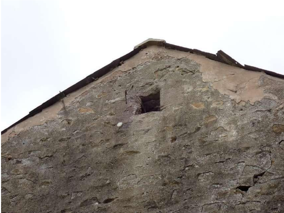
Photograph 29 – Close view of the PRF formed by the ventilation hole near the apex of the eastern gable end of Building 3.
