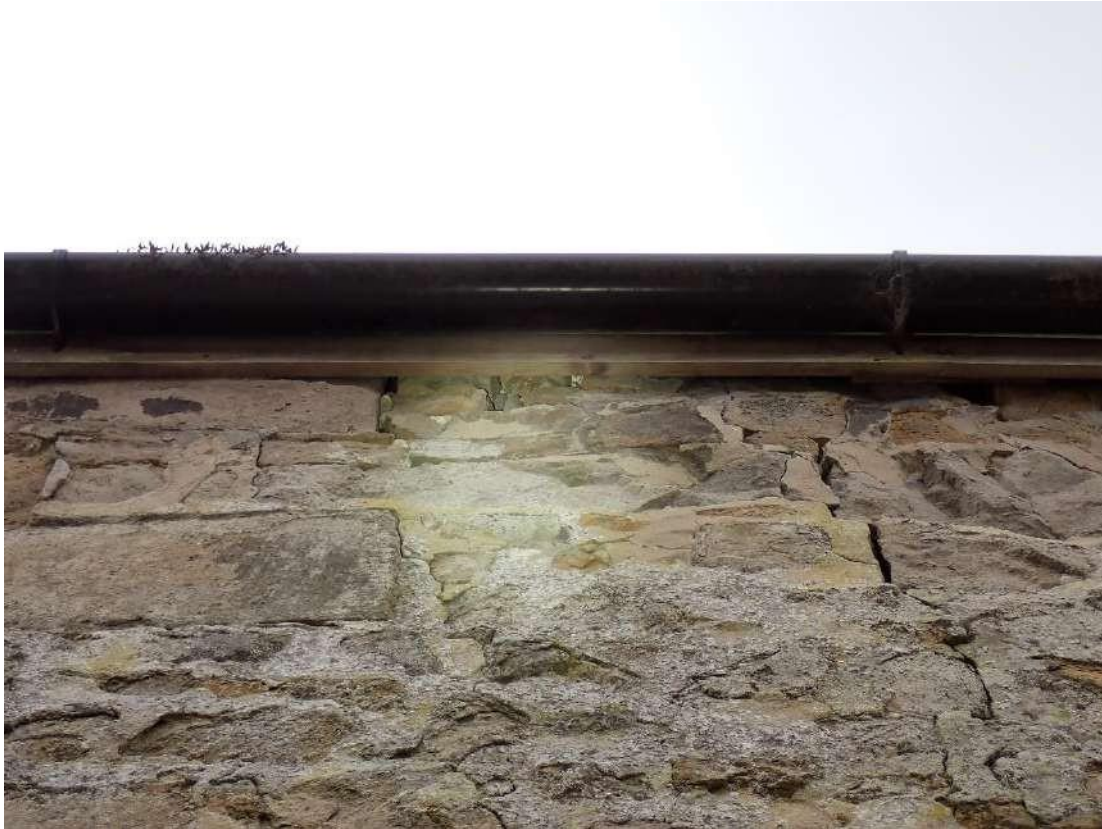
Photograph 13 – View of access points into Building 2 formed from missing mortar behind the fascia boards.
