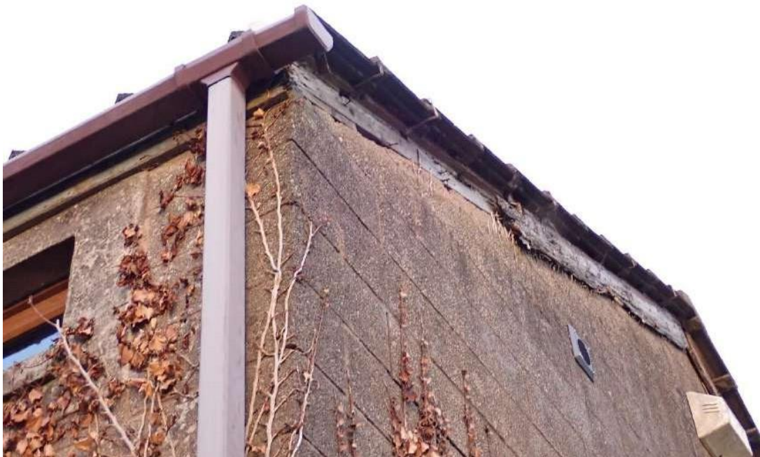
Photograph 6 - View of a missing section of bargeboard on the western aspect of Building 1.
