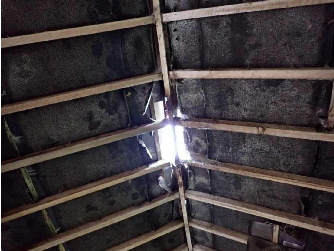
Photograph 45 – View of the damaged bitumen lining in the eastern room of the pig sty section of Building 2.
