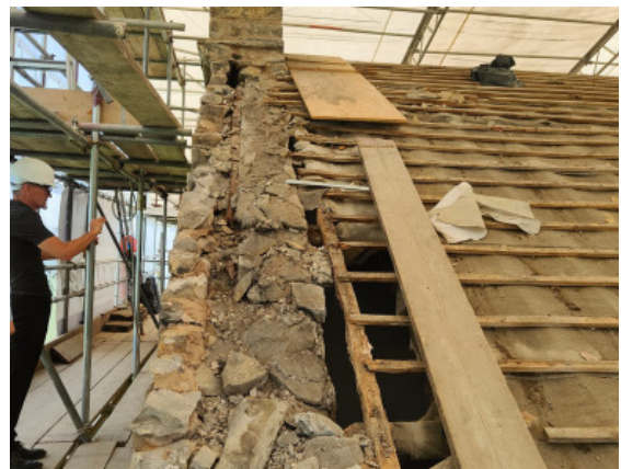
Roof not water tight
