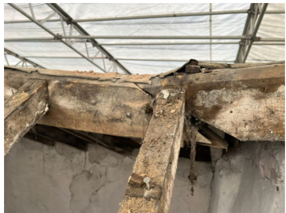
Rotten softwood ridge beam
