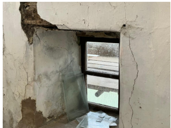
Internal water ingress causing rot and cracking
