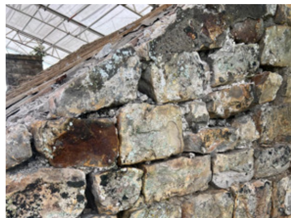
Walls in disrepair
