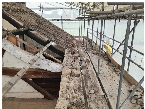
Rear Wall Bowing
