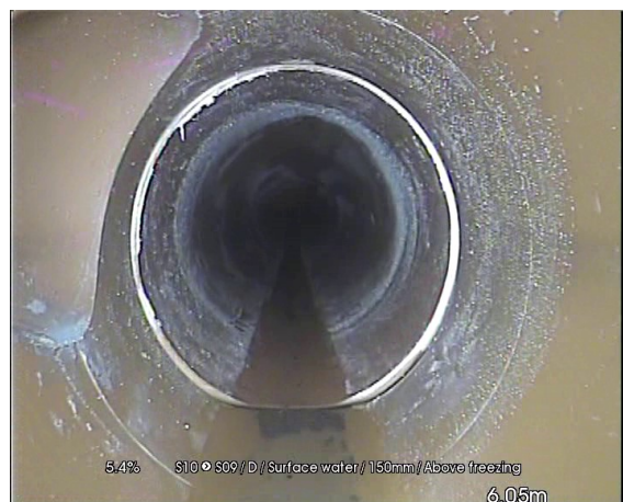
S10X_50b5d0d3-e8fd-429b-bef8-979ea171d560_20250113_085426_991.jpg, 00:00:41, 6.05 m Junction at 10 o'clock, diameter: 100mm
