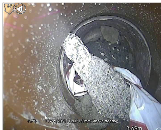
F20X_3d84a70f-4581-490e-ad73-6543cc097683_20250113_094433_129.jpg, 00:00:28, 3.65 m Junction at 1 o'clock, diameter: 100mm
