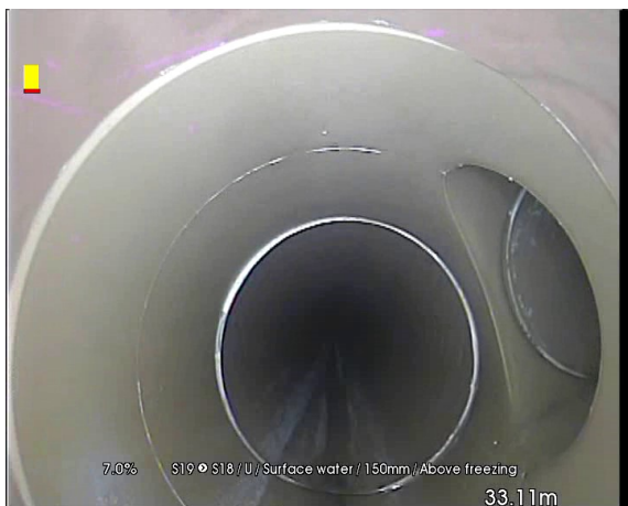
S19X_760acfd5-202e-424c-8b42-26ac3cacf73e_20250113_082802_885.jpg, 00:03:32, 33.11 m Junction at 3 o'clock, diameter: 100mm
