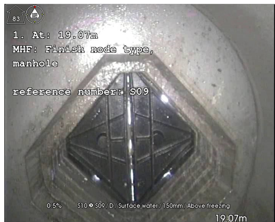
S10X_8bf43c25-5d20-400b-9aaa-4247d52b0cf5_20250113_085624_334.jpg, 00:02:06, 19.07 m Finish node, manhole, reference: S09
