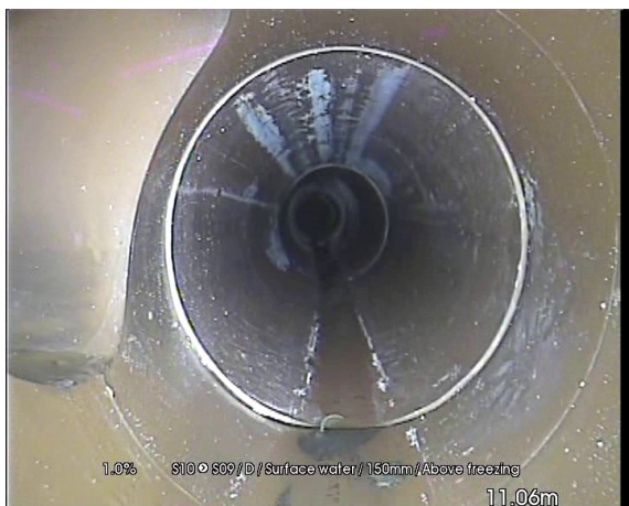
S10X_4ee92ac1-4a4e-43dc-972d-f44ff607f18a_20250113_085517_857.jpg, 00:01:13, 11.06 m Junction at 10 o'clock, diameter: 100mm
