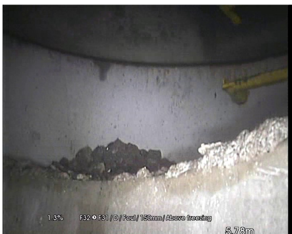
F32X_215f00d8-43ff-4ab6-8c6e-f14bd1ddca18_20250113_082026_450.jpg, 00:01:02, 5.78 m Finish node, manhole, reference: F31
