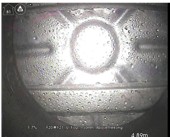
F21X_14a05c3f-1eea-45f5-a783-61f1c9508b32_20250113_10 0202_748.jpg, 00:00:35, 4.89 m Finish node, manhole, reference: F21
