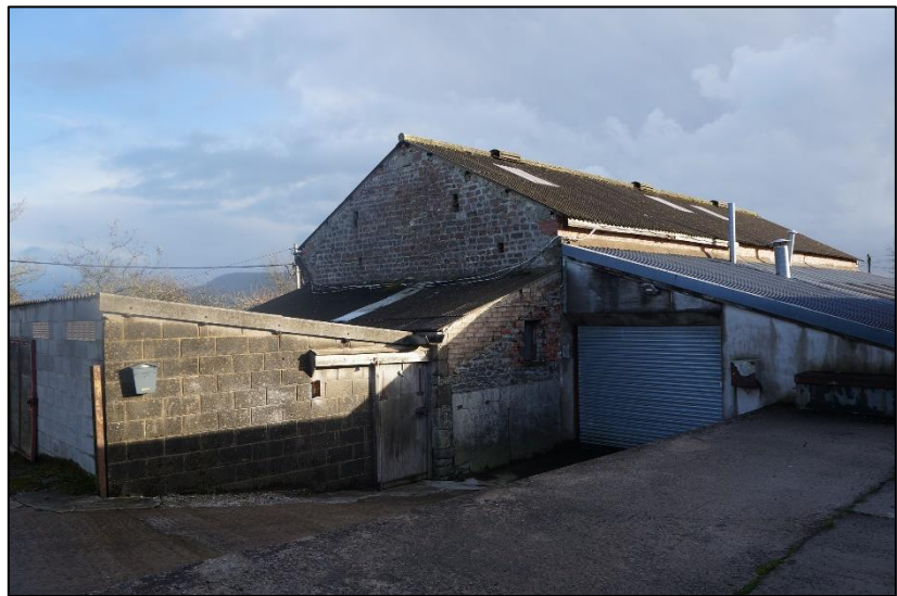
Photo 2: Northwest elevations of the barn, showing the area where the single storey extensions have been added.
