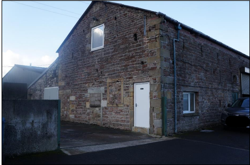
Photo 3: South & east elevations of the building, the gable end having less gaps and potential roosting features than other elevations.
