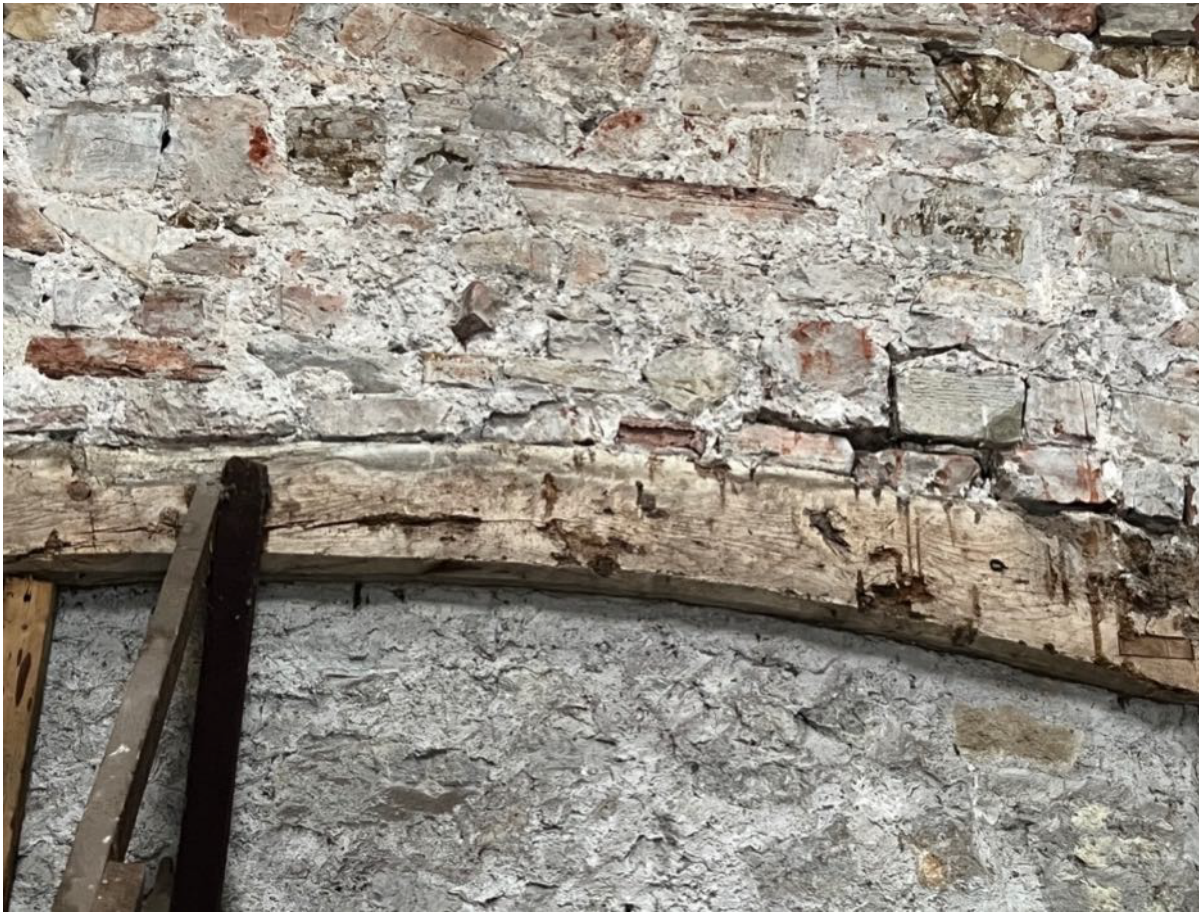
Photo 26 – Timber curved lintel to former opening in rear elevation of main barn
