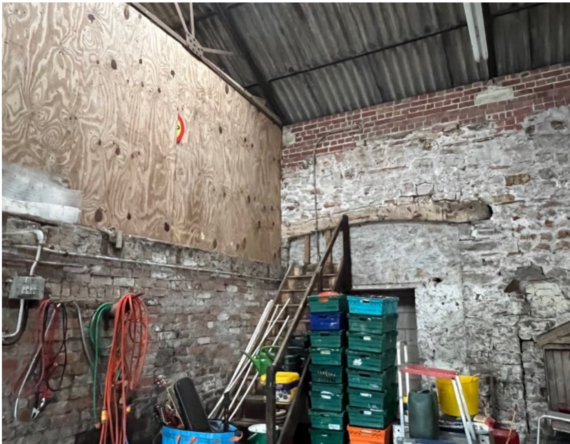
Photo 20 - Internal with storage at North East End and South West Wall internal
