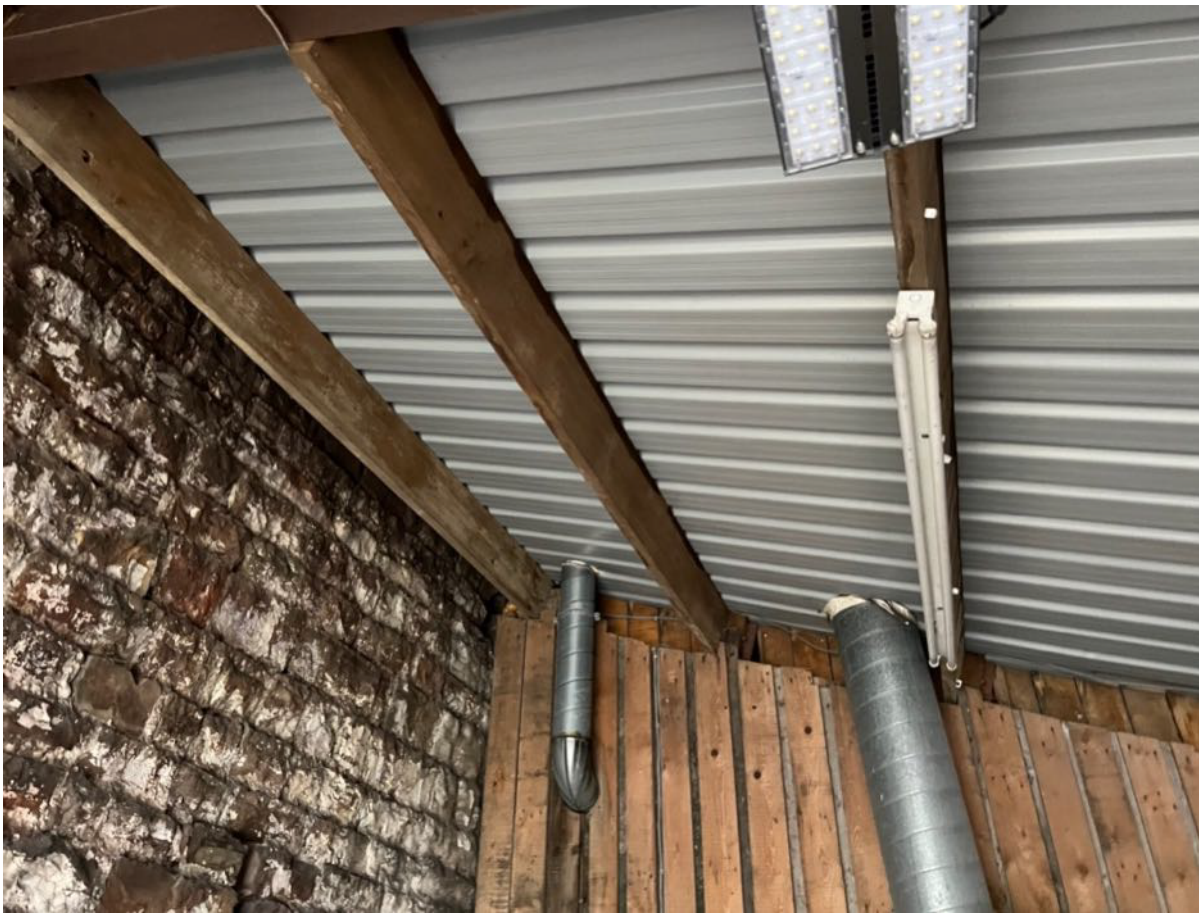
Photo 29 – Rear south west wall of main barn and roof to rear lean to
