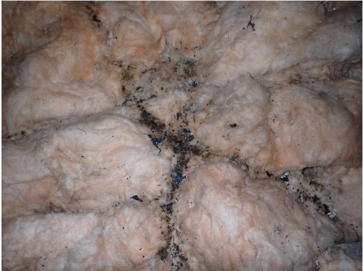
11 – Mouse droppings and runs were present in each of the roof voids inspected.
