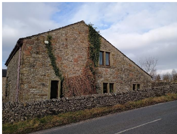
Photograph 8: Collapsed ivy on southeast elevation of B1
