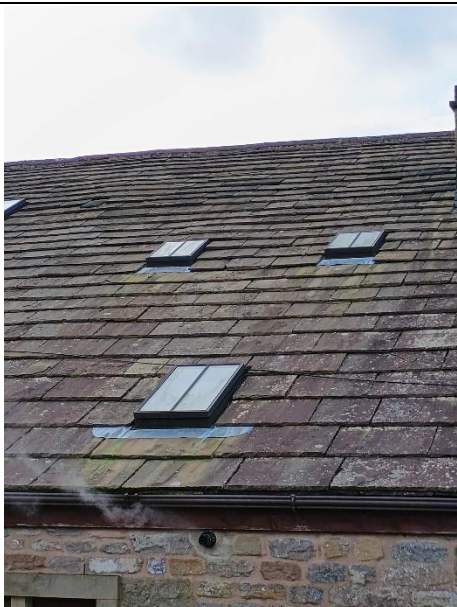
Photograph 7: Gaps between tiles on northeast elevation of B1
