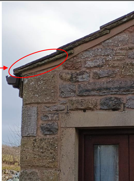
Photograph 6: Gap underneath tile on northwest elevation of B1
