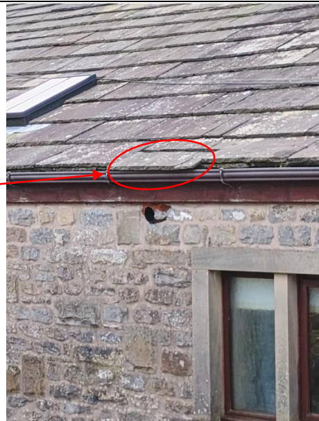
Photograph 4: Example of slipped tile on B1
