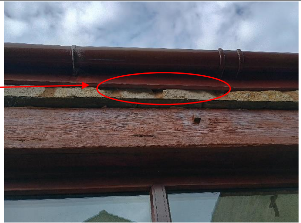
Photograph 12: Example gap underneath fascias on southeast elevation of B2
