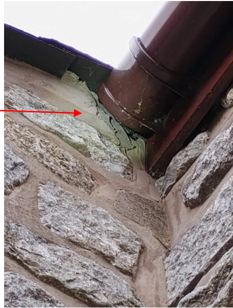
Photograph 18: Gap underneath fascia board at the corner of the northeast/southeast elevation at B2
