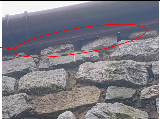
Photograph 14: Example gap underneath fascias on northwest elevation of B2
