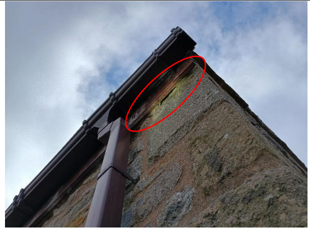
Photograph 2: Gap underneath fascia on northeast elevation of B1
