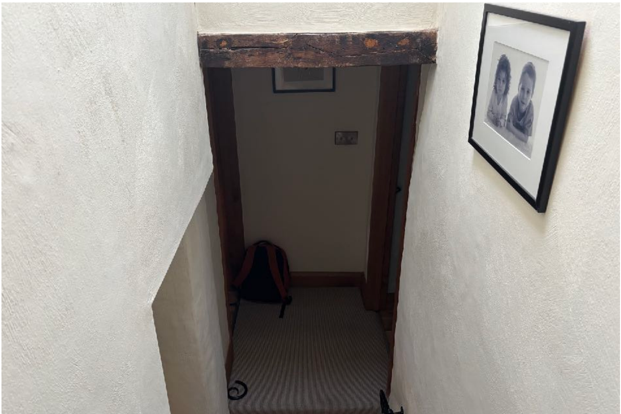
Figure 6: Altered lintel over bathroom/ bedroom entrance.
