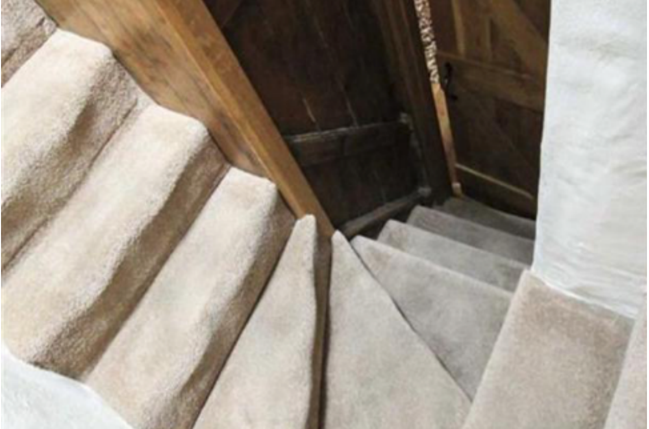
Figure 2: Prior stair from sales particulars, note the bathroom step discharging across two steps on the winder portion of the stair.
