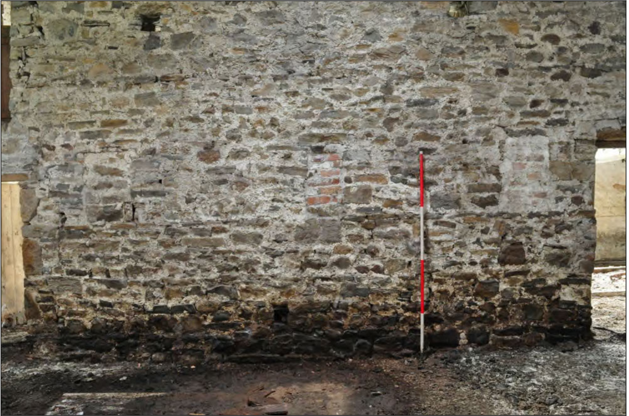
Photo 34: Main building: interior, blocked breathers in south side
