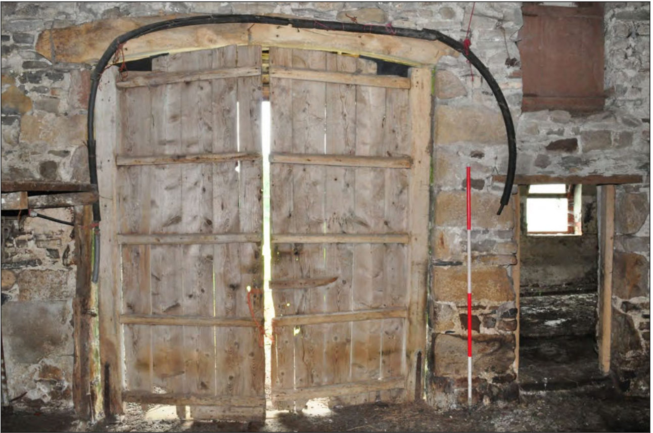
Photo 26: Main building: interior view of south cart entrance and inserted doorway to later shippon
