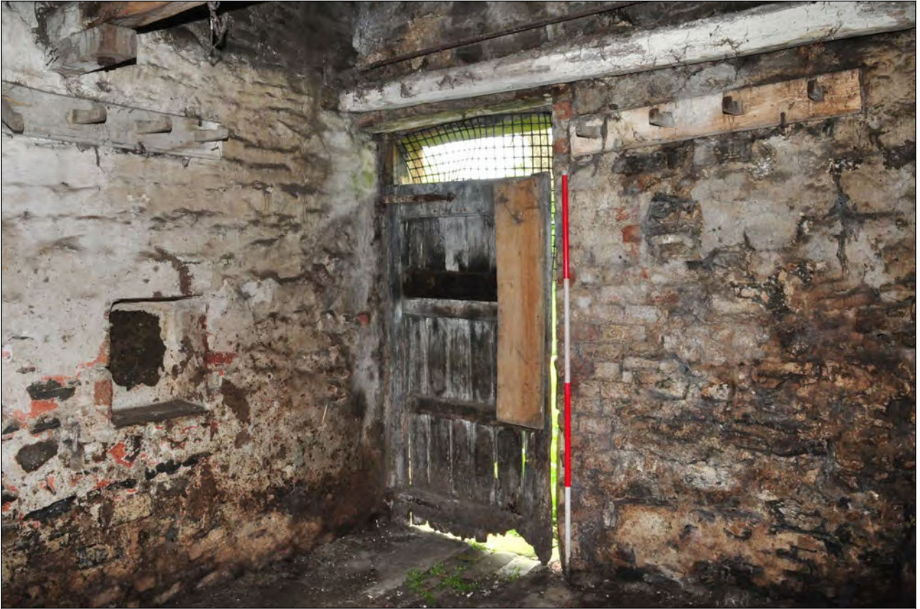
Photo 42: Main building: stable at west end, looking south-west
