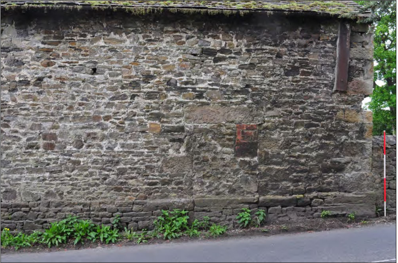
Photo 9: Main building: blocked doorway near west end of north elevation
