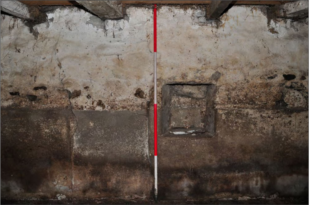
Photo 30: Main building: interior, detail of blocked doorway and lamp hole in back of shippon, looking east
