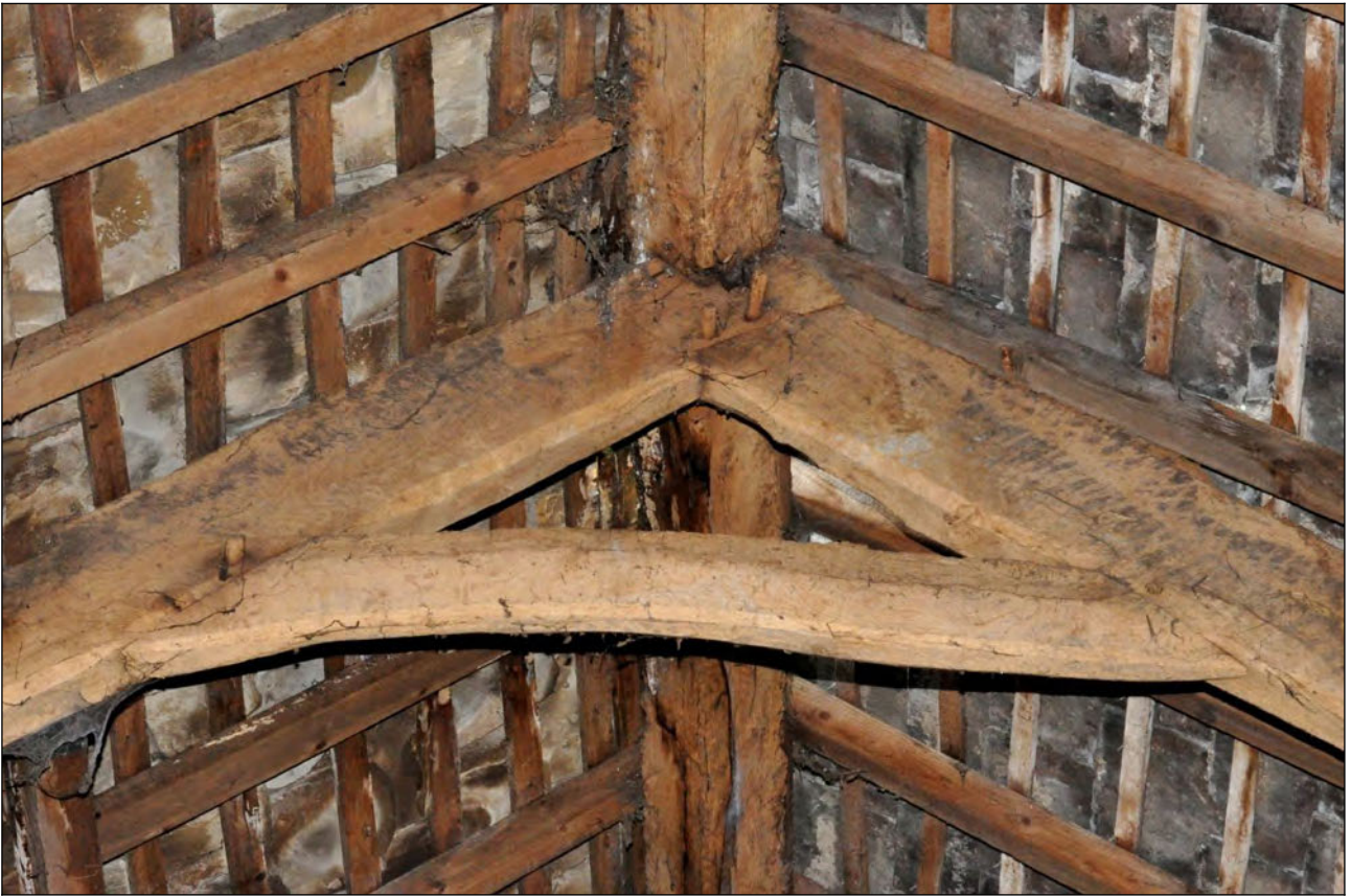
Photo 38: Main building: detail of collar and apex of roof truss, looking west
