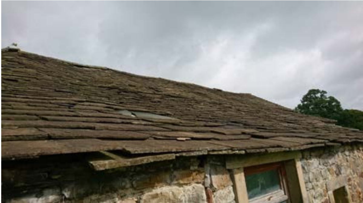
Figure 4: The roof over the Main Barn viewed from the south – covered with stone flags.
