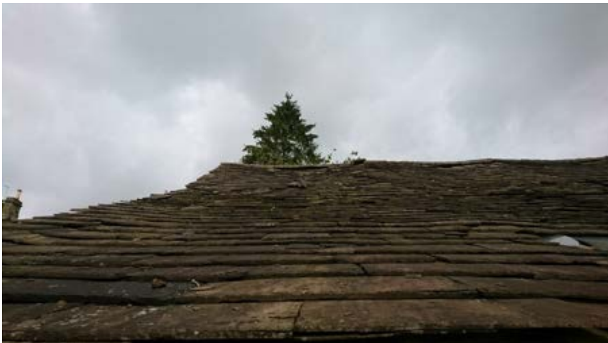
Figure 9: Separation of the ridge and the rafters below over the Stable / Store areas. note the large fillet of mortar which has become detached and was presumably used to fill the gap.
