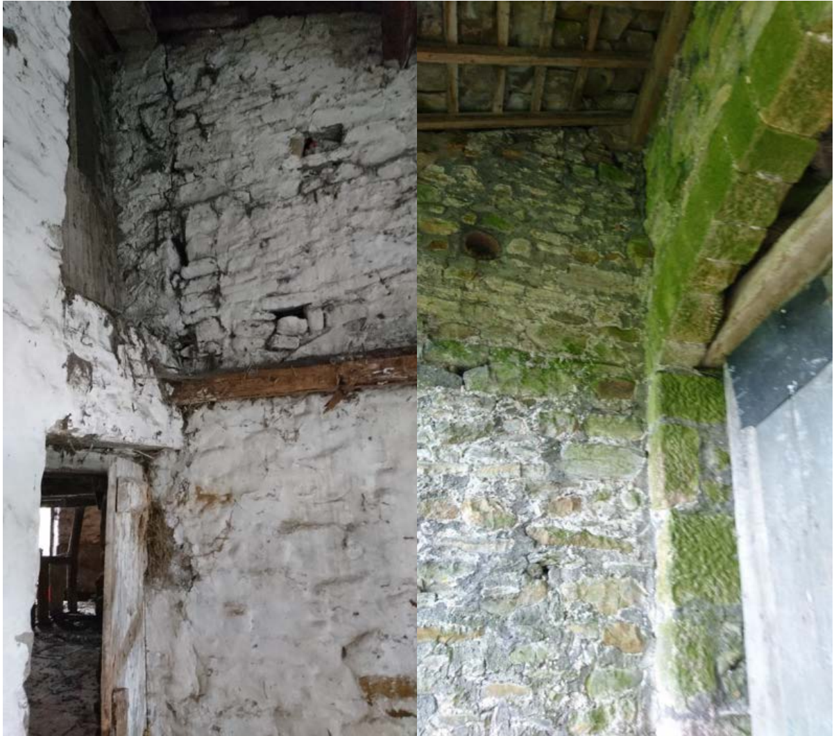
Figure 47: WP8, internally with a just visible tapering crack running down internally from eaves level (LEFT), which was not visible externally.
