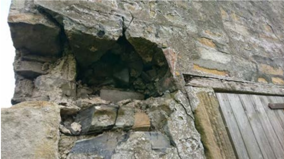
Figure 36: The missing quoin stone in WP5.
