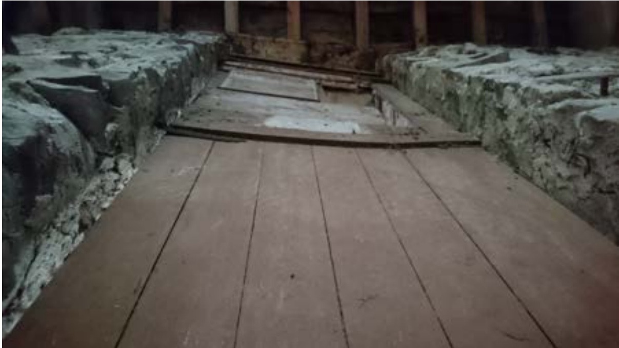
Figure 29: Potential buckling under compression of the door at first floor having been trapped under the outward thrust movement of the arch.
