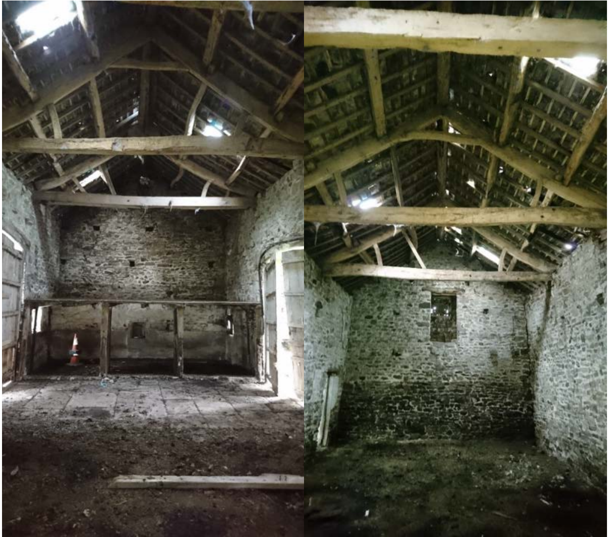
Figure 3: The roof from inside the Main Barn, viewed from the west (image left) and viewed from the east (image right).
