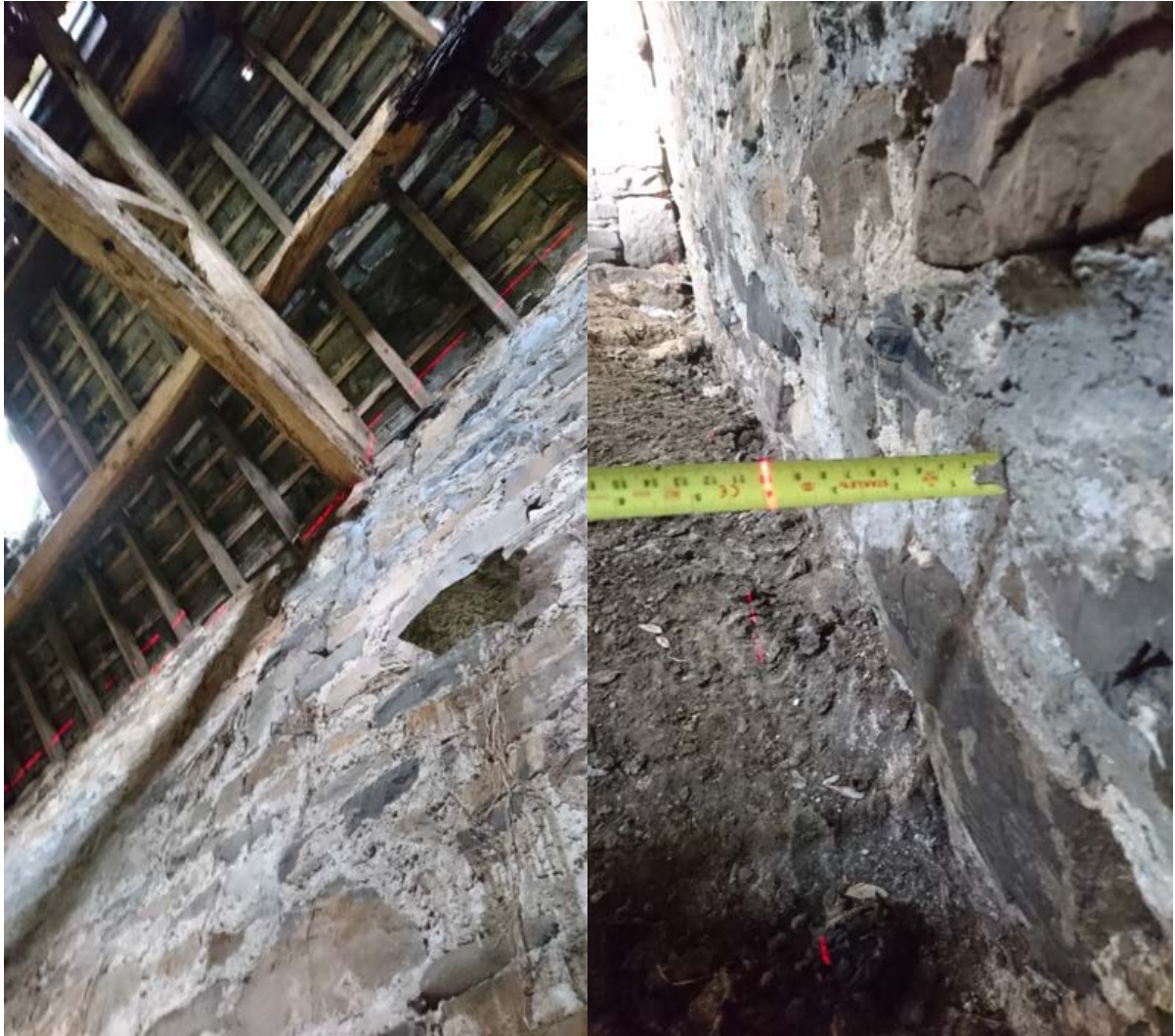
Figure 17: LEFT: Plumb laser trained on the bearing of Truss 4. RIGHT: Measurement of the maximum excursion from vertical at mid-height of the wall.
