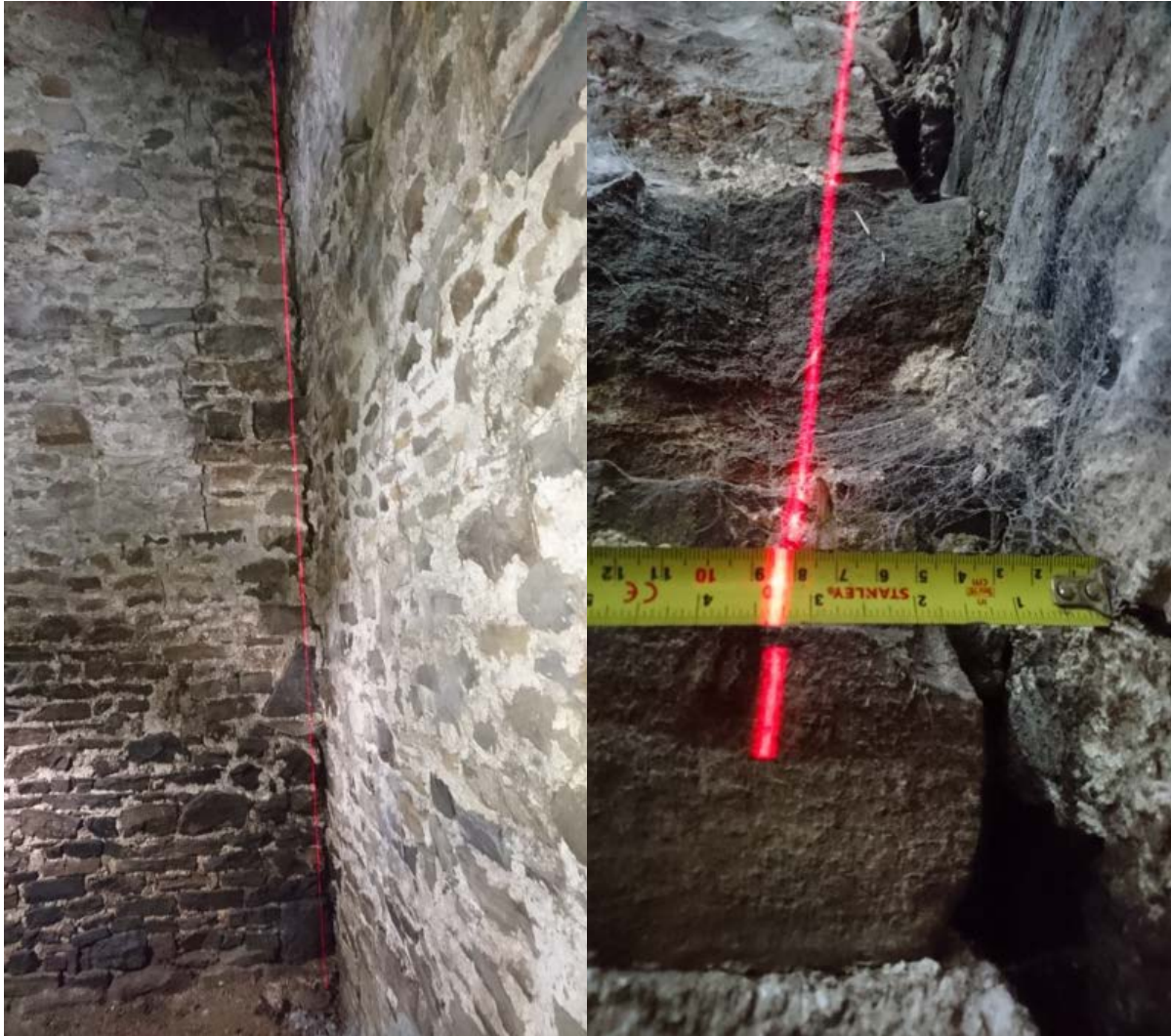
Figure 16: LEFT: Plumb laser highlighting the deviation from vertical at the abutment to the internal partition (WP4). RIGHT: Measurement of the maximum excursion from vertical.
