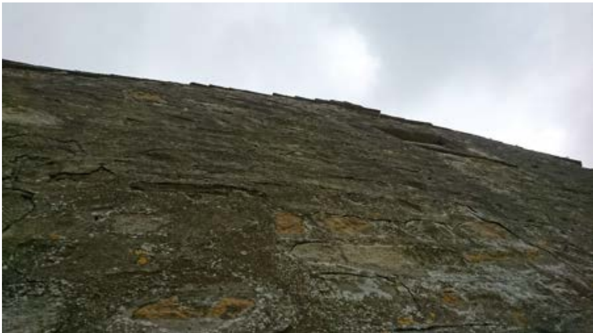
Figure 33: Undulating and bulged surface of WP5.
