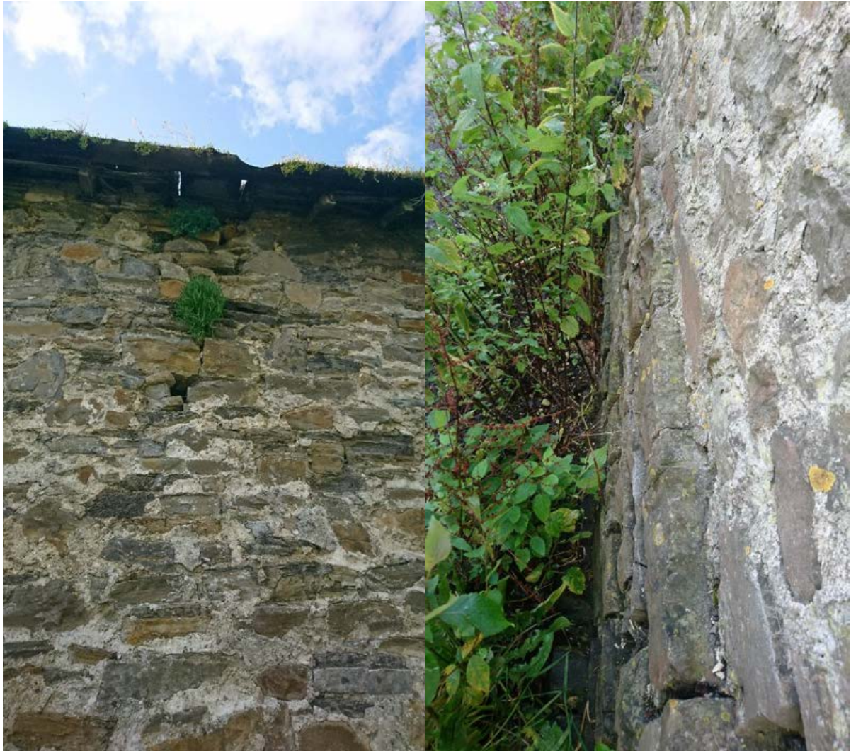
Figure 20: LEFT: Water damage under the leaking gutter. RIGHT: Stepped lower course construction.
