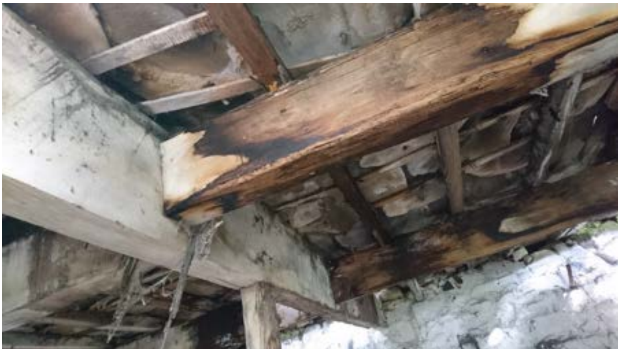
Figure 12: Example of superficial decay under holes in the roof.
