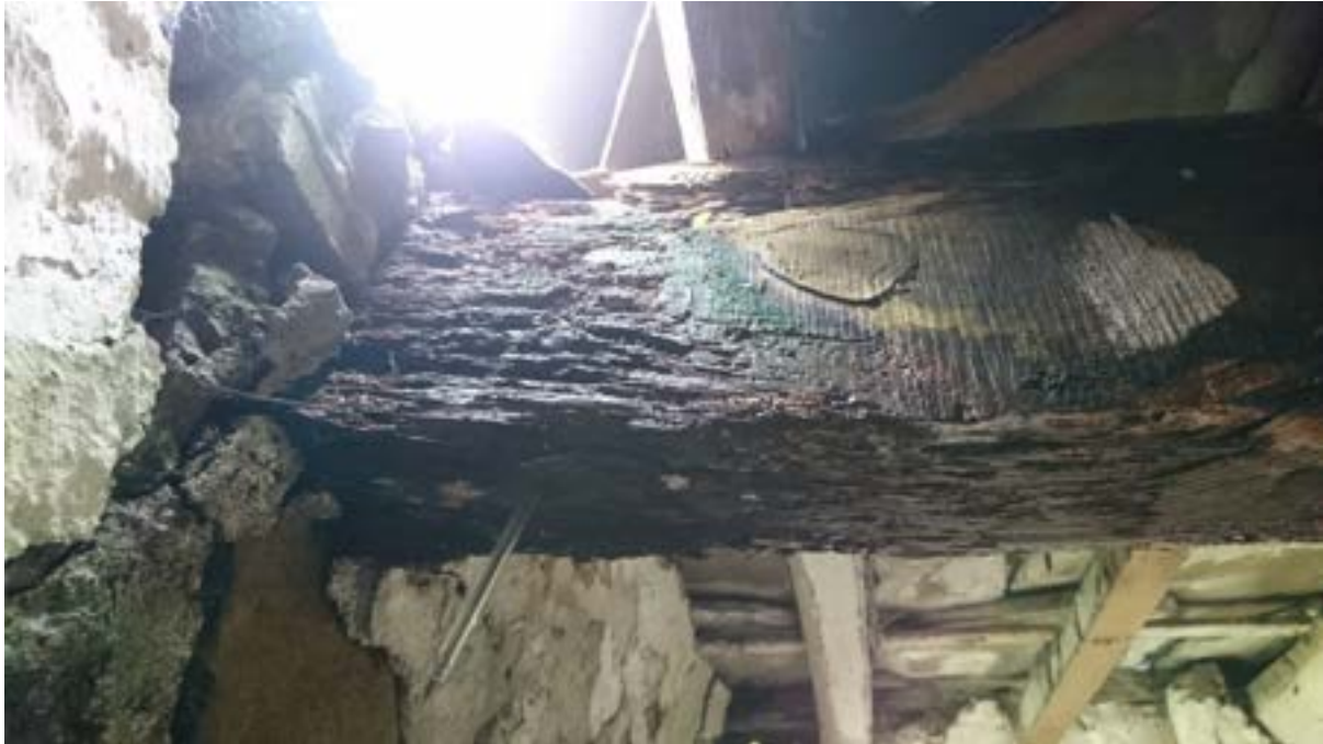
Figure 13: Example of heavy decay of a purlin at the eastern gable, note the embedded pen.
