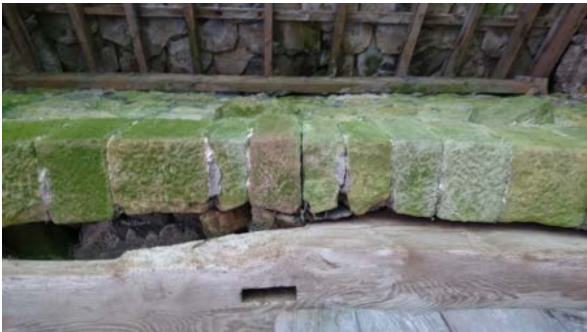
Figure 27: Opening of vertical joints of the masonry arch in WP3, consistent with outward movement under the outward thrust at one or both bearings.
