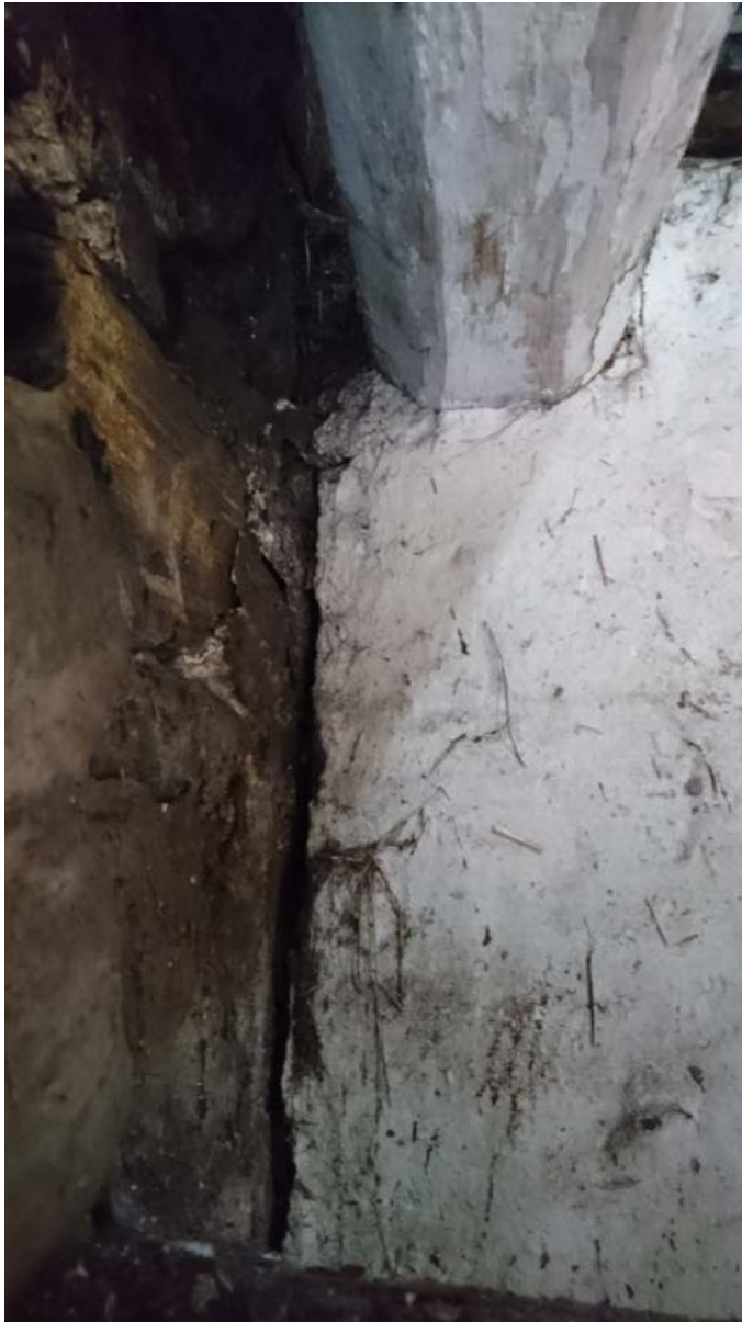
Figure 35: Separation of WP5 from the internal masonry partition between the stable and storeroom.
