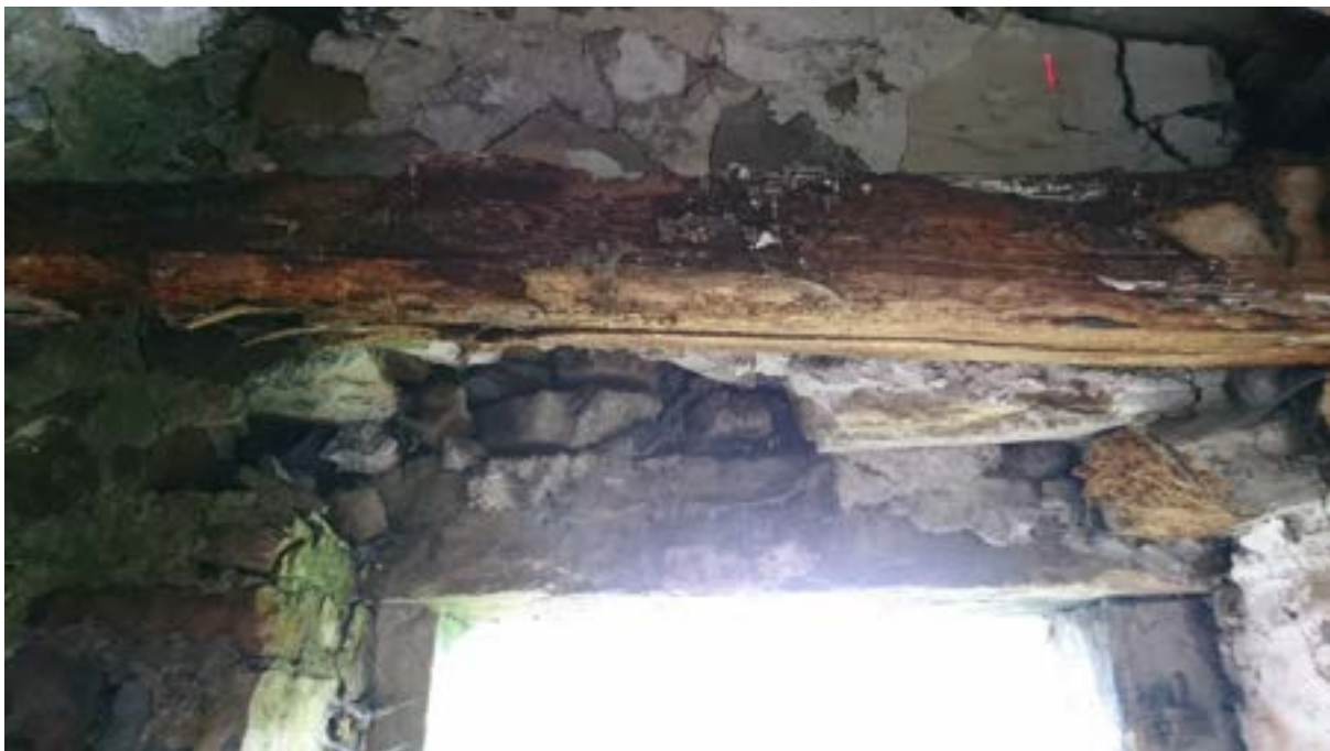
Figure 49: Failed timber lintel remains visible at the 'right hand' bearing just below the timber first floor beam.
