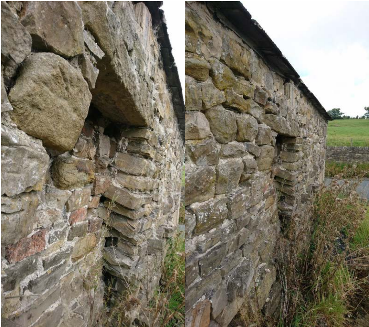
Figure 39: The eastern elevation of Extension 1. LEFT: Poor quality masonry blocking the opening. RIGHT: The stepped-out nature of the shearing crack visible over the blocked-up opening, just below the gutter.
