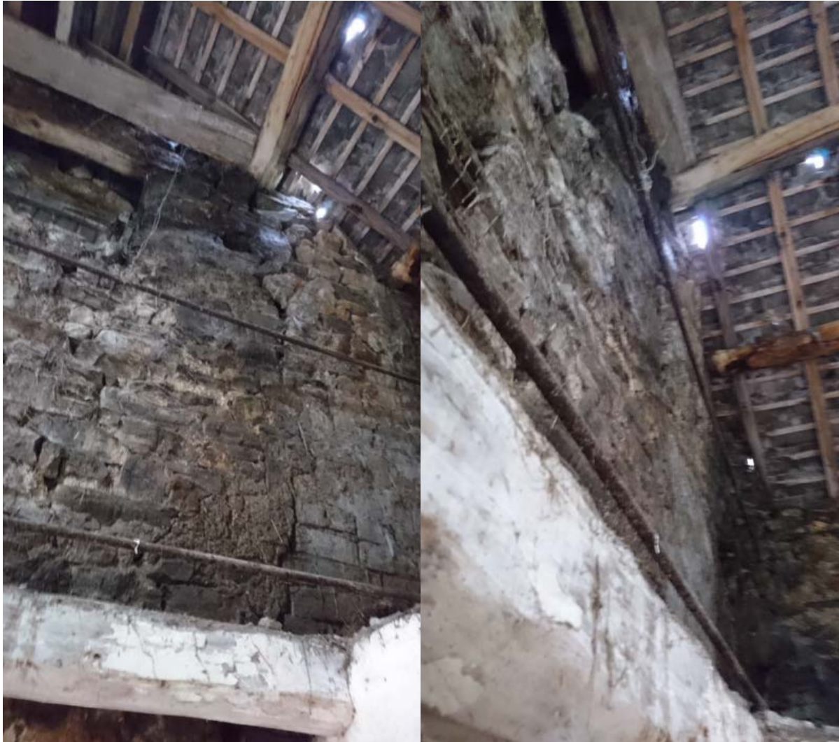
Figure 15: Steel tie rods connecting the two steel patten plates. Western gable beyond.
