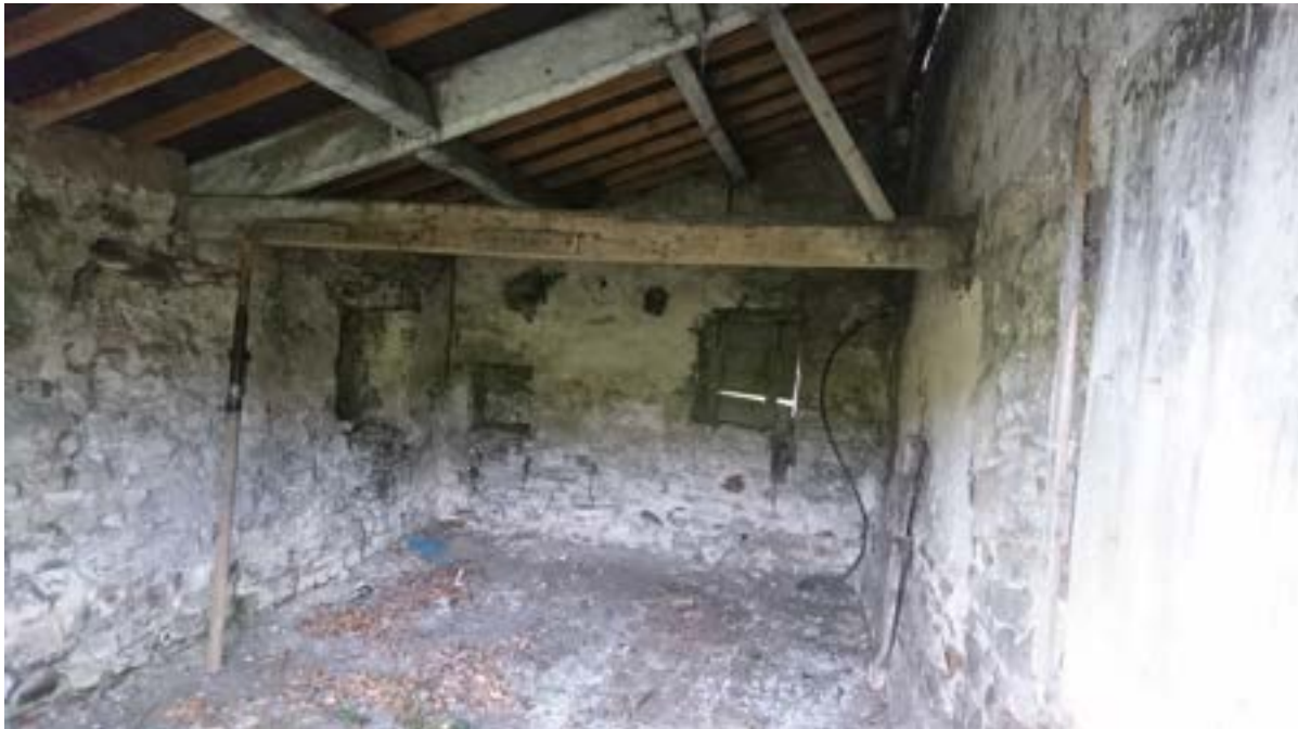
Figure 6: The roof from inside Extension 1, noting the prop to the truss at WP 11.
