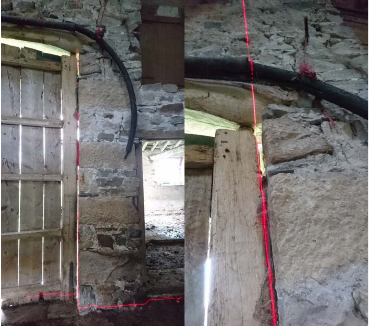
Figure 28: Image LEFT: A plumb laser trained on the edge of the bottom stone at the arched opening. Note the lack of buttressing masonry at the arch's bearing. Image RIGHT: apparent outward movement, likely due to the arch thrust.
