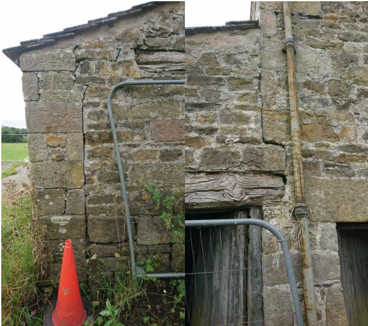
Figure 41: LEFT: Separation of the eastern elevation from the northern elevation. RIGHT: settlement of the masonry at the abutment with WP12, WP1 and WP2, believed to be related to the compression of the decaying timber lintel over time.
