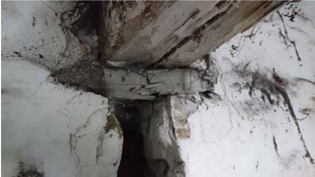
Figure 26: Fractured mudstone / slate lintel.
