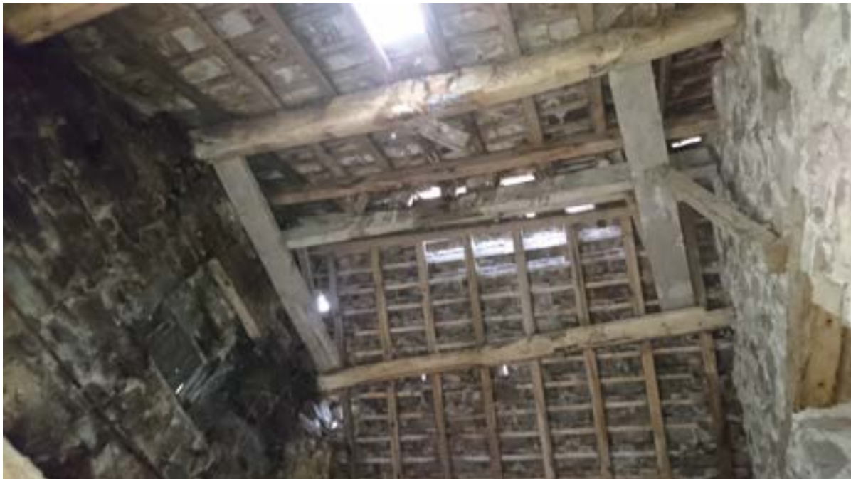
Figure 8: The new ridge, supported by various props and two boards spanning between the two upper purlins.
