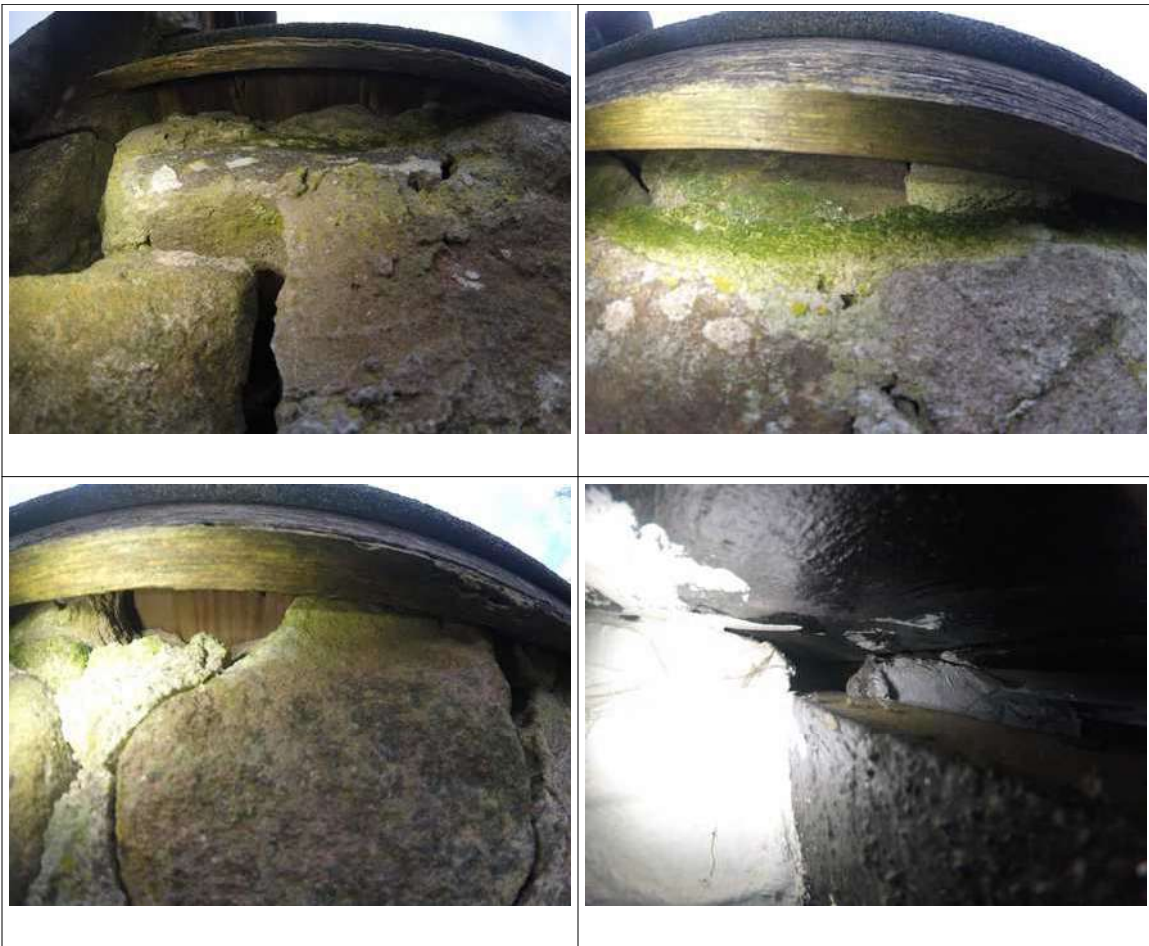
Gaps behind fascia boarding allowing access to wall tops on two storey extension
