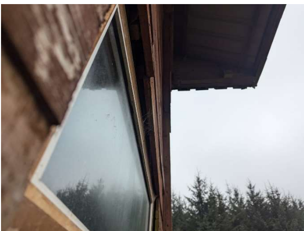
Photograph 8: B1 – PRF2: Gap under cladding over window on eastern aspect.
