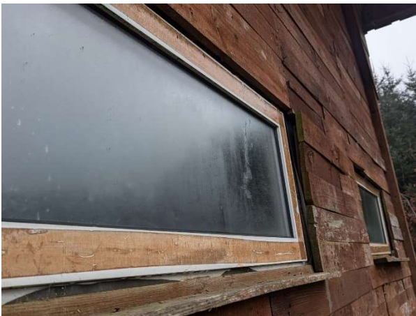
Photograph 7: B1 - PRF1: Gap behind cladding right of window on eastern aspect.
