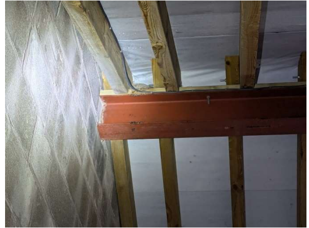
Photograph 15: Historic swallow nest on steel ridge beam in southern-most section of B2.
