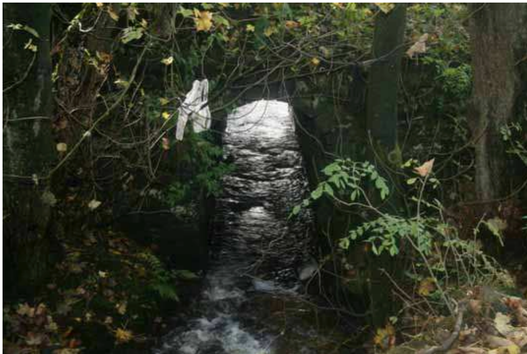
Plate 14: Cowley Brook within an artificial channel to the west of Cowley Brook cottage and culverted beneath Clitheroe Old Road
