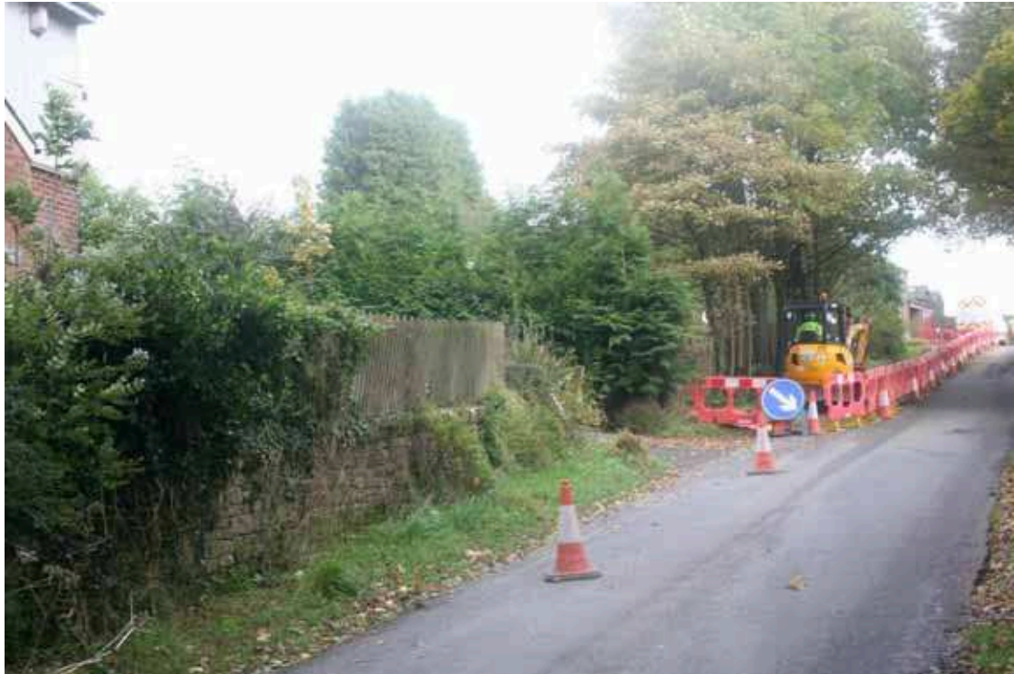
Plate 10: The line of the pipe trench along the northern side of Clitheroe Old Road, looking east
