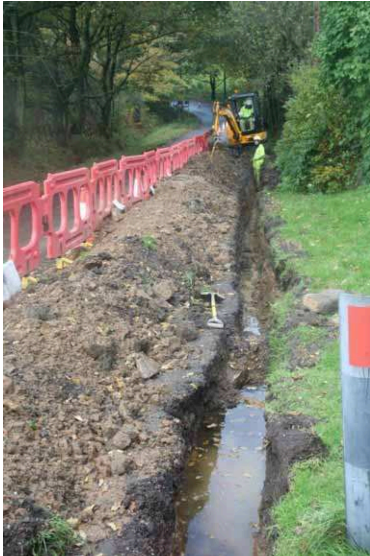
Plate 11: The narrow and inundated pipe trench at the northern side of Clitheroe Old Road, looking west
