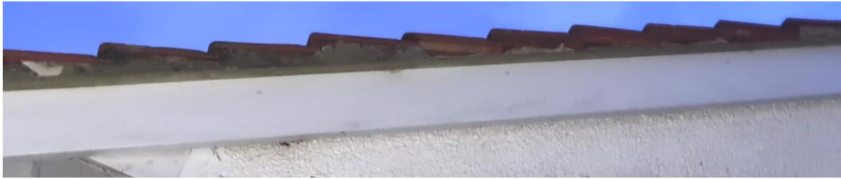
The verge pointing was slightly degraded, however there were no crevices deep enough to allow any bat ingress.
