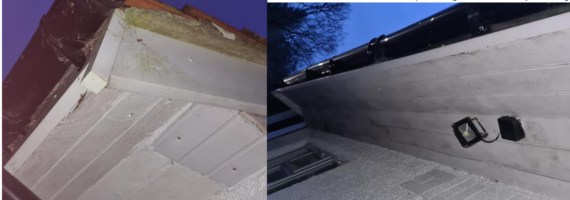
The overhang soffits are in very good condition and did not provide any access points
