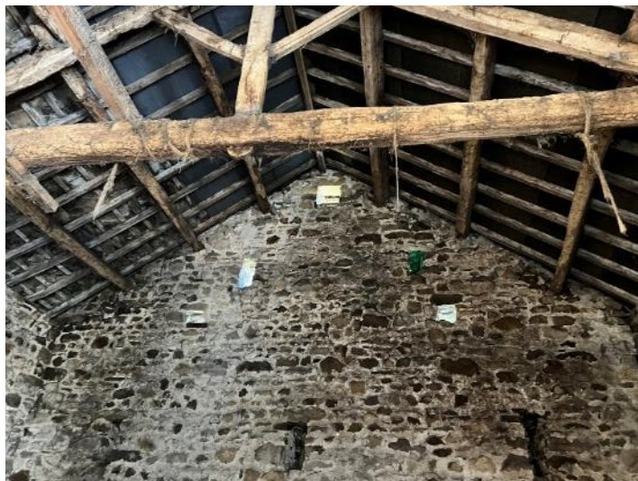
Figure 8: Showing the roof open to the underside of the tiles in places in B1.
