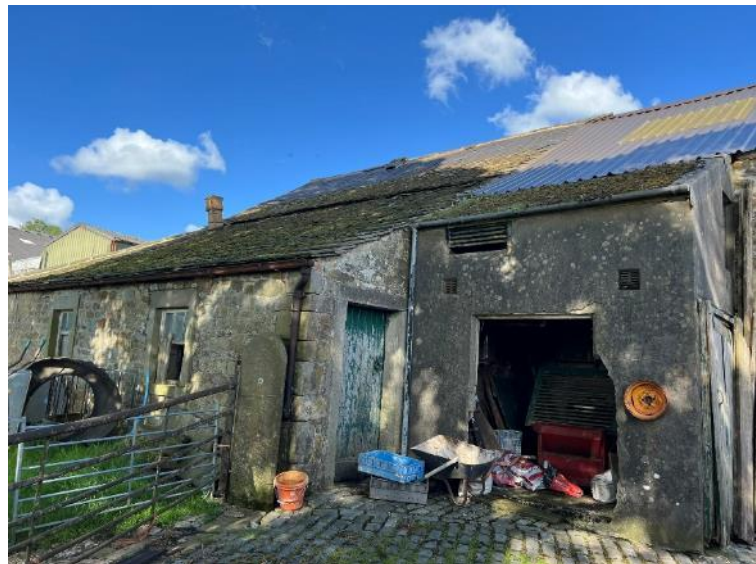
Figure 3: south end of the west elevation, showing part corrugated roof covering and single storey extension.
