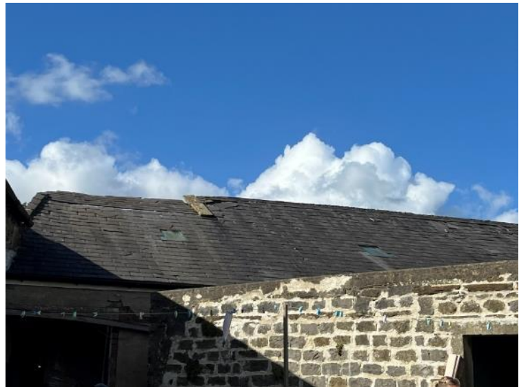
Figure 4: South facing roof pitch of B3, and front fascia of B2. Gaps can be seen in the roof materials at the ridge of B3.
