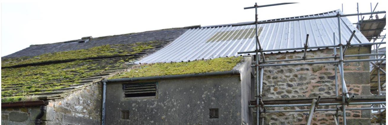
PL11: West Elevation Photo: showing stone slates to the left hand side of the barn roof and metal roof sheeting to right hand side. The rear rendered add on is proposed to be removed. The gutters and rainwater pipes are a mix of grey pvcu, black cast and missing sections of gutters.
