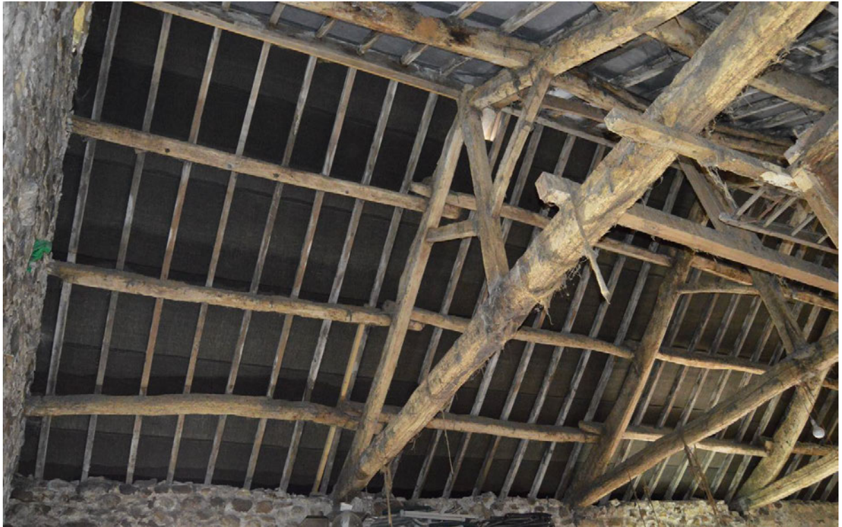
PL15: Photo showing underside of bituminous roofing felt, with battens and blue slate over. Original timber trusses and purlins.
