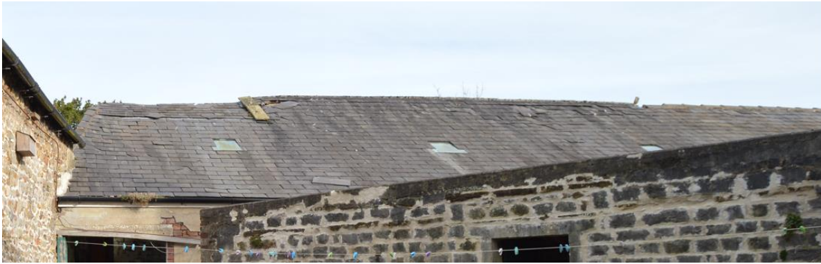
PL20: Photo showing mono pitch slate roof to outbuilding 2, a number of slate are missing and loose and a number of ridge tiles are missing.
