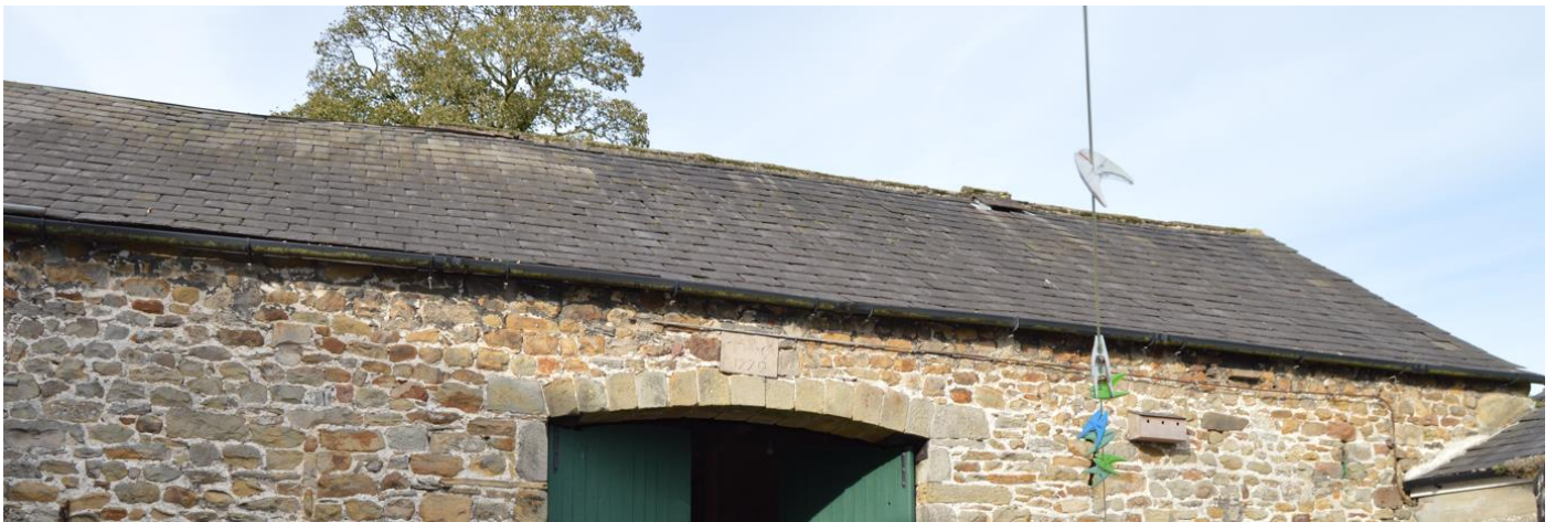
PL13: East Elevation Photo: Blue slate to roof slope, part sand and cement pointed ridge tile and part ridge flashing.
