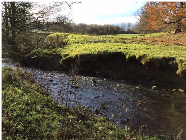
Photograph 7: Bank Erosion and Undercutting Upstream of Proposed Outfall Location
