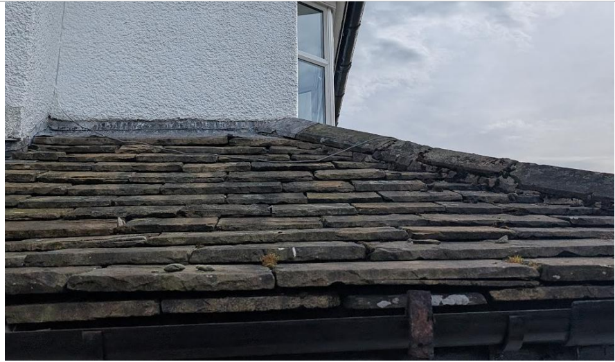
Photo 6 Example photo of gaps between roof slates.
