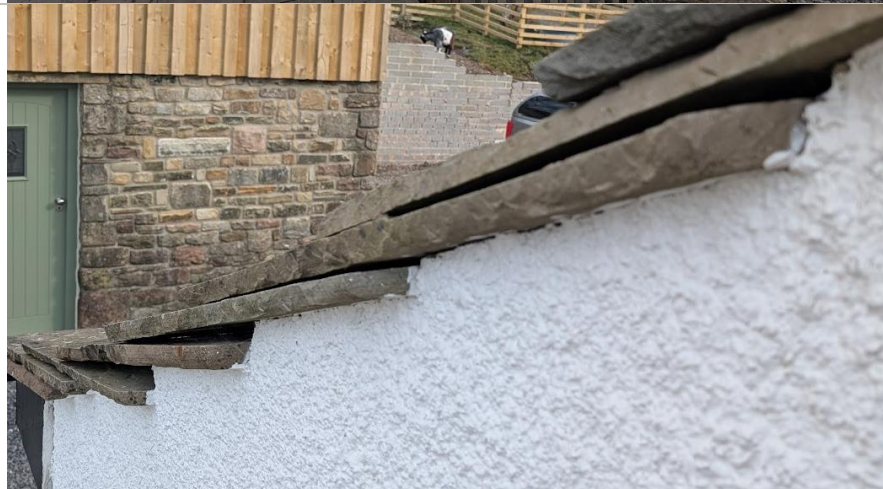
Photo 5 Crevices between slates on roof verge.
