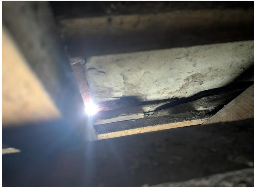
Photo 9 Daylight gap in roof.
