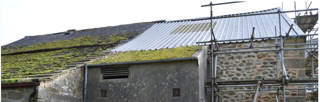
PL11: West Elevation Photo: showing stone slates to the left hand side of the barn roof and metal roof sheeting to right hand side. The rear rendered add on is proposed to be removed. The gutters and rainwater pipes are a mix of grey pvcu, black cast and missing sections of gutters.
