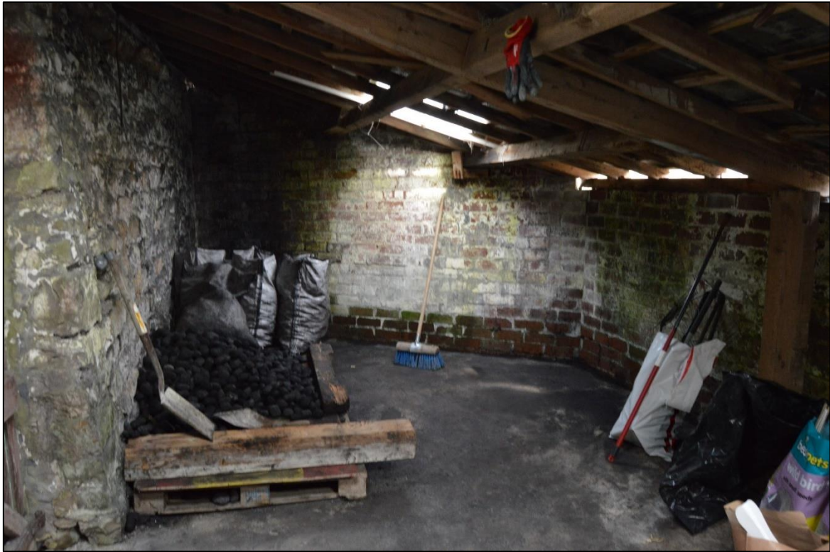
PL19: Photo showing roof structure to Outbuilding 1, comprising of sawn timber purlins and rafters
