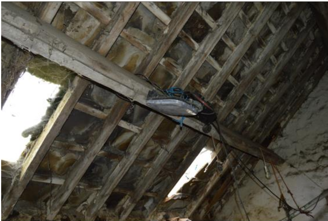
PL16: Photo showing underside of shippon roof, comprising of purlins and rafters with stone slates / flags over.
