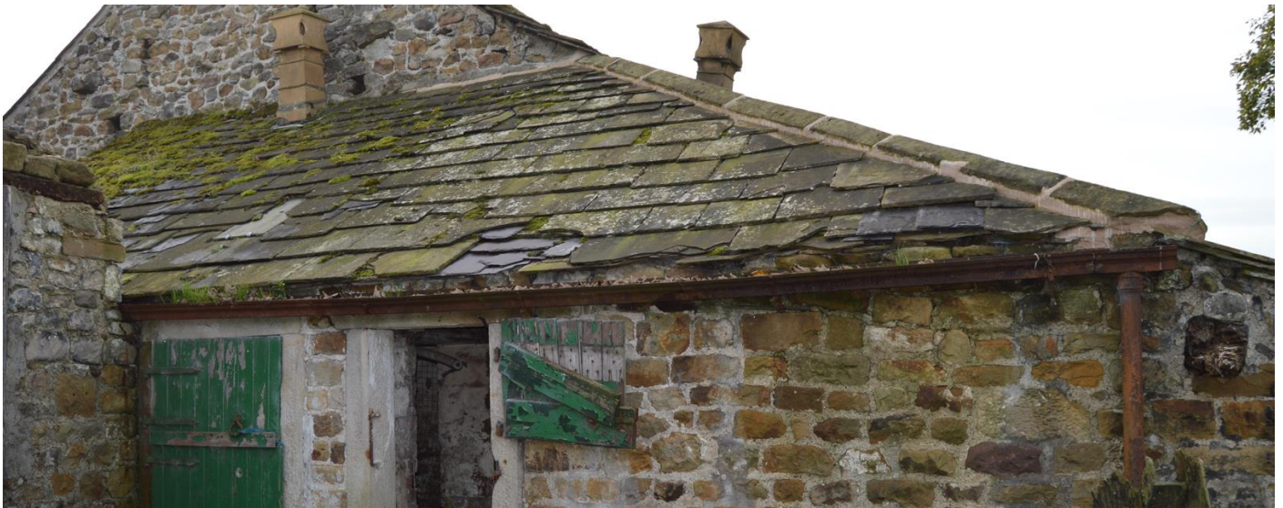
PL12: North Elevation Photo: showing stone slates and sand and cement pointed ridge tiles. A number of the original stone slates have broken and have been replaced and patched with blue slate. Rusted cast gutter and rainwater pipe.
