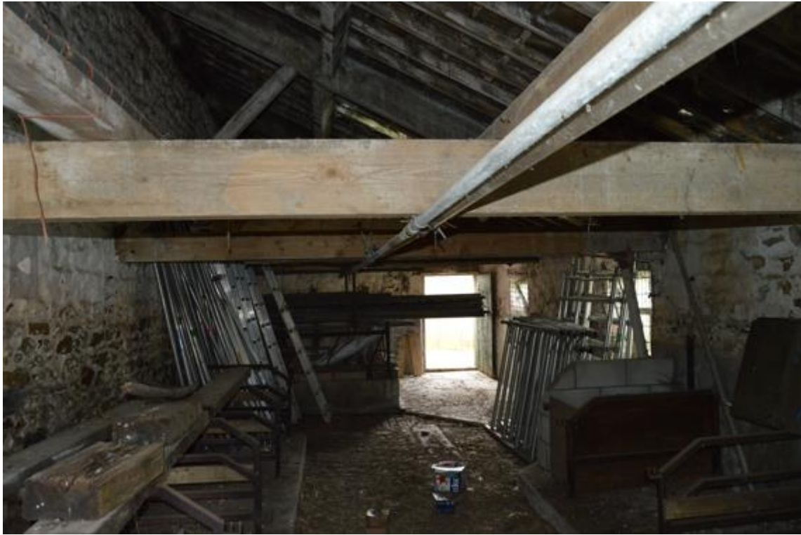
PL17: Photo showing underside of shippon roof, comprising of sawn timber half trusses purlins and rafters with stone slates / flags over.
