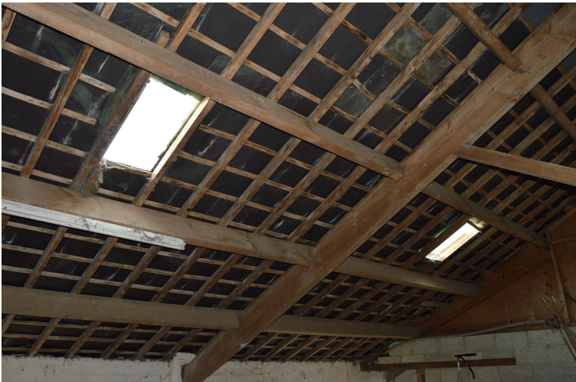
PL19: Photo showing underside of outbuilding 2 roof, comprising of sawn timber half trusses, purlins, rafters battens with natural slate over
