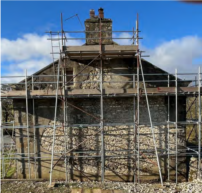
East gable. Note remains of 20 th century cement render.
