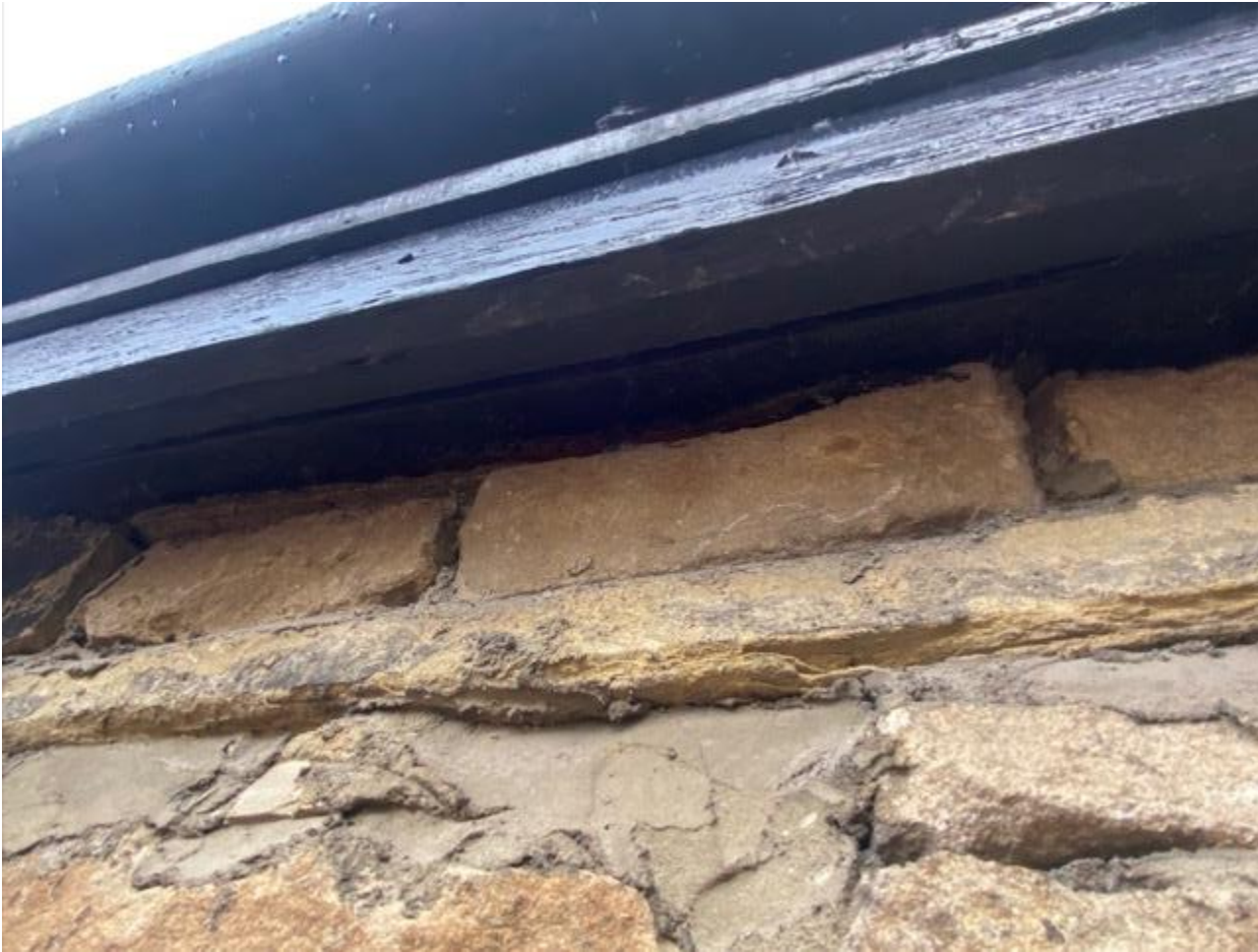
Photo 5: Close up of soffit boxes, which are well sealed against the brickwork.
