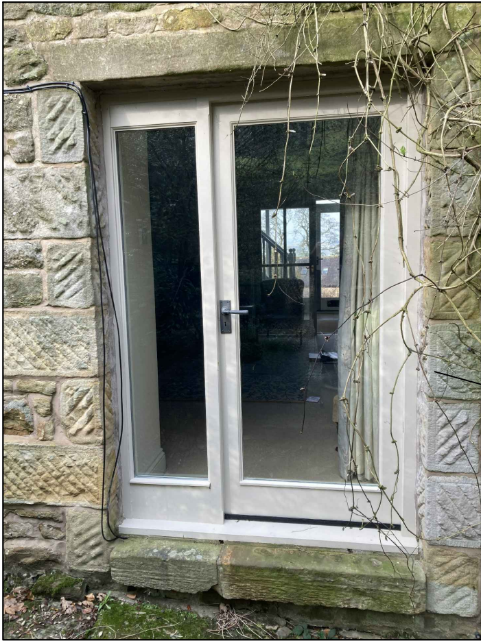
Photograph showing DF2
