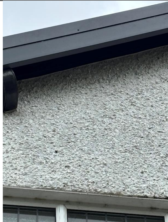
Photograph 2: View of tightly sealed eaves.
