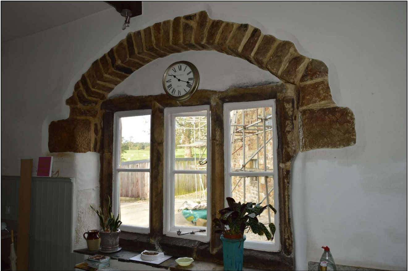
PL10: View of the extant window to the rear north wall of the ground floor utility room.
