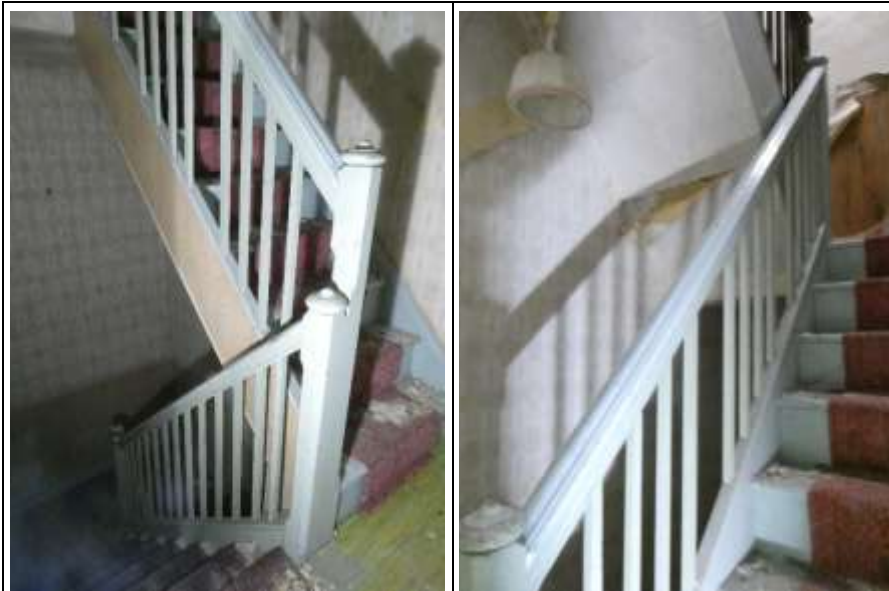
Slender Square Balusters, Some Missing
