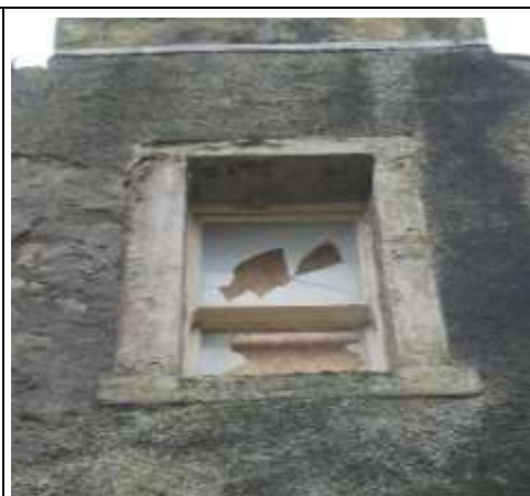
Timber Frame, Broken Pane
