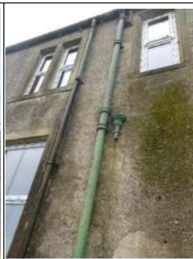
Plastic and Painted Cast Iron Downpipes
