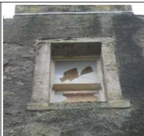
Timber Frame, Broken Pane
