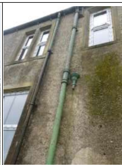
Plastic and Painted Cast Iron Downpipes
