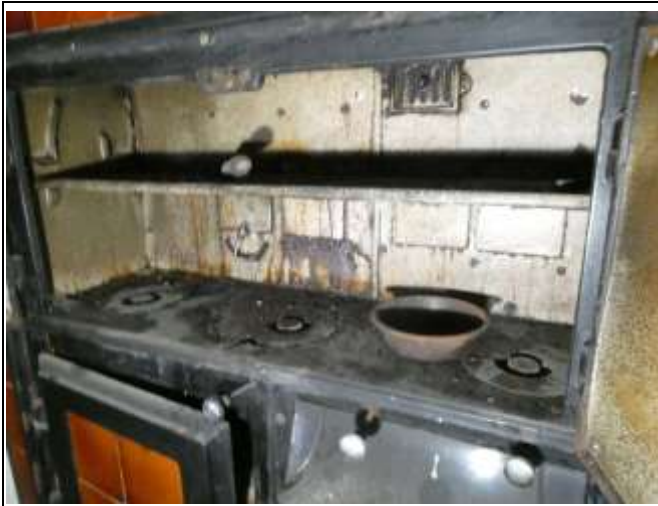
Interior of the Oven
