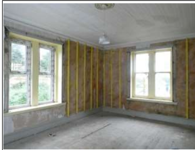
Corner of Room, Dual Aspect Replacement Window to the North and Timber Frame Window to the West
