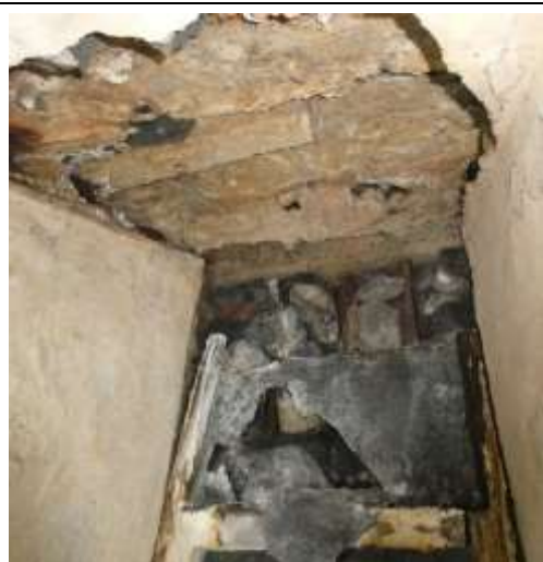
Damage to the Ceiling
