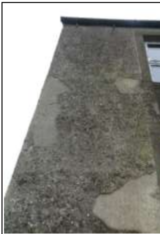
Damage to the Render at the Southwest Corner
