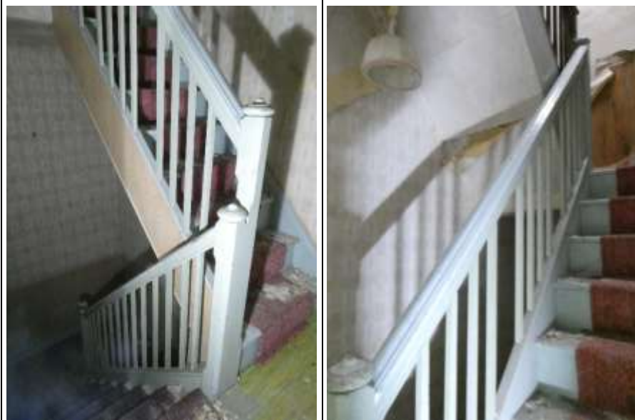
Slender Square Balusters, Some Missing
