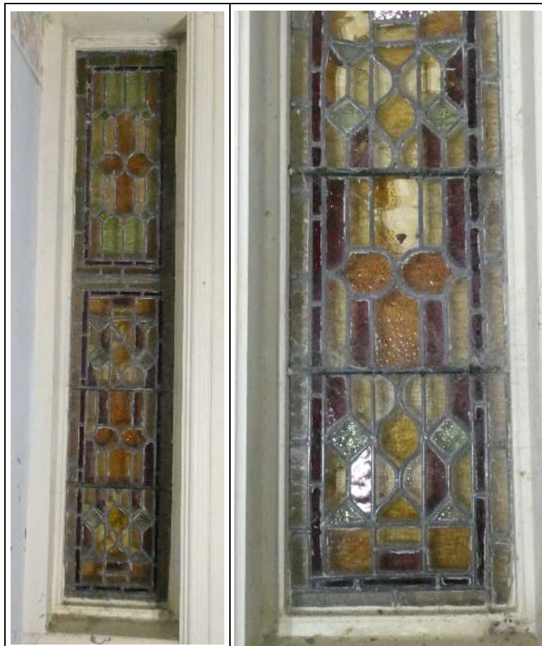
Damage to the Glazing at the Side Panels
