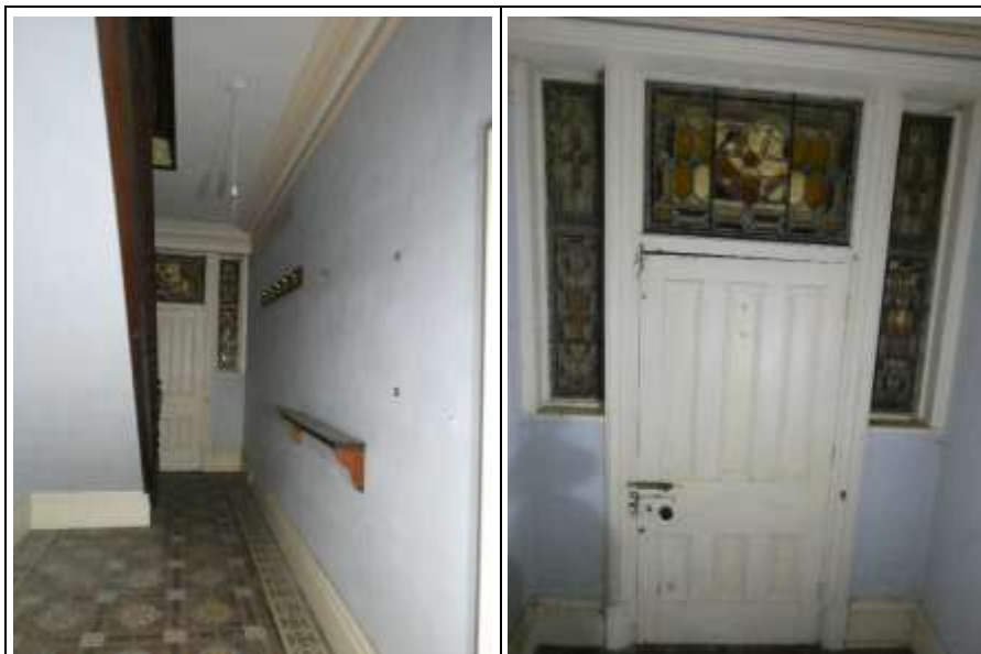
Looking West Towards Timber Door and Stain Glass Surround at Main Entrance
