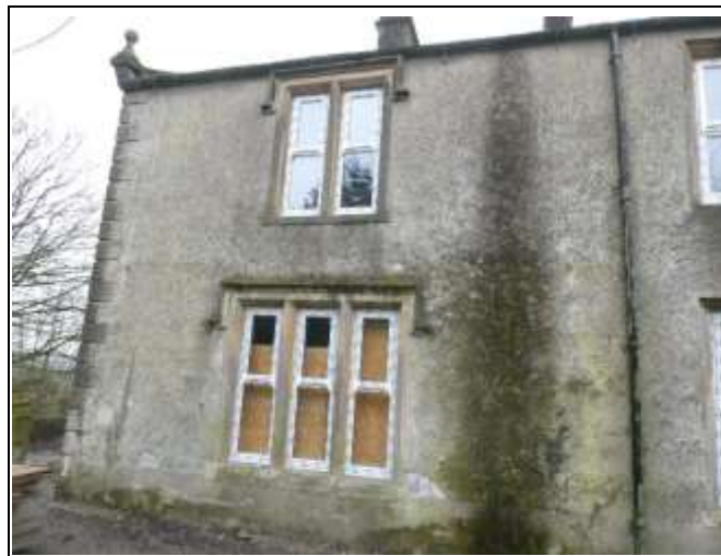
West Side of Elevation, Water Damage to the Render
