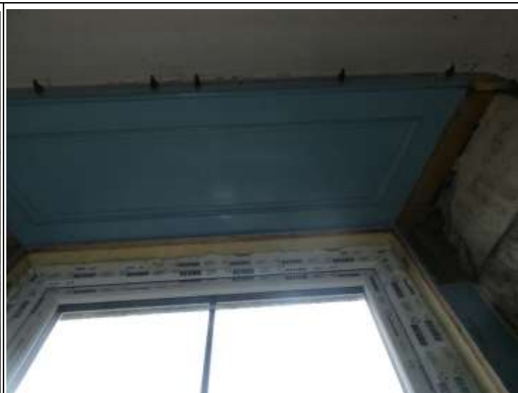
Remnant of Timber Shutters
