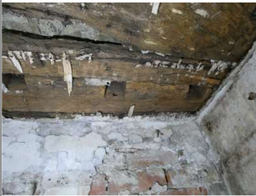
Ceiling at the Former Built-in Cupboard
