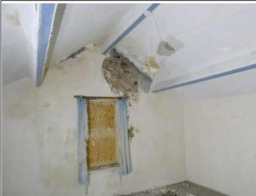
Boarded-up Window at the East Elevation
