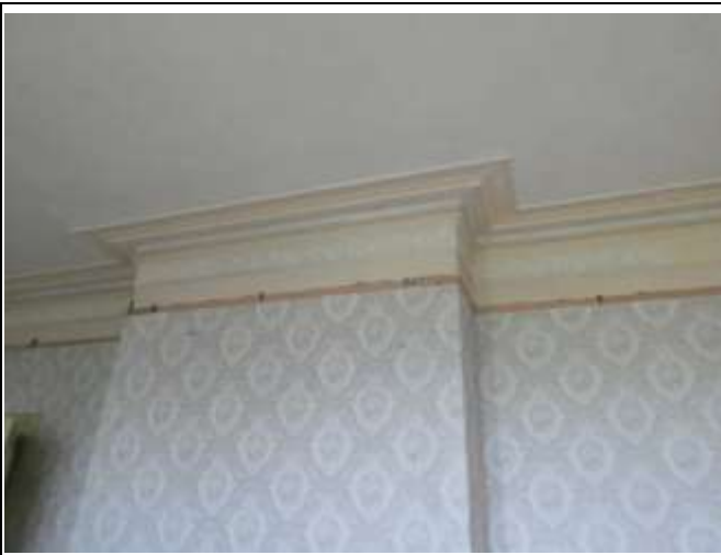
Plaster Cornice, Missing Picture Rail
