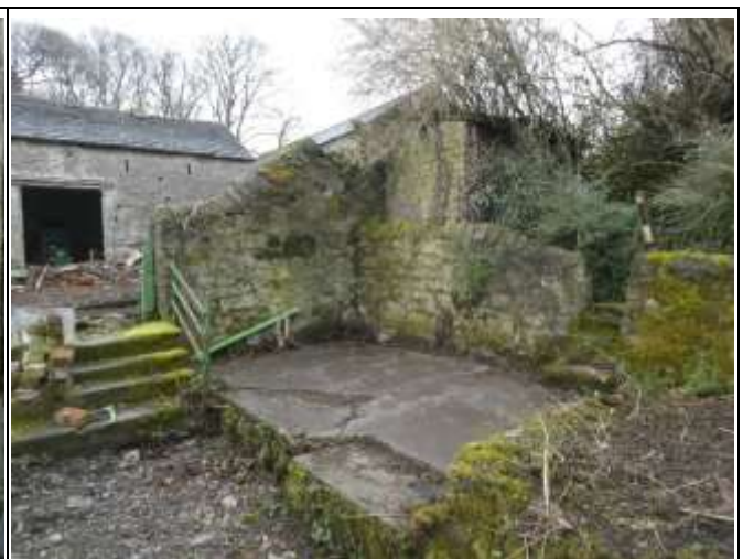
Remnants of Foundations and Stone Steps to the Farmyard, Listed Barn Behind
