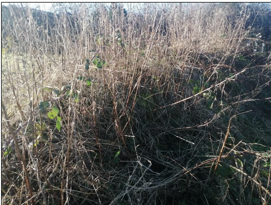
Plate 18 – Overgrown old stone wall (TN4)
