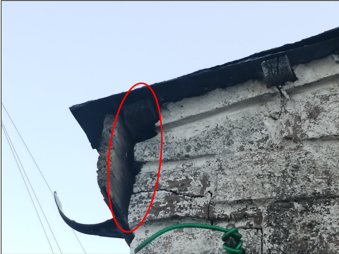
Plate 3 – PRF in the form of a gap behind the timber fascia board on northern elevation
