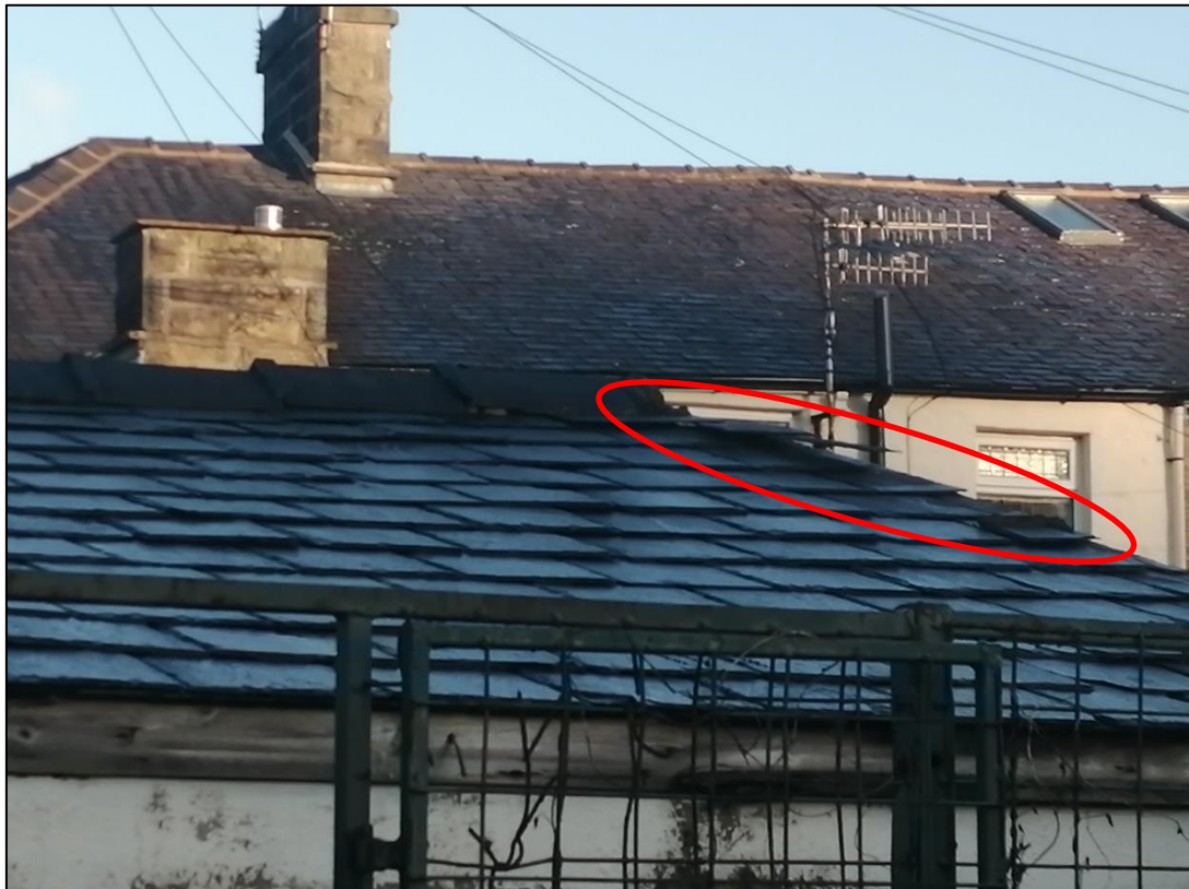
Plate 2 – PRFs in the form of lifted slate tiles on eastern verge
