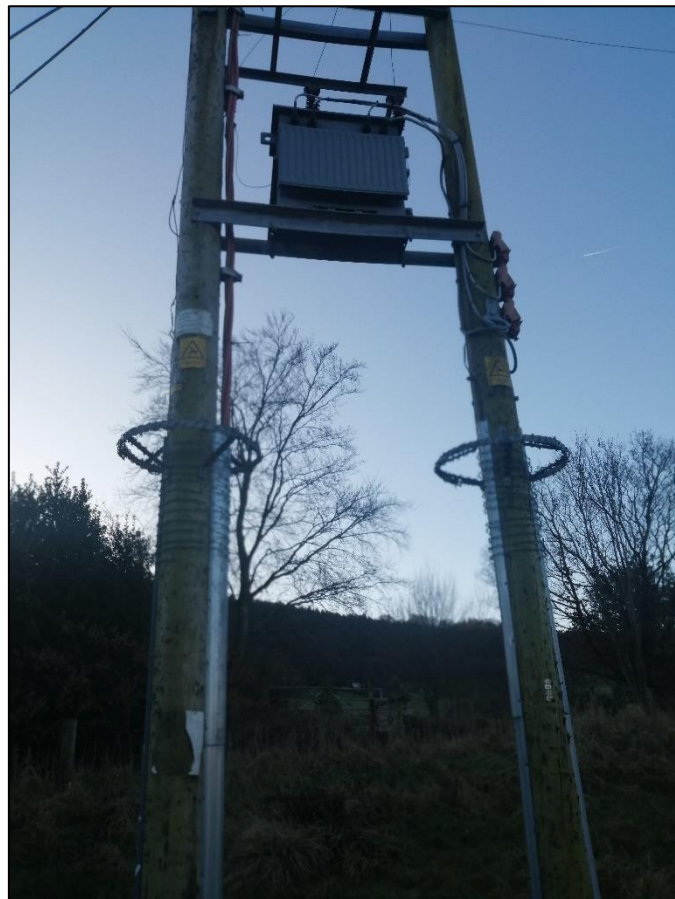
Plate 8 – Power line / transformer located onsite
