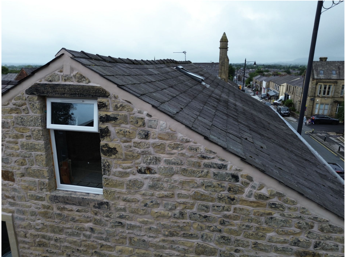
3 – Cement at the gable end verges is in good condition with no viable gaps.
