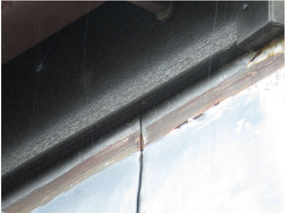
5 – Where present, fascia, and lead flashing are fitted tightly with no suitable gaps.
