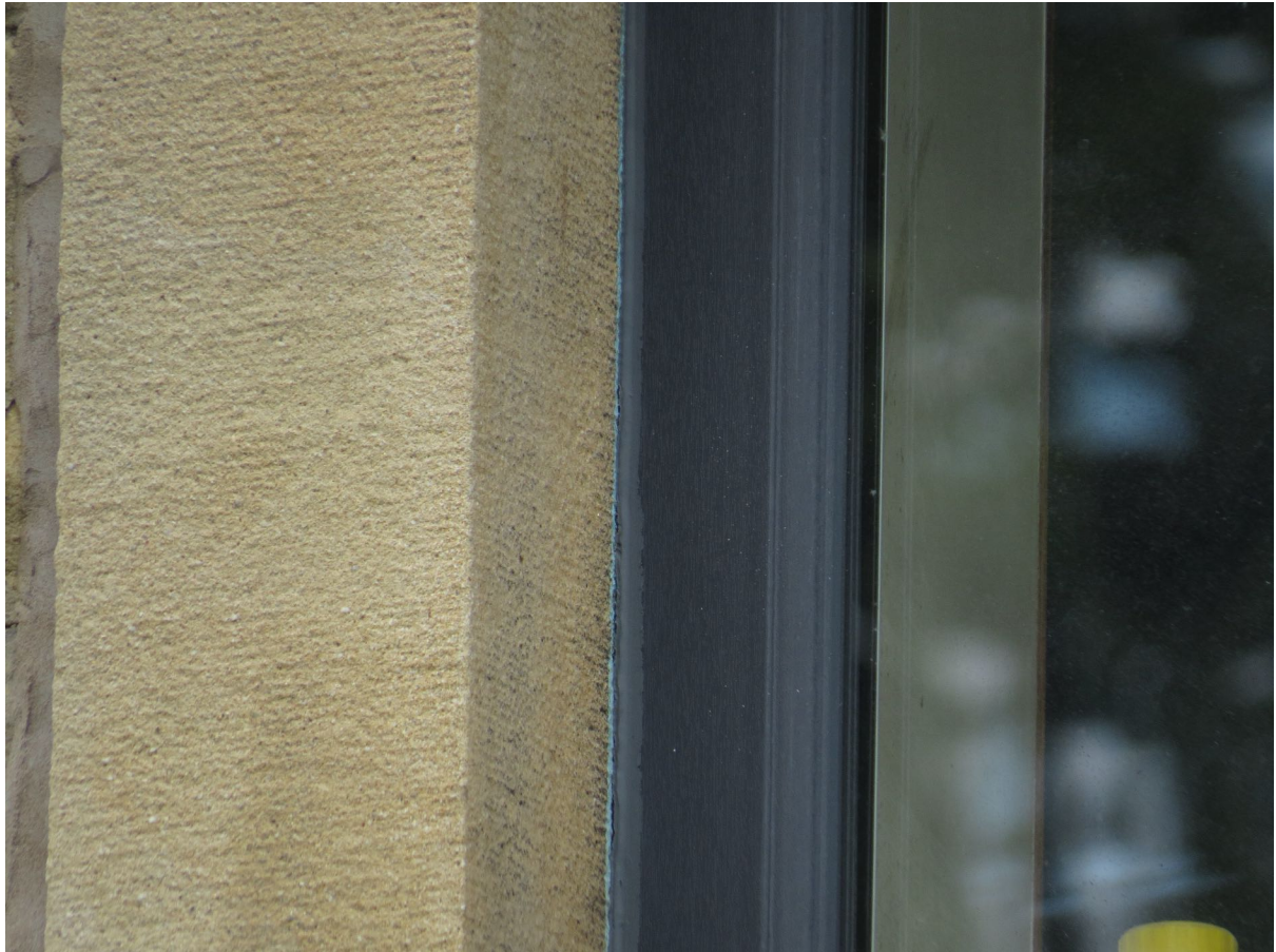
7 – Window and door frames are tightly sealed into stonework with no suitable gaps.
