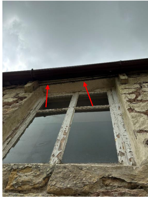
Photograph 6: Areas where the fascia board has separated from the wall plate on southern aspect.
