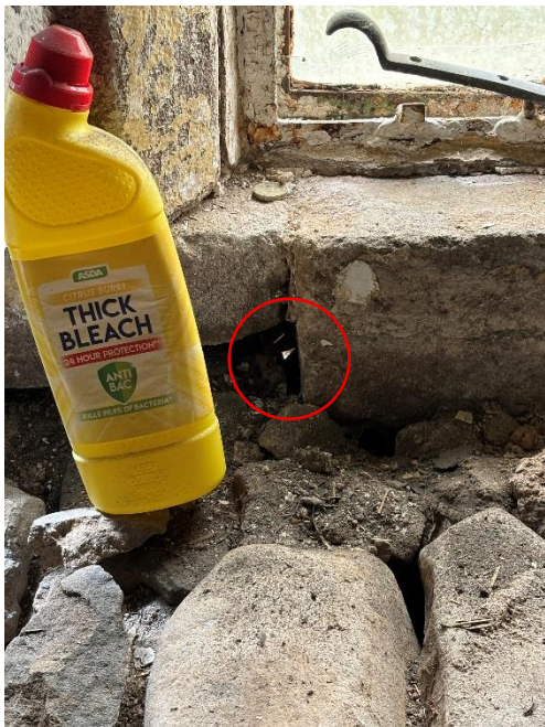
Photograph 7: Light shining through from outside between stone bricks.
