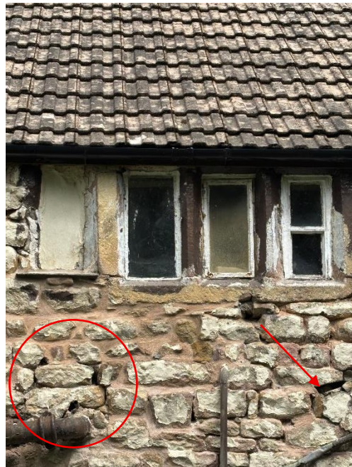
Photograph 4: Cavities between stone bricks on southern aspect.
