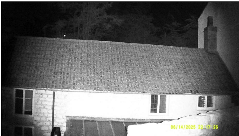
Figure 3-1: NVA screenshot of eastern aspect of the building at darkest point of Survey 1.
