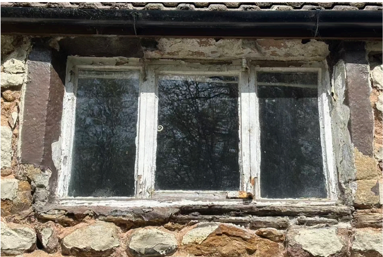
Figure 8: Missing mullions and cill to rear.
