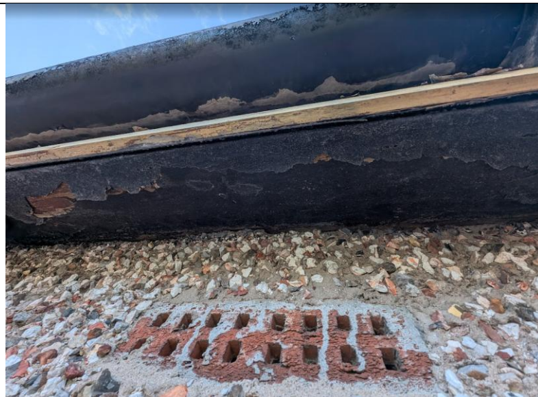
Photo 4. View of sealed soffit and slight gap underneath fascia (no suitability).
