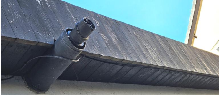
Boarded fascia to garage
