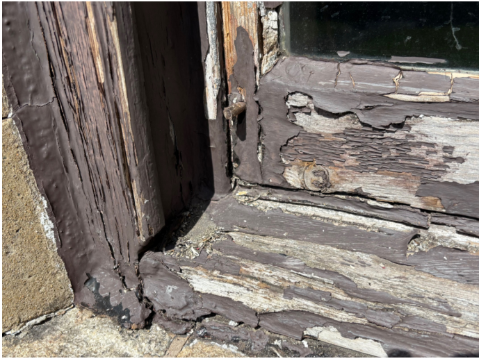
Photograph 1. Rot at the junction between sash box and sill.
