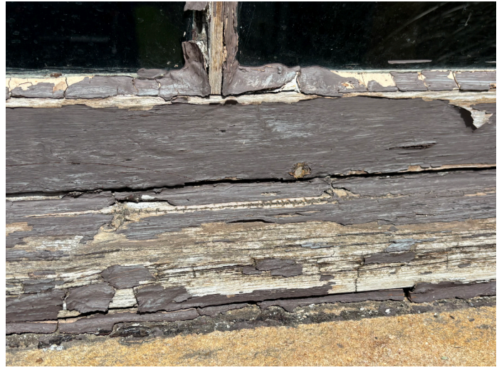
Photograph 2. Loose putty and rot in sill.
