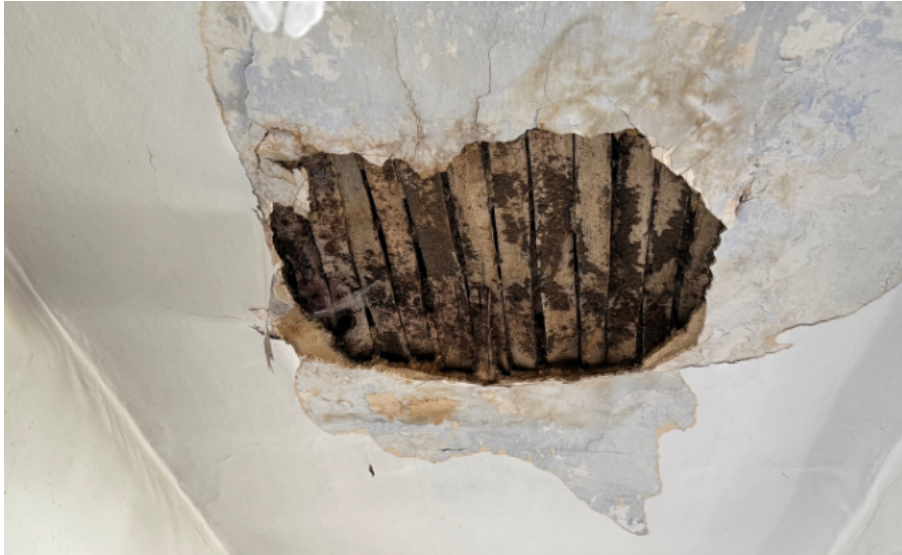
Photograph 25. A partly collapsed ceiling in the eastern ground floor room.
