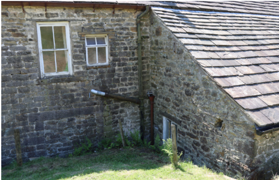
Photograph 11. The north side of the main house and east side of the lean-to.
