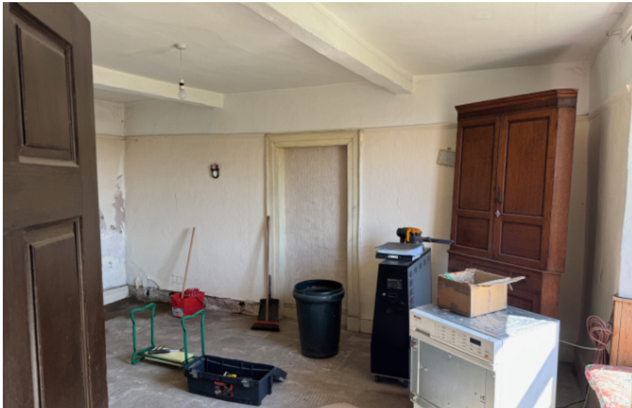
Photograph 23. The eastern ground floor room, with an architrave to a blocked doorway.
