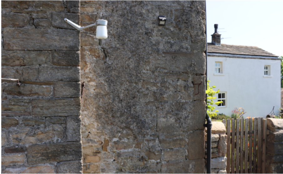
Photograph 9. The remains of lime roughcast on the west gable wall.
