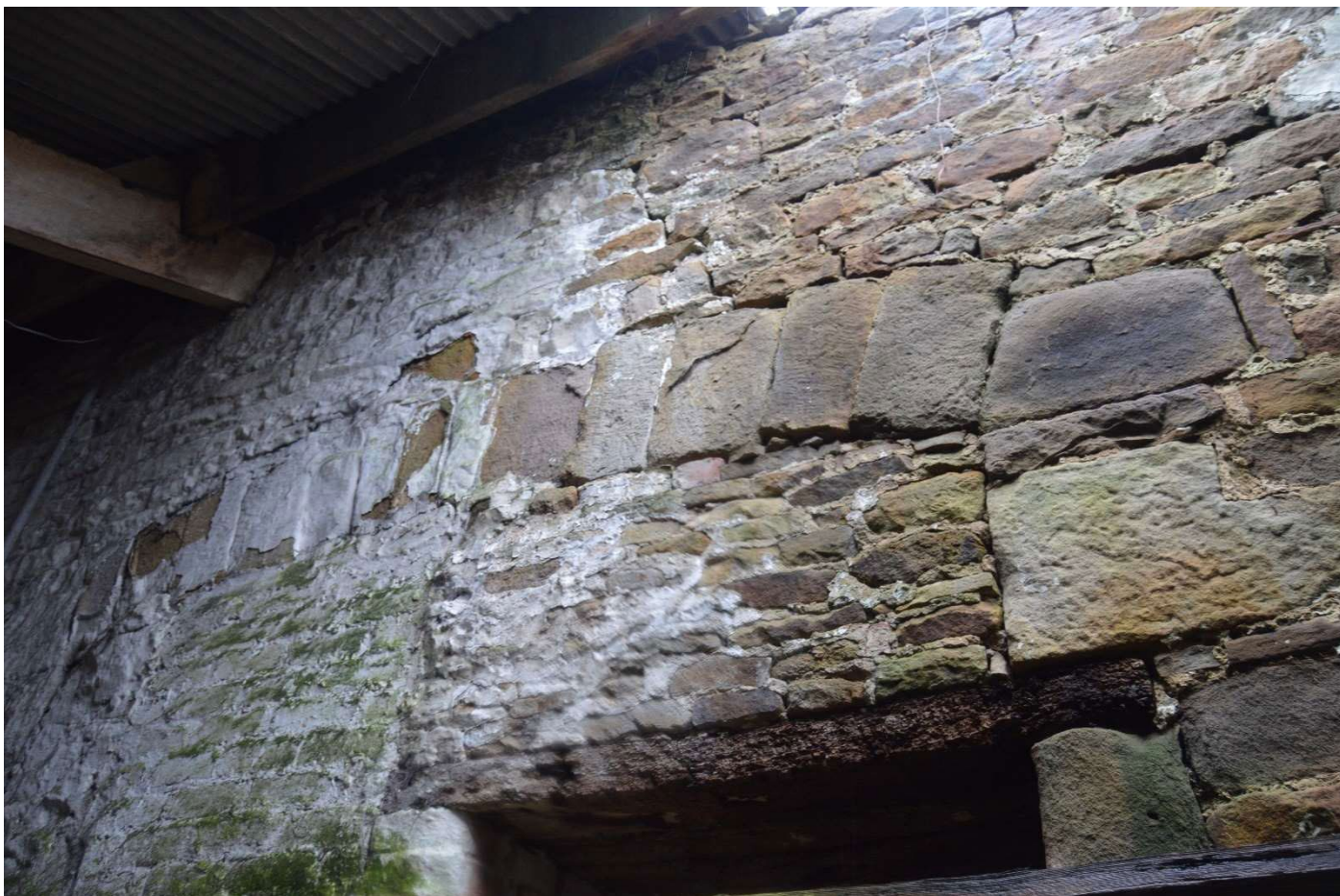
Fig 12 View of stone voussoirs to the blocked up opening from within the south shippon
