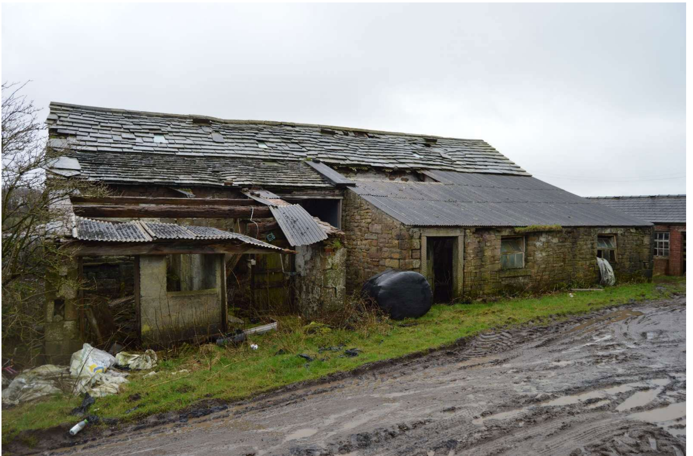
Fig 3 View of the front elevation (north) of the barn from the north east
