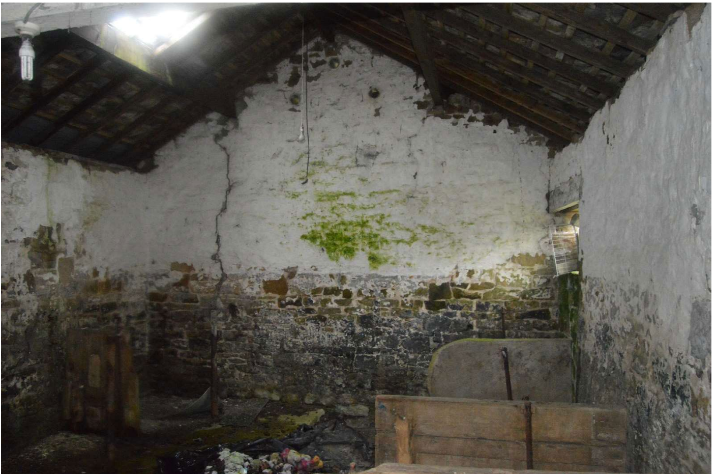
Fig 16 Internal view (north) of the stone outbuilding
