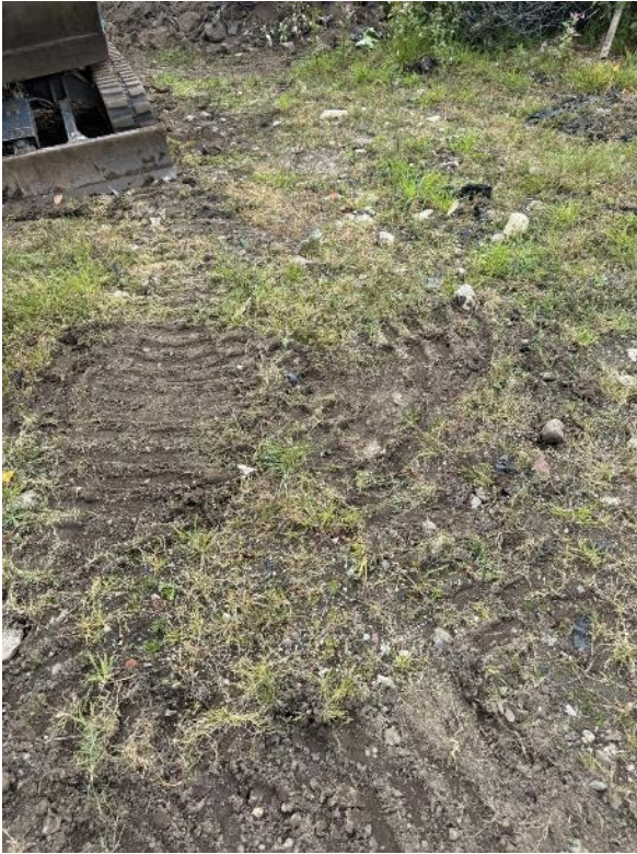
Photograph 3: Example of substrate where the machinery has tracked and exposing the u1c artificial substrate. The development area will be confined to the already developed farm yard.
