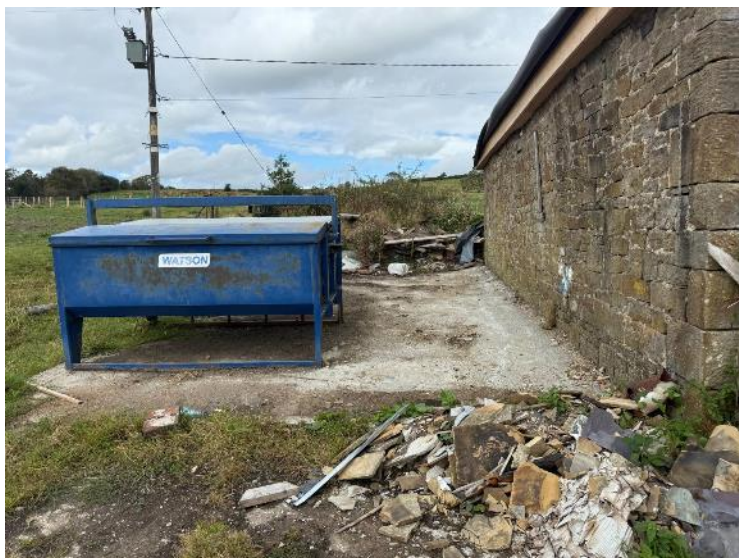
Photograph 2: Areas of u1b6 (concrete) and u1c artificial substrate around existing farm buildings. Localised areas of grass and forb coverage establishing on u1c substrate but vegetation coverage is ~20% of the overall u1c area.
