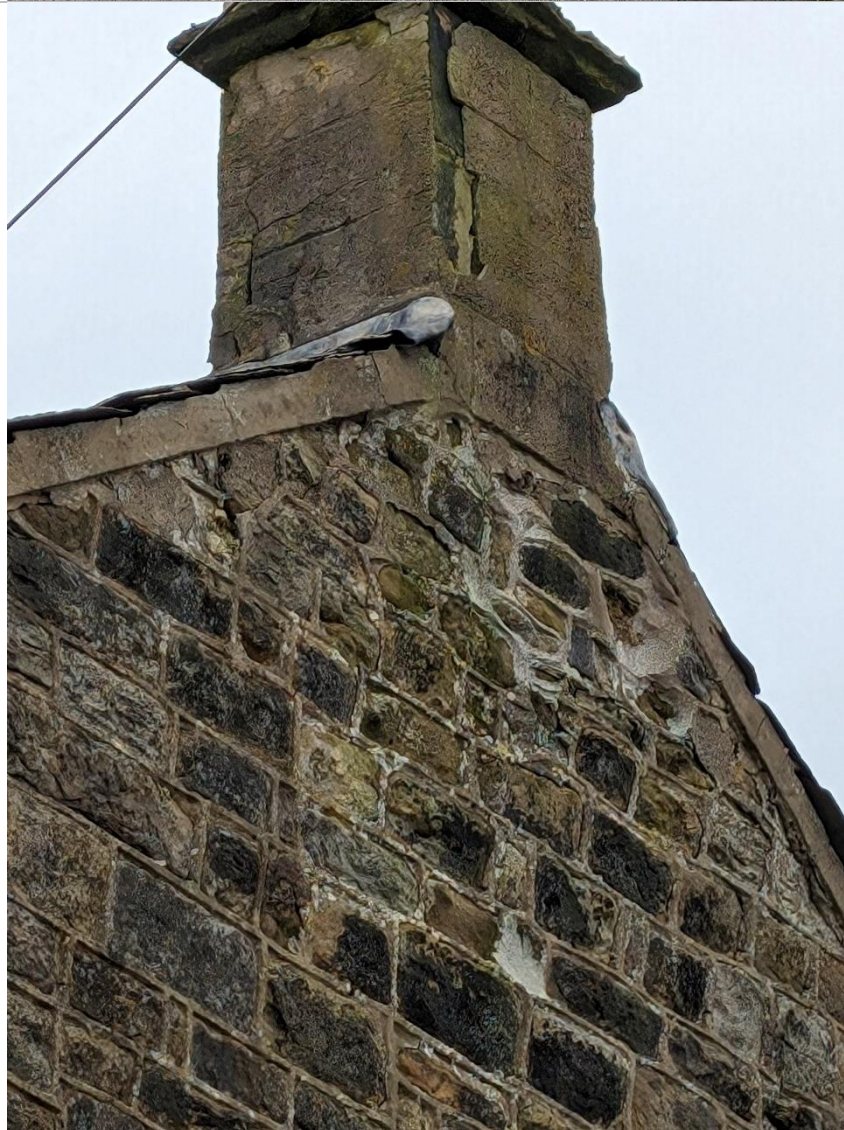
Photo 6. Gap under lead flashing on east gable.
