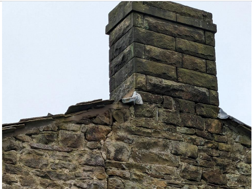
Photo 3 Gap in stonework, gaps under verge roof tiles and gaps under lead flashing.
